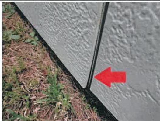
Damaged Siding. Right side of the home
