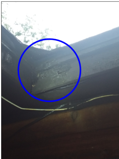
-Seal gaps and holes in trim to help prevent water penetration or rodent intrusion. Mainly at - left side
