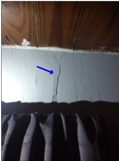
-Settlement cracks were noted in the drywall. Mainly at - right front bedroom
