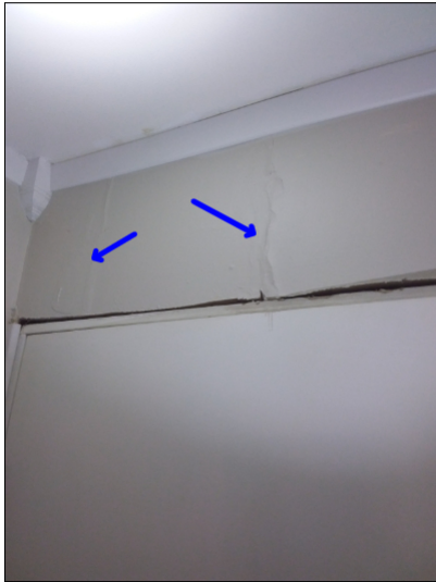
-Settlement cracks were noted in the drywall. Mainly at - right middle bedroom
