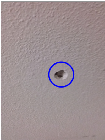
-There is damage to the drywall, recommend repairs as needed. Mainly at - right middle bedroom
