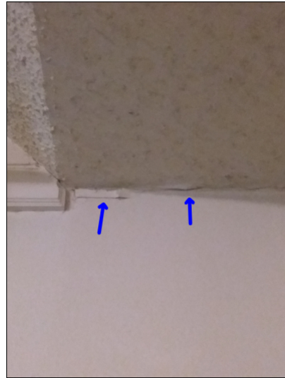
-Settlement cracks were noted at the tape joint in the drywall. Mainly at - master bedroom
