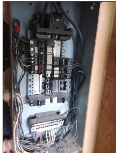
Overview of main electrical panel
