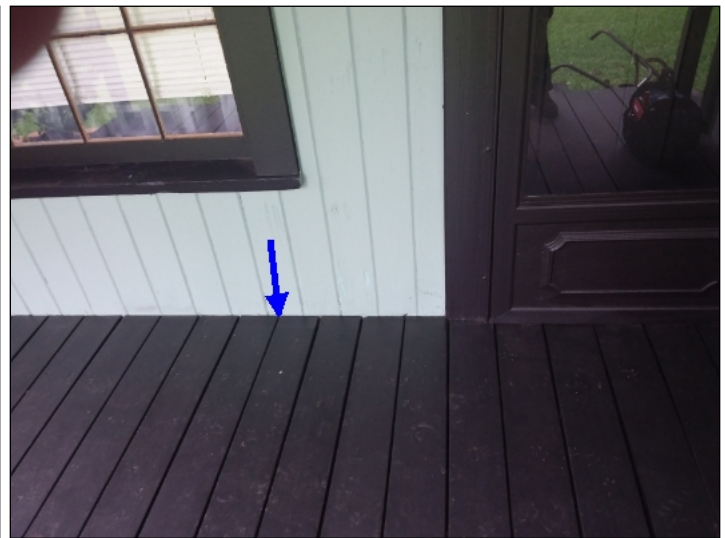
-The deck is installed against the house. Recommend all decks be separated from the structure to help prevent conducive conditions for wood destroying insects.
