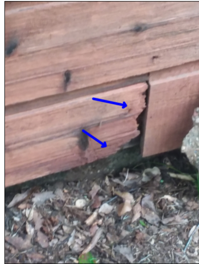
-Deterioration was noted at the siding, recommend replacing all deteriorated siding to help prevent further deterioration and water penetration. Unable to determine the condition of the underlying materials. Mainly at - left side
