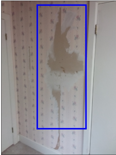
-Torn wall paper was noted. Mainly at - master bath
