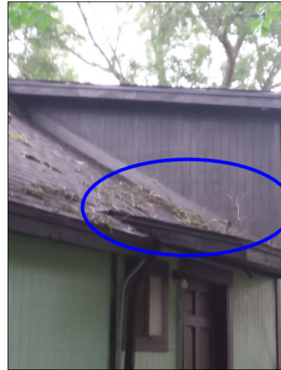
-Debris were noted on the roof which can cause water to back up on the roof and allow water to penetrate through the roofing materials, recommend removing debris from roof. Unable to fully inspect roof covering as debris limit the visibility of the roof surface.
