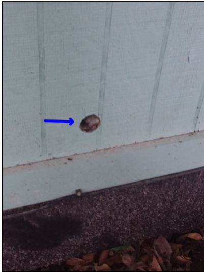
-Seal gaps and holes in siding to help prevent water penetration. Mainly at - right side
