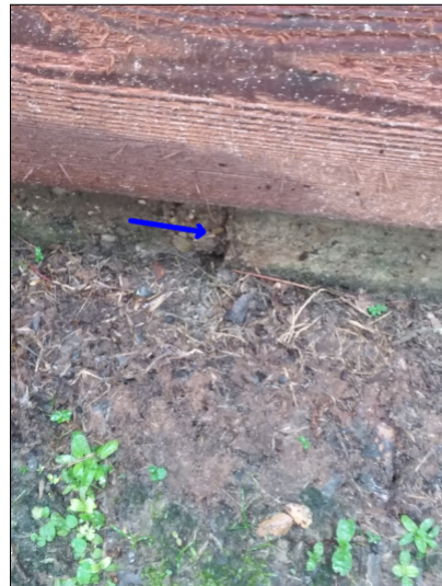
-Expansion cracks were noted in the slab. Mainly at - left side
