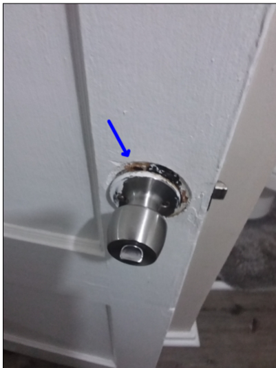
-The door knob is loose. Mainly at - front right bath
