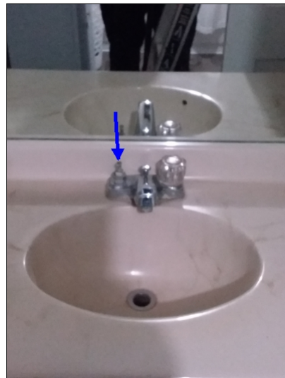
-There is a missing/broken shut off handle. Mainly at - right side bath
