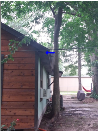
-All trees should be located no closer than 15' from structure to help prevent foundation movement. You may want to keep larger trees trimmed to help slow further root growth and future foundation movement as removing older trees may cause voids under the slab from dyeing root systems.
