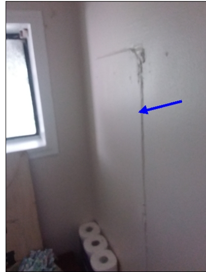
-Previous repairs were noted in the wall. Mainly at - right side bath
