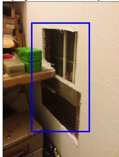
-There is damage to the drywall, recommend repairs as needed. Mainly at - master bath
