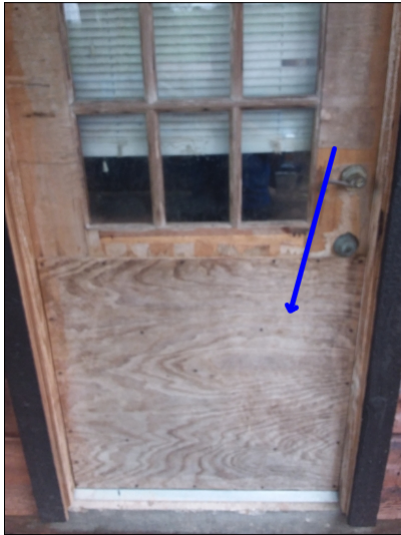
-Deterioration was noted mainly along the door, recommend repair or replacement to help prevent water penetration. Unable to determine the condition of the underlying materials. Mainly at - left side
