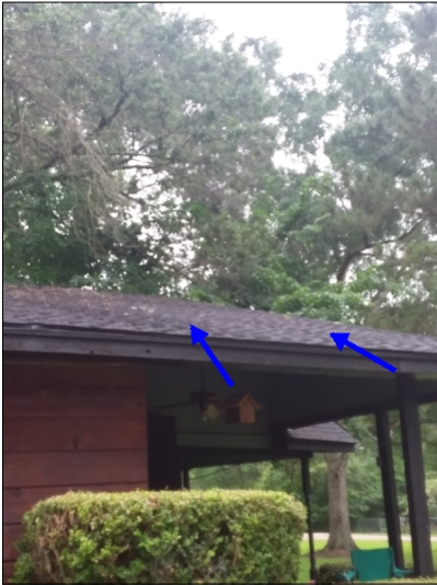
-The decking is buckling on the roof, this is often caused by an improper gap for expansion of the decking materials, recommend consulting a roofing contractor for evaluation and repairs as needed.
