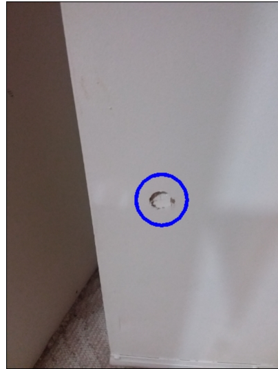
-Deterioration was noted mainly along the door, recommend repair or replacement to help prevent water penetration. Unable to determine the condition of the underlying materials. Mainly at - right middle bedroom
