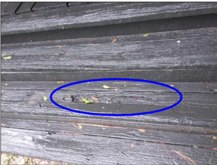
-The deck is showing signs of deterioration, recommend repair or replacement.
