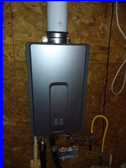
tankless water heater attic
