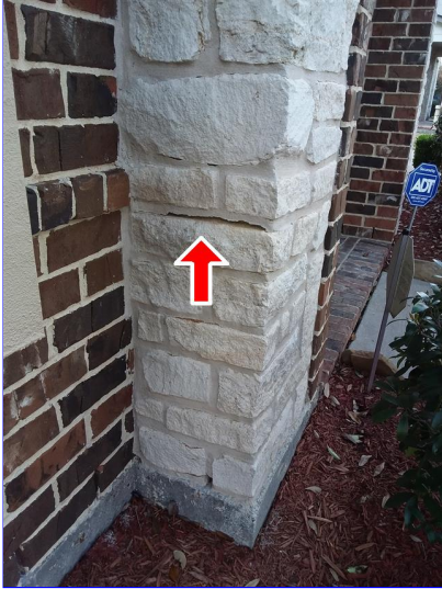
E. Item 11(Picture) entry left
