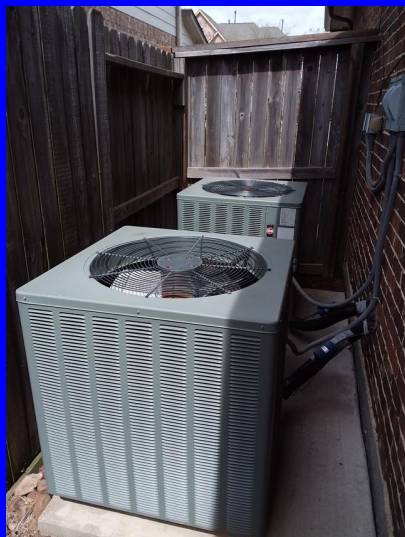
ac units exterior right
