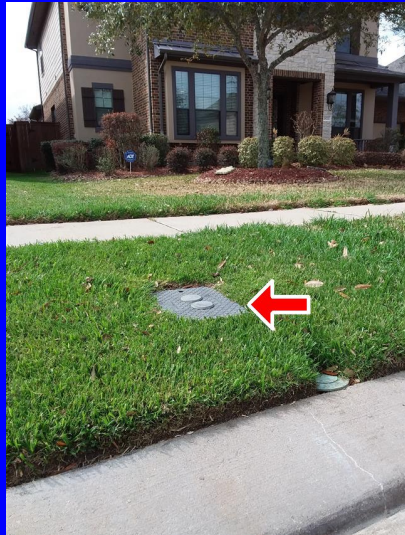
water meter front left
