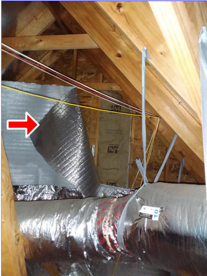
D. Item 5(Picture) front right
