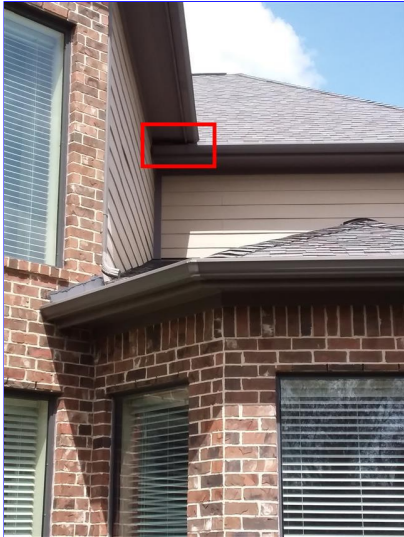
L. Item 5(Picture) rear left
