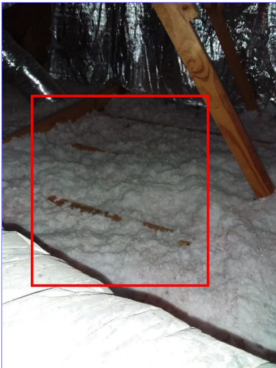
D. Item 6(Picture) front right
