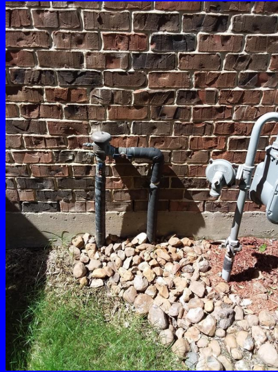
sprinkler shut off front left
