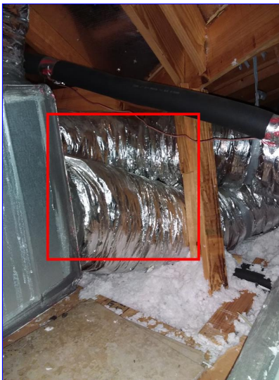
C. Item 2(Picture) rear
