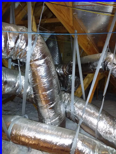
insulated ducts attic
