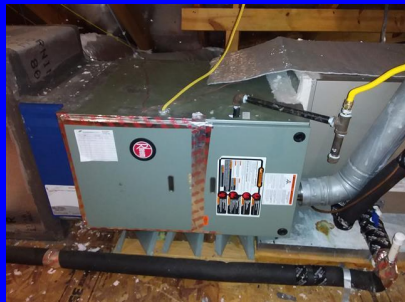
gas furnace attic
