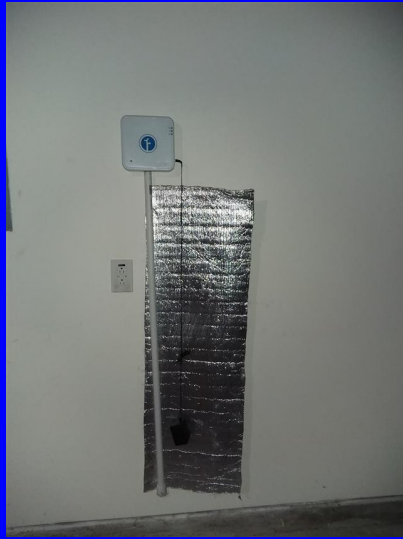
sprinkler control system garage
