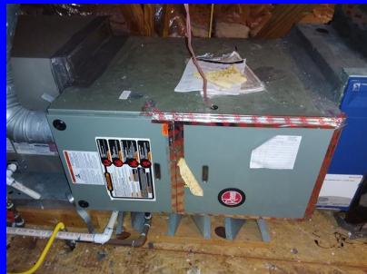
gas furnace attic
