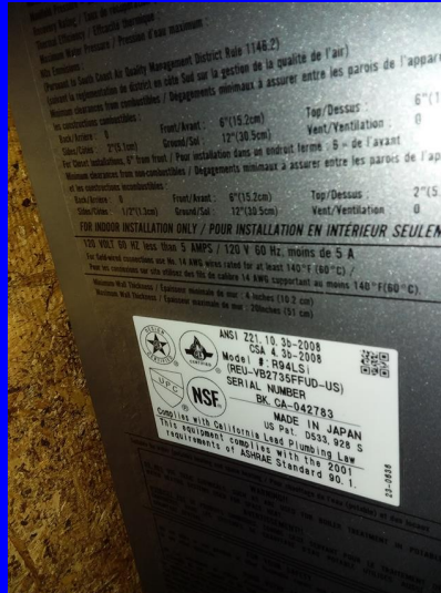
water heater data plate
