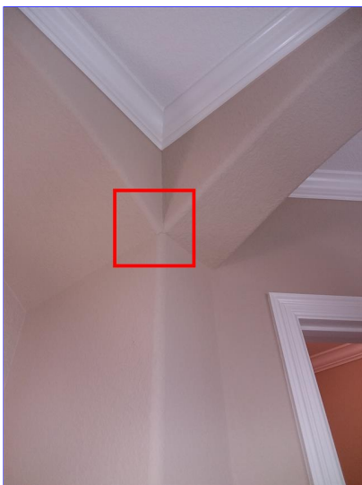
F. Item 4(Picture) primary bath
