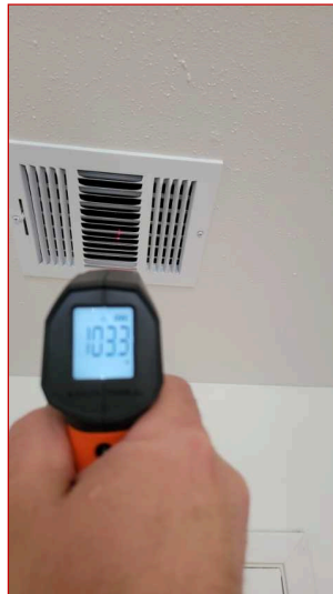
Heater supply temp 103.3 degrees.
