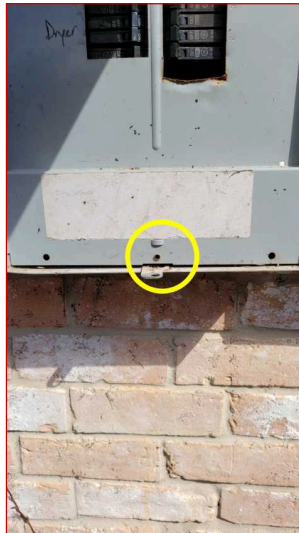
Missing screw to secure dead front cover.
