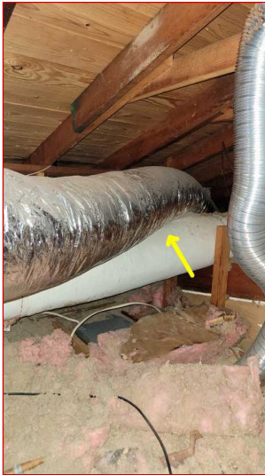
Ductwork should not be touching.
