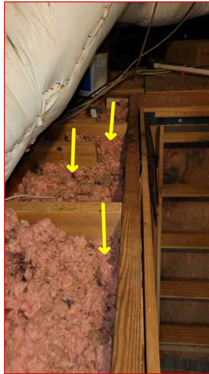
Insulation is low in one or more spots. Should be replaced.
