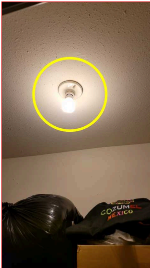
Light cover(s) missing in one or more locations.
