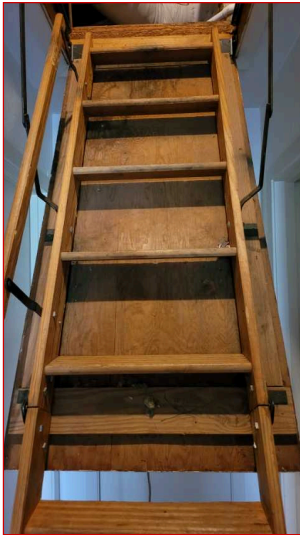
Attic ladder is not insulated or weather stripped at this time. This is an "As Built" condition that does not meet current energy standards. It is recommended to insulate the hatch door after taking ownership of the property.
