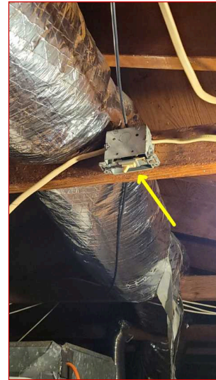
Damaged and/or missing outlet and/or switch covers were observed. This situation creates a Safety Hazard and should be corrected
