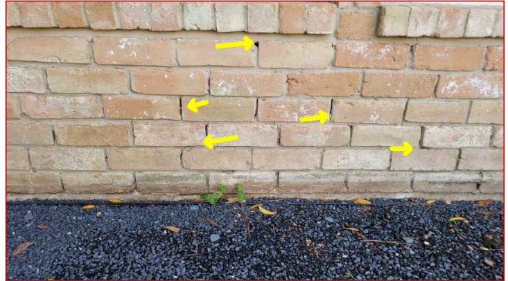
Mortar thin in multiple areas around home.
