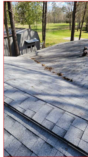
Debris should be removed from the roof covering and/or gutter system.
