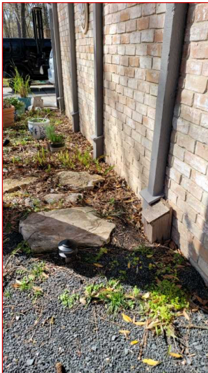
Earth to siding contact was observed on the exterior siding and should be a minimum of {4"} clearance from the ground for brick/stone {6"} for wood and {8"} for stucco. Common in older homes.
