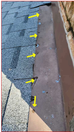
Nails exposed and Should be caulked. This is common maintenance.
