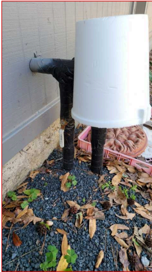
Water cut off on the north side of home.
