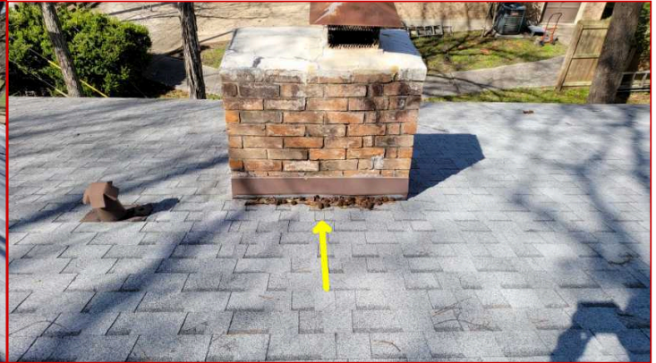
Cricket flashing needed.
