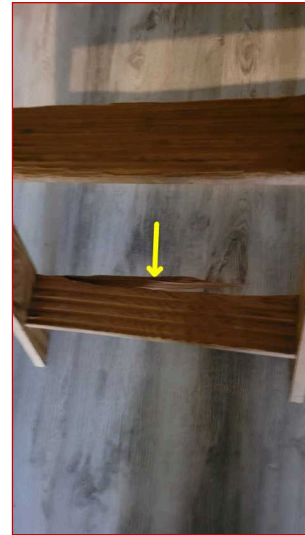
One or more of the attic ladder components were observed to be damaged and should be corrected for safety reasons.
