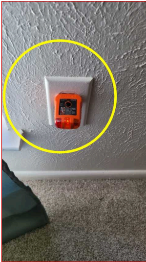
Open ground(s) noticed at one or more locations around the home.
