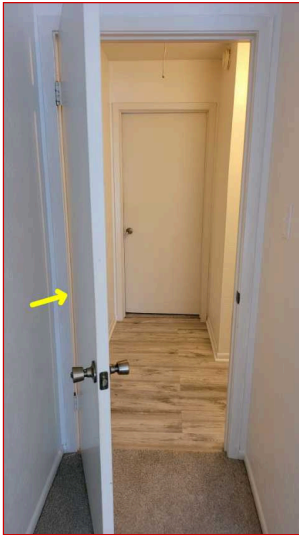
One or more doors were closing on there on. May need adjusting. Common in older homes.
