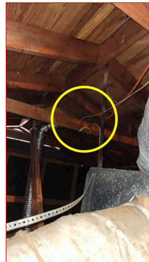
Electrical wire not properly secure in one or more locations.
