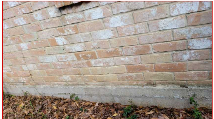
There were no weepholes observed in the lower course of the masonry veneer in one or more areas of the structure. Under current building standards; there should be open weepholes not less than {3/16"} in diameter on the lower course of the masonry wall and spaced no more than {33"} apart to drain excess water from the interior of the wall voids.
