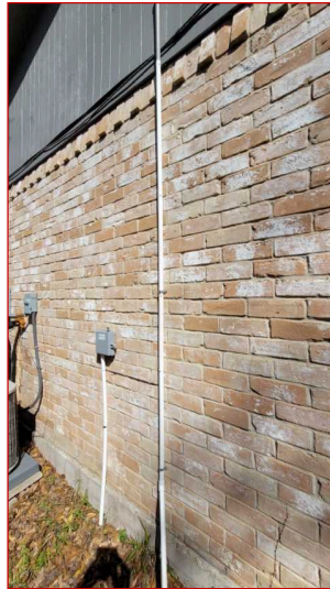
Drain pipes should be painted. They are not UV resistant.
