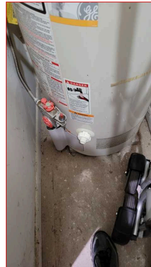
Water heater was not equipped with a corrosion resistant drain pan .
