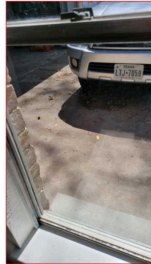
Window screens were observed to be damaged or missing in one or more locations.
