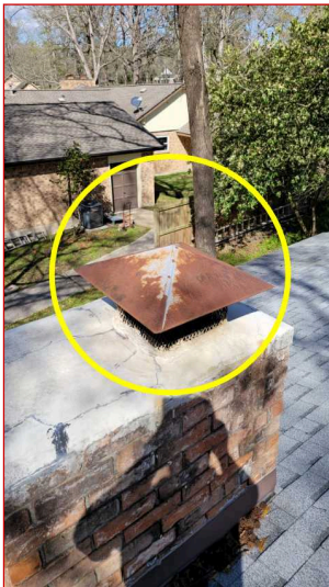
Chimney cap and or rain cap is rusty.
