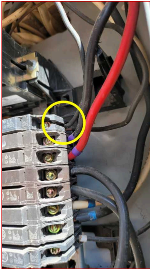
Double tap on breaker(S) were observed in the service panel. One wire under each screw is recommended.
