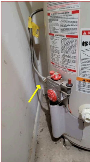
No sediment trap on gas line.
