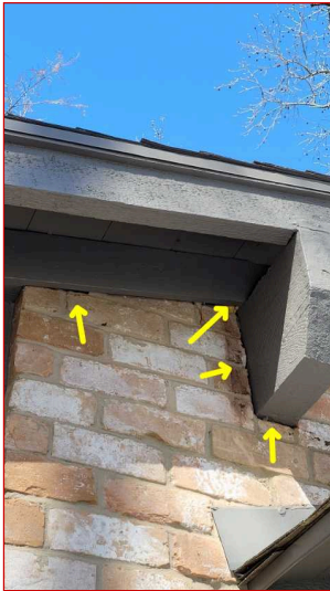
Caulking needed at one or more places around the home/building. This is common maintenance.
