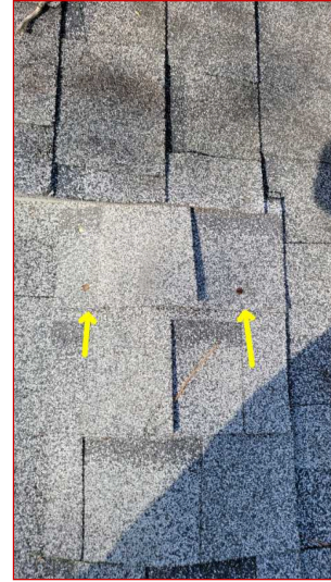
Nails exposed and Should be caulked. This is common maintenance.
