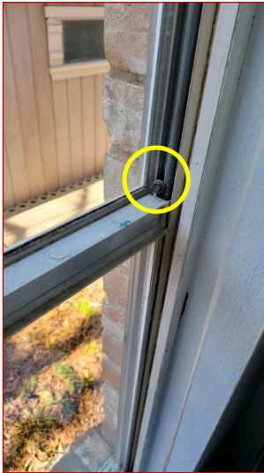
Window(s) would not open in one or more locations.
