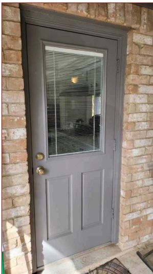
Doors between the garage and the residence should be equipped with a solid wood door not less than {1 3/8"} in thickness, solid or honeycomb core steel door not less than {1 3/8"} thick or {20} minute fire rated doors equipped with a self closing device.
