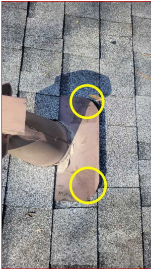
Nails missing from flashing.
