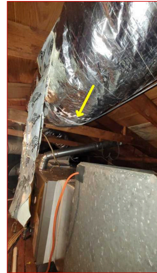
Ductwork is leaking at connections.
