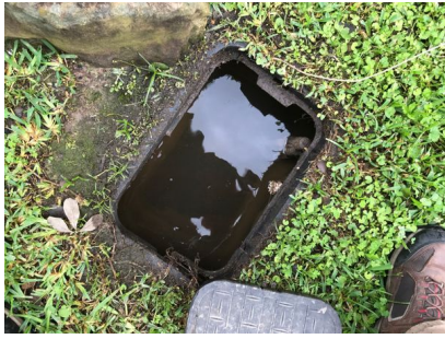
Location of Main Water Supply Valve : Exterior wall- Front
