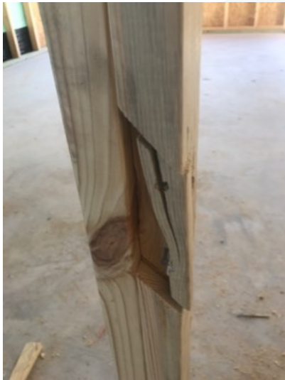
Damaged king stud in the master bathroom
