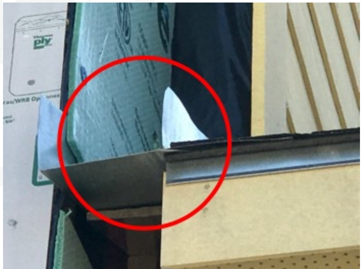
Missing kick out flashing
