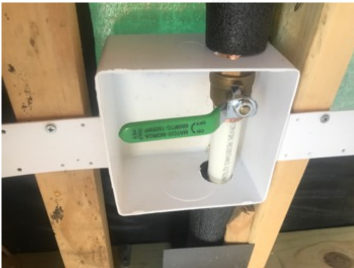
Main water shut off valve
