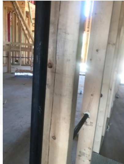
Cracked framing member
