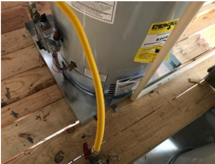
water heater drain pan
