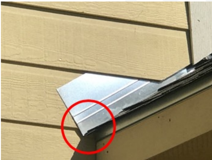
Missing kick out flashing
