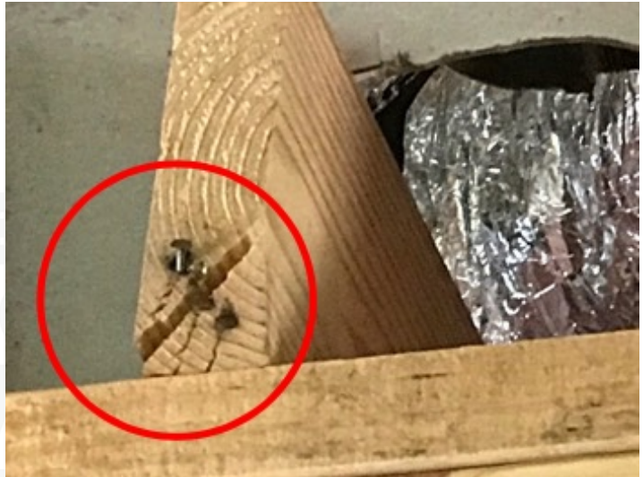
Broken framing member
