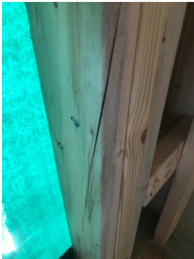
Cracked framing member
