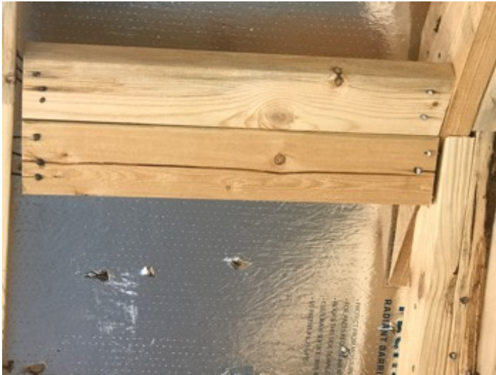
Cracked framing member
