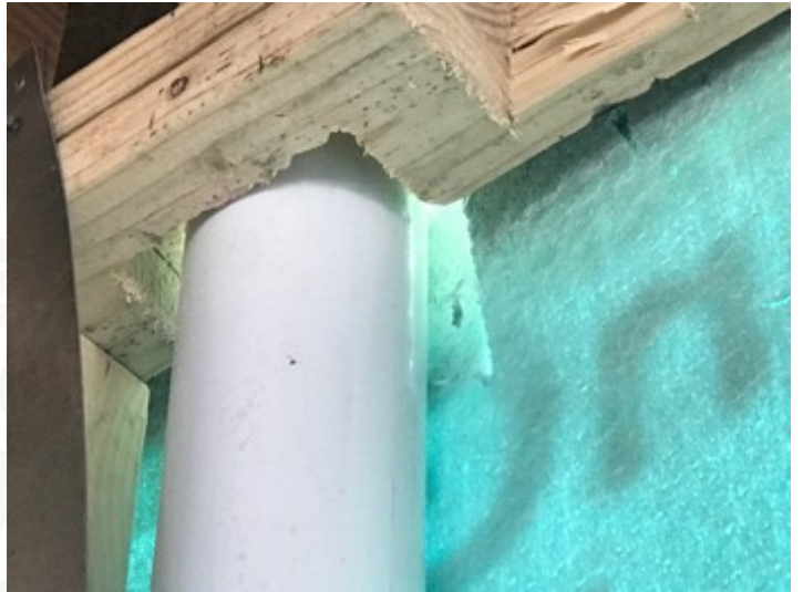
Missing steel reinforcement
