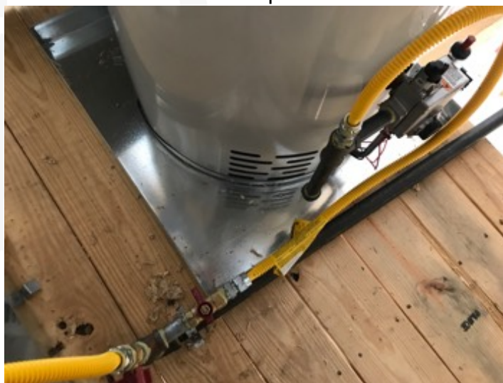
water heater drain pan
