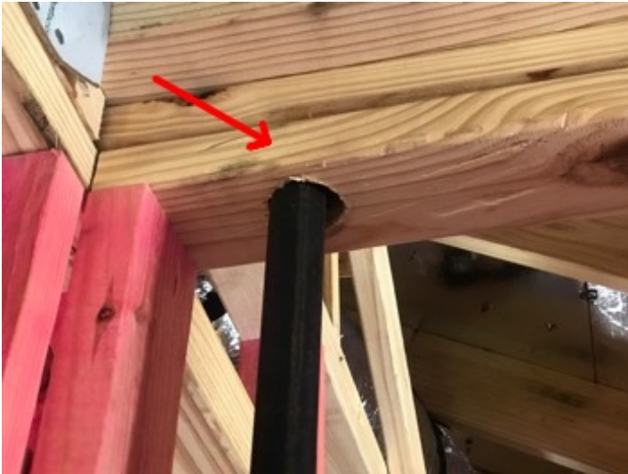
Missing steel reinforcement
