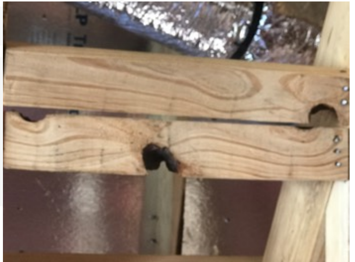
Less than quality material used for framing members.
