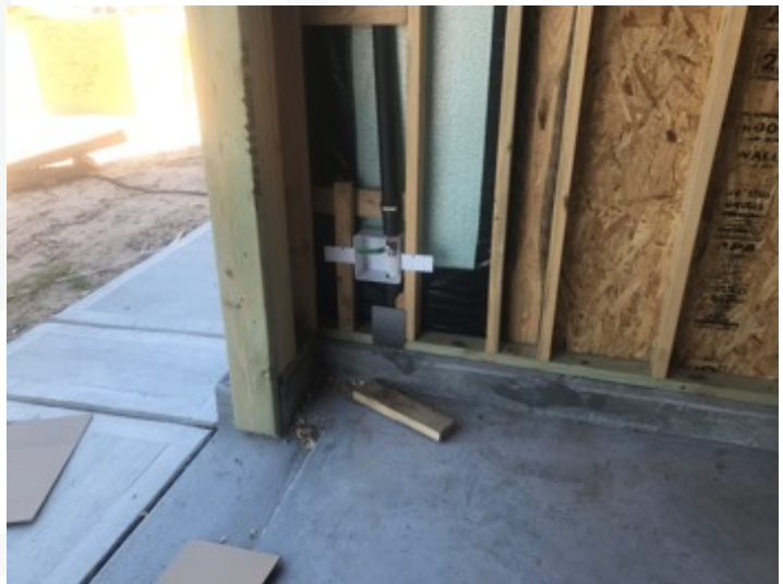
location of main water shut off valve
