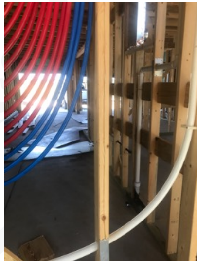
Cracked framing member
