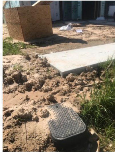
Location of water meter
