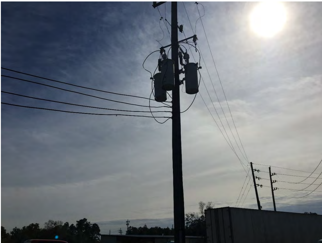
8. A view of the three pole-mounted electrical transformers observed near the eastern boundary of the subject site. No visible staining or leakage was observed.
