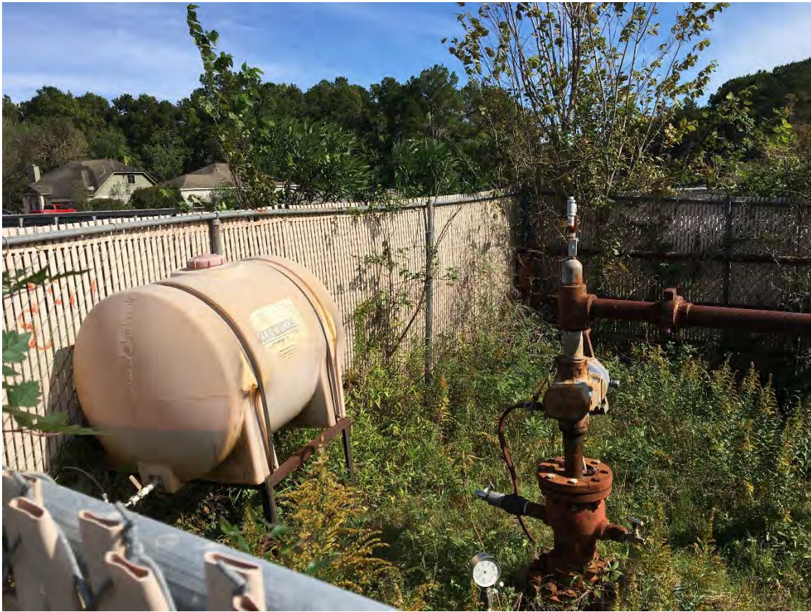
9. A view of AST and plugged oil well located on the subject site. Rusting is visible, but no leakage, stressed vegetation, or staining were observed underneath.
