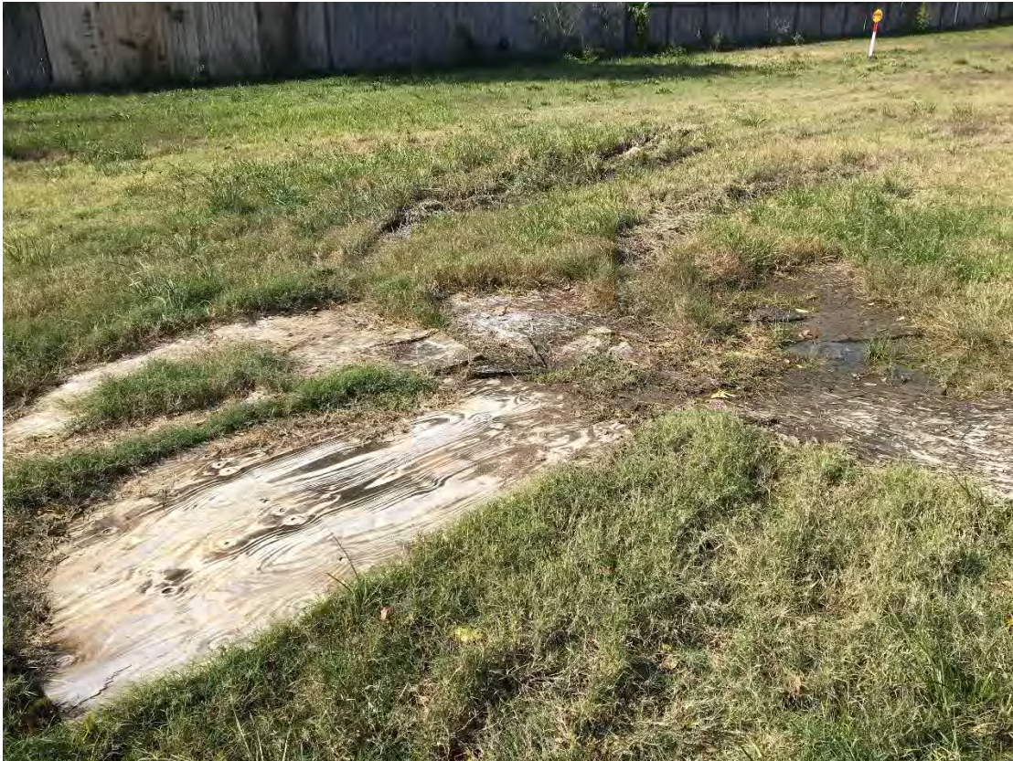
7. A view of some of the solid waste (wooden debris) that was observed throughout the subject site.
