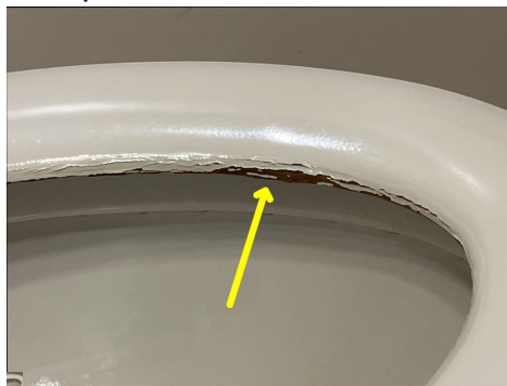
Observed damage to both commode seats.
