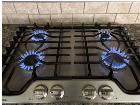
Gas cooktop in operation during the gas re-inspection.
