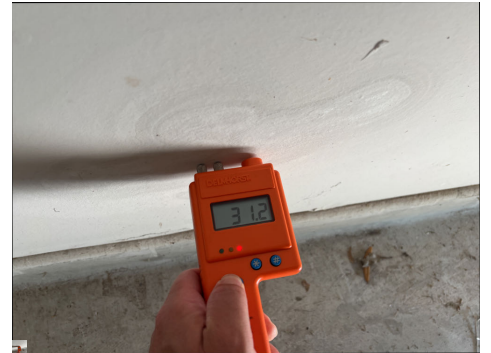
Water stain on the north interior garage wall was wet at the time of inspection.
