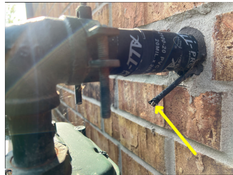
Gas bond wire has been disconnected.
