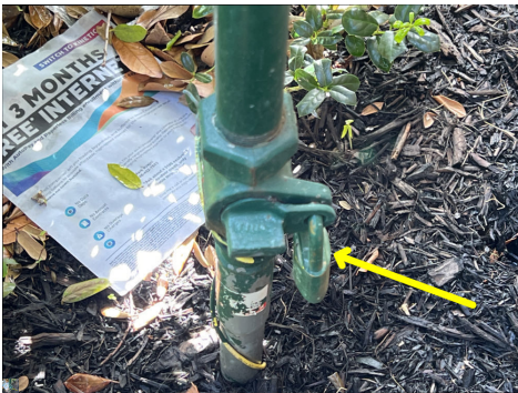
Gas service was locked in the off position at the time of inspection.
