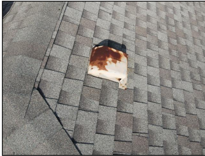
12. Exposed fasteners not sealed
