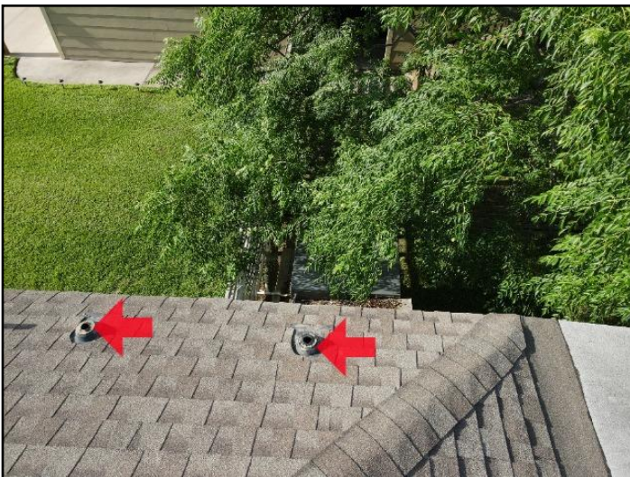
9. Installation incorrect (top exposed or...
