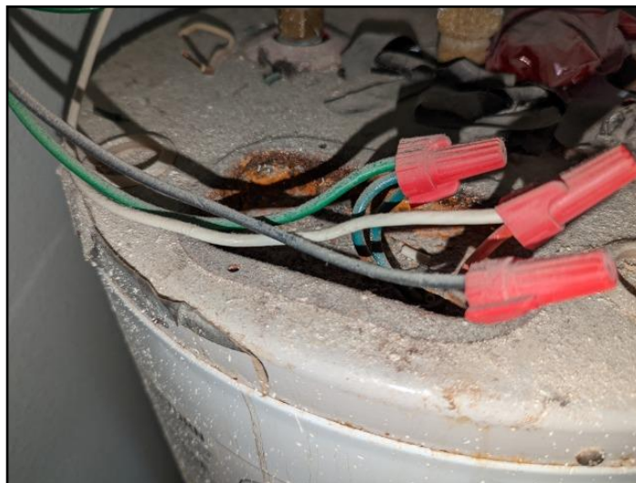
53. Tank not electrically bonded to ground
