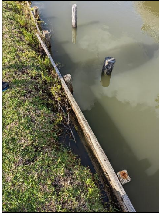
88. Bulk Head In disrepair
