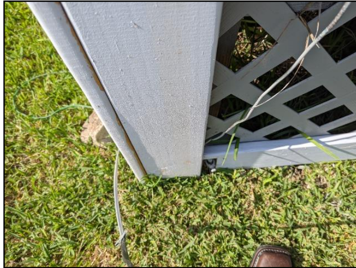
27. Copper - ground rods
