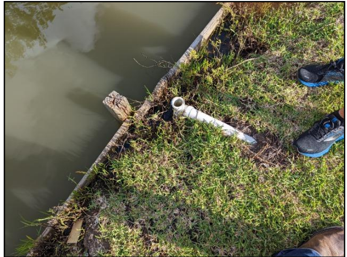
87. Bulk Head In disrepair
