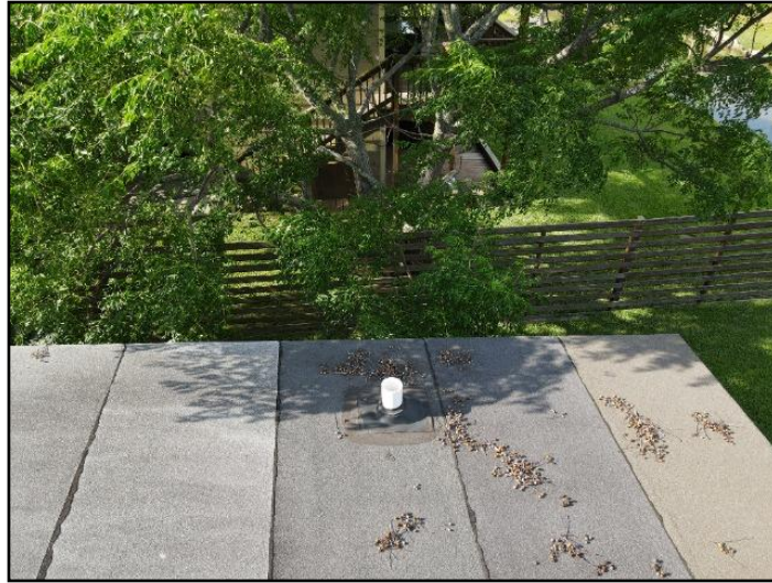
7. Tree branches touching roof
