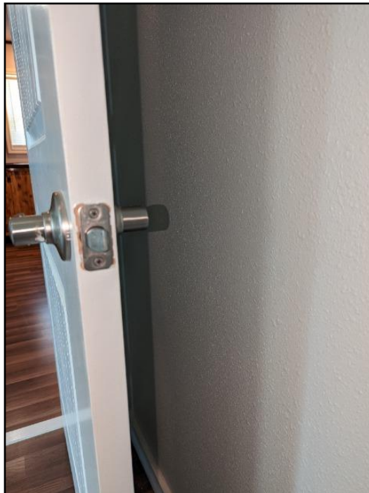
76. Doorstops missing or ineffective
