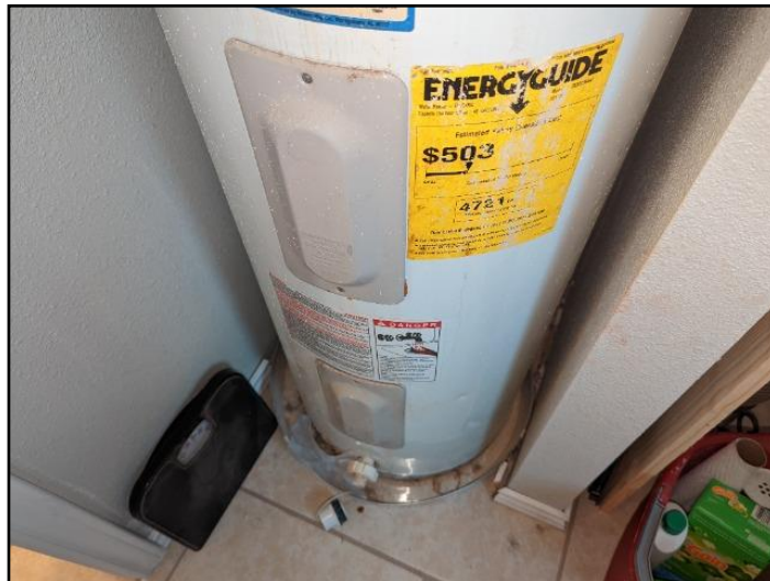
51. Safety pan and drain defect
