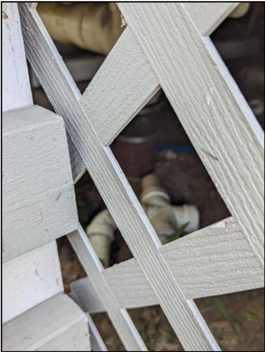
56. Clean-outs missing or inaccessible
