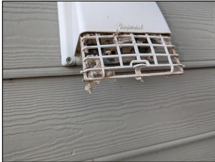
85. Dryer vent obstructed
