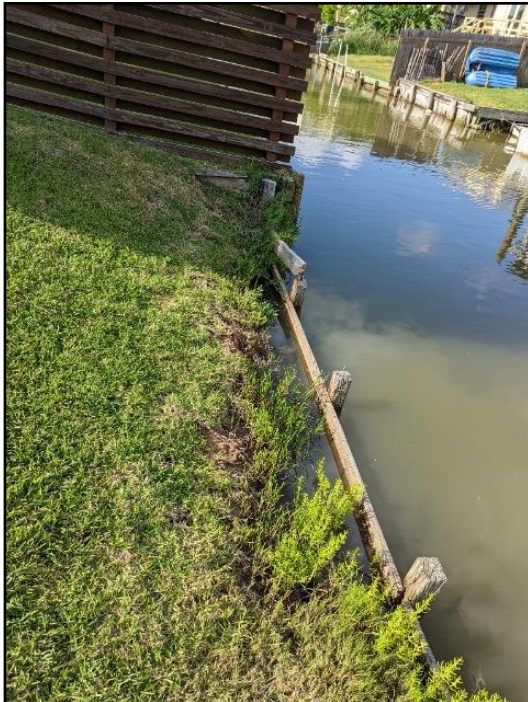
86. Bulk Head In disrepair
