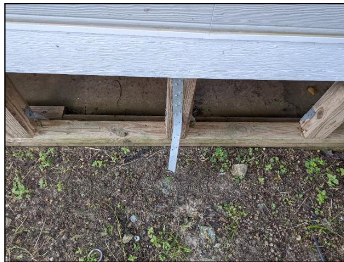
25. Anchors not centered in sill
