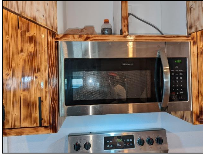
81. Not vented to exterior
