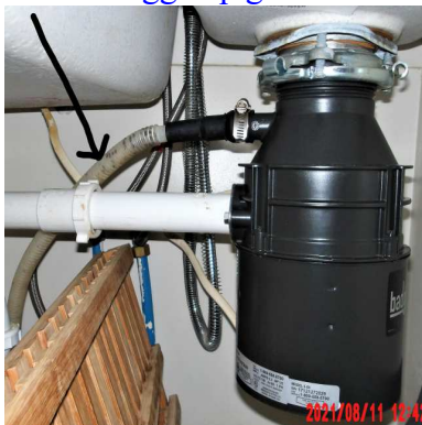
No anti-siphon device.
