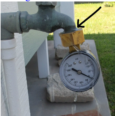
No backflow device.
