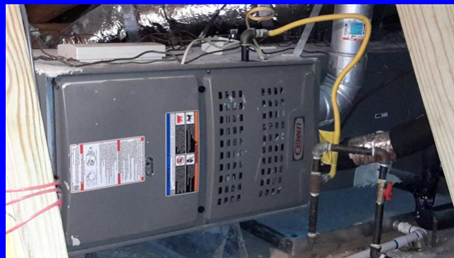
Lennox gas furnace
