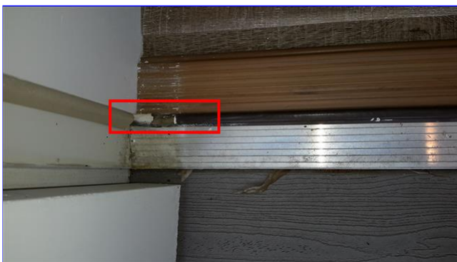
G. Item 1(Picture) damaged weather stripping second floor patio
