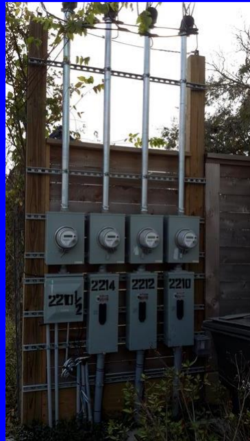
Above ground service with 150 amp disconnect
