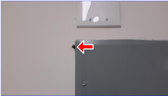
E. Item 26(Picture) garage right wall
