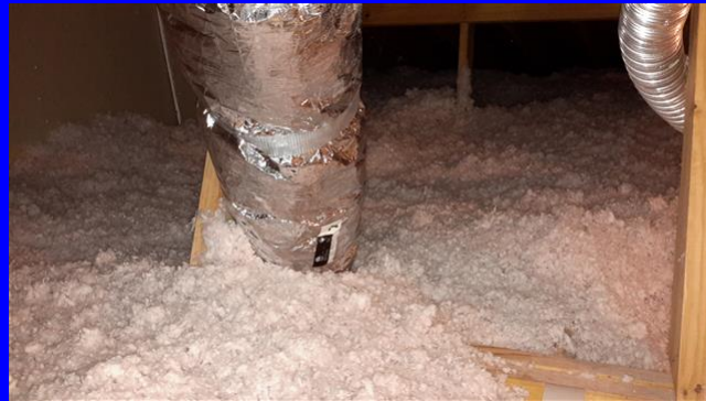
12 inches blown insulation
