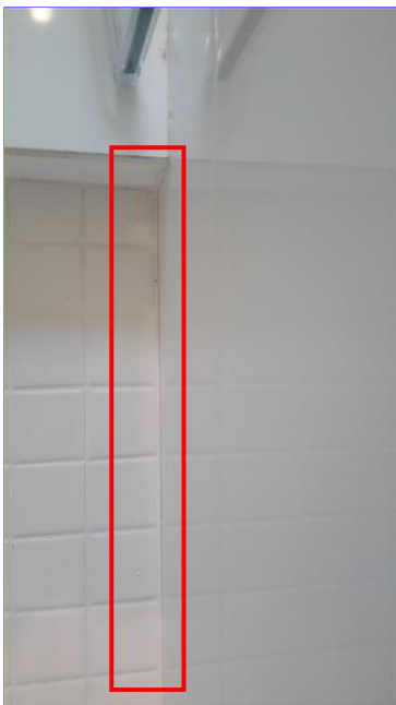
E. Item 31(Picture) master shower
