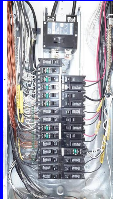
150 amp main panel located in garage
