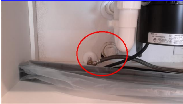
E. Item 10(Picture) kitchen under sink
