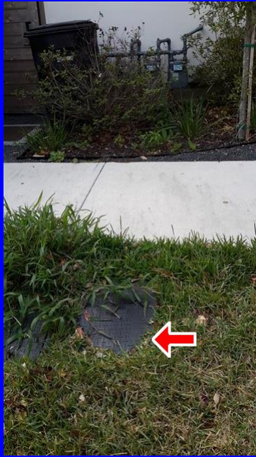
Water meter at street
