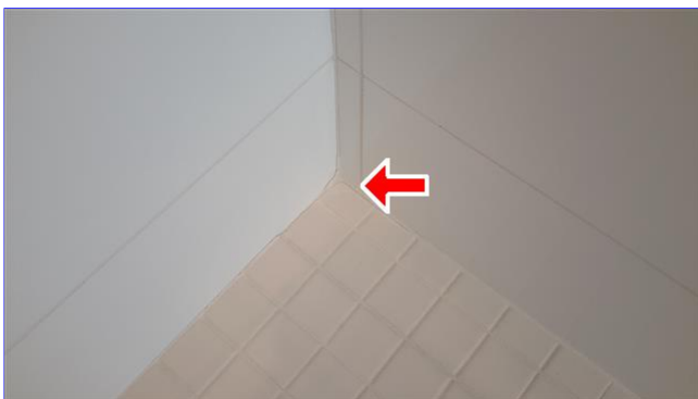
E. Item 34(Picture) master shower
