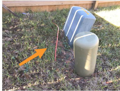
Cable Needs To Be Buried In Back Yard
