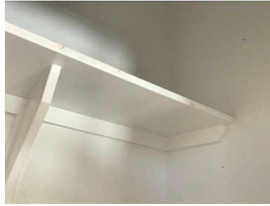
Touch Ups Needed In Dining Room Closet
