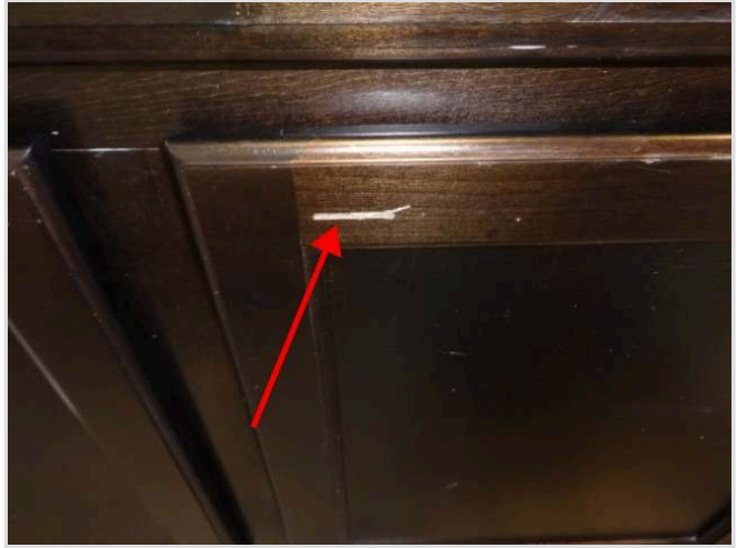
Damage to hallway bath cabinet door
