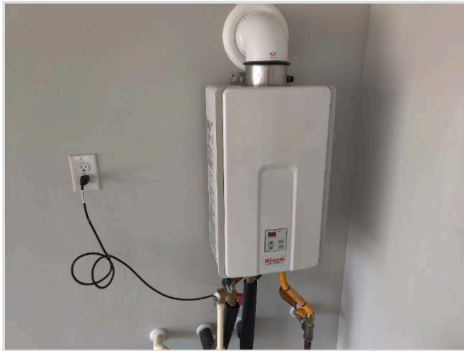
Water heater - garage
