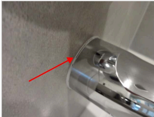
Gap in tub spout sealant
