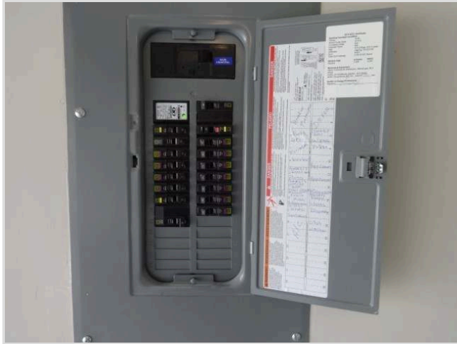
Main Service Panel
