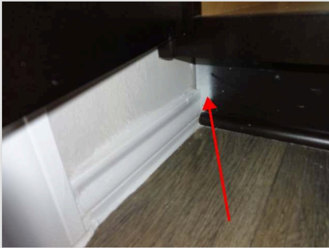
Over spray on master bath cabinet kick plate
