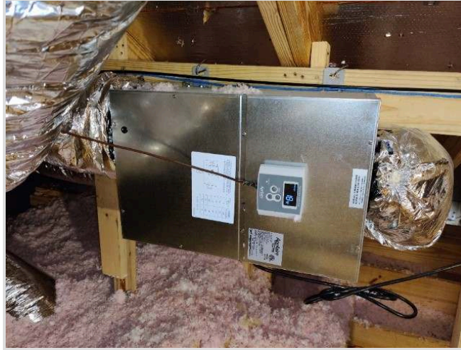
Fresh air exchanger in attic
