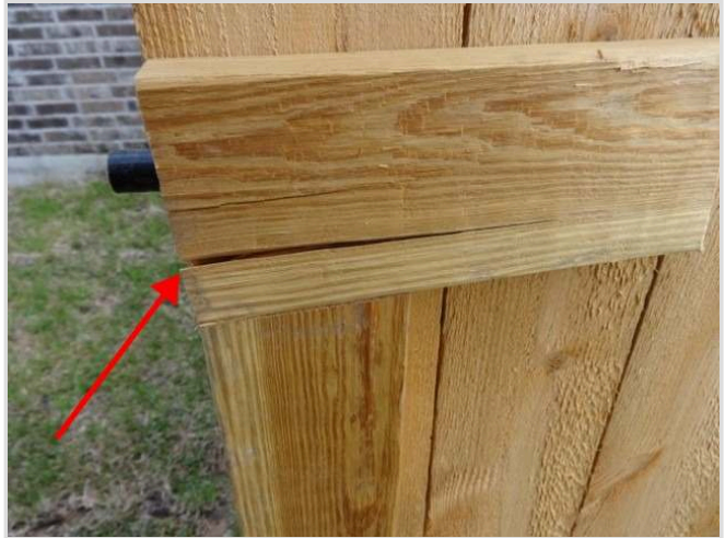
Cracked 2x4 - fence gate
