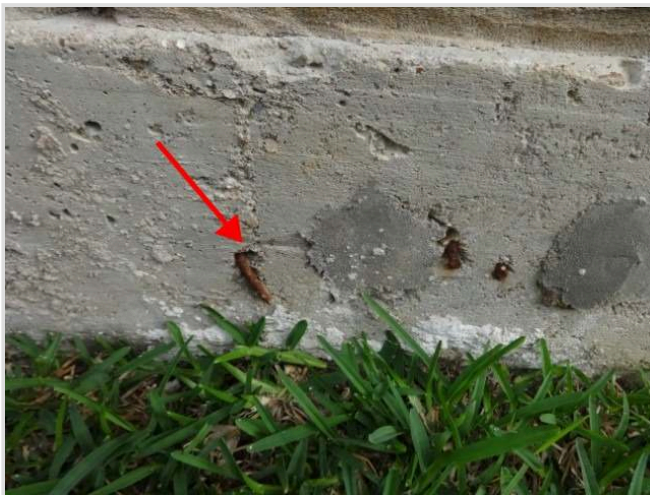
Exposed nails on right side exterior beam
