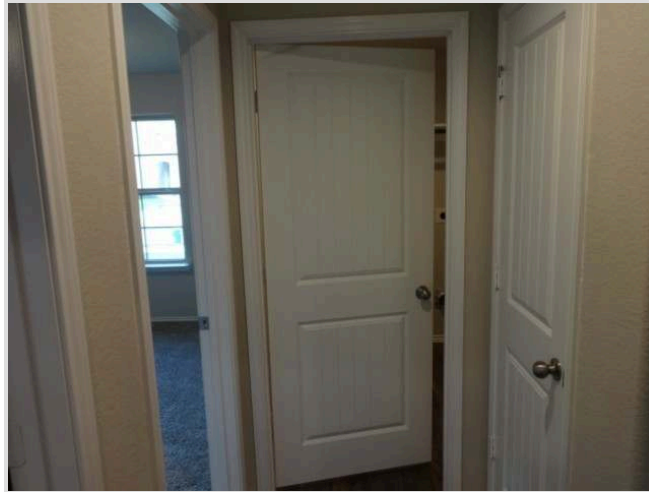
Laundry room door would not latch
