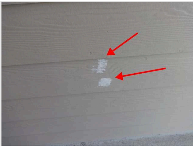
Paint mark - Front porch siding
