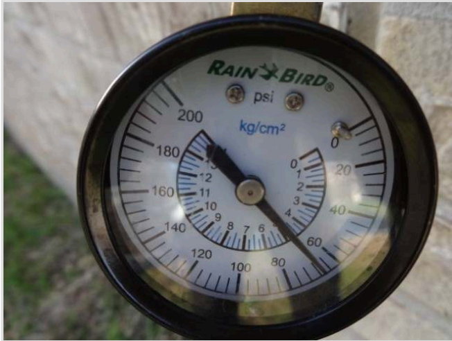
Water pressure reading
