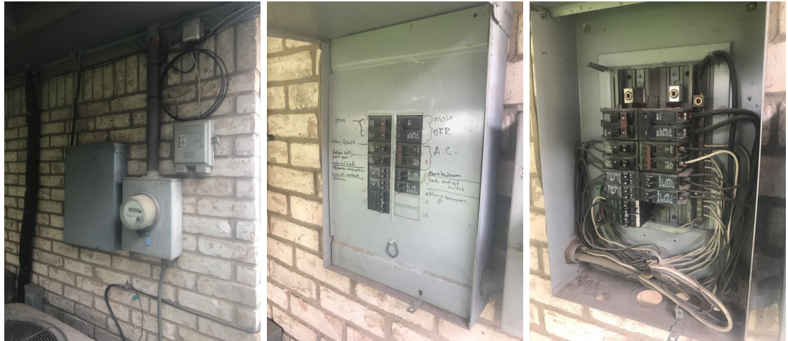
General Infrared Photos of Distribution Panel(s):
