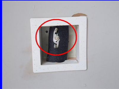
water shutoff inside garage left side
