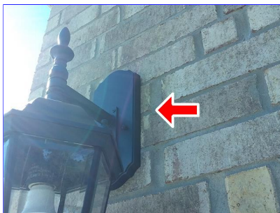
L. Item 3(Picture) multiple areas exterior outlets and service panels
