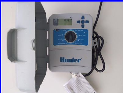
sprinkler system control panel inside garage
