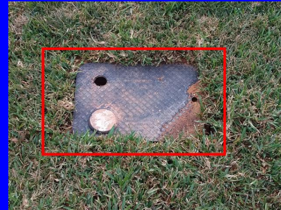
water meter front left of home
