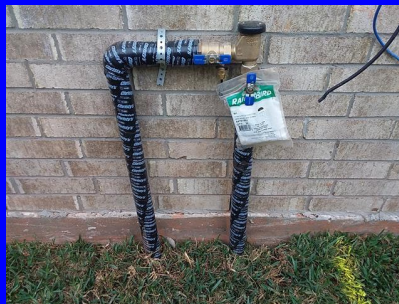
backflow preventer left side of home
