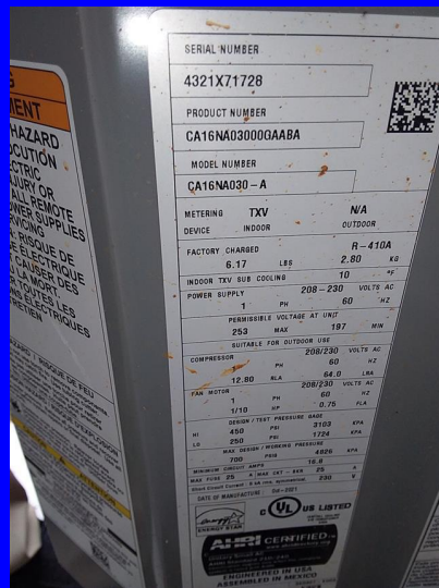
mfd 2021 25 amp maximum breaker
