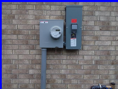
meter box and main disconnect box left side of home underground service
