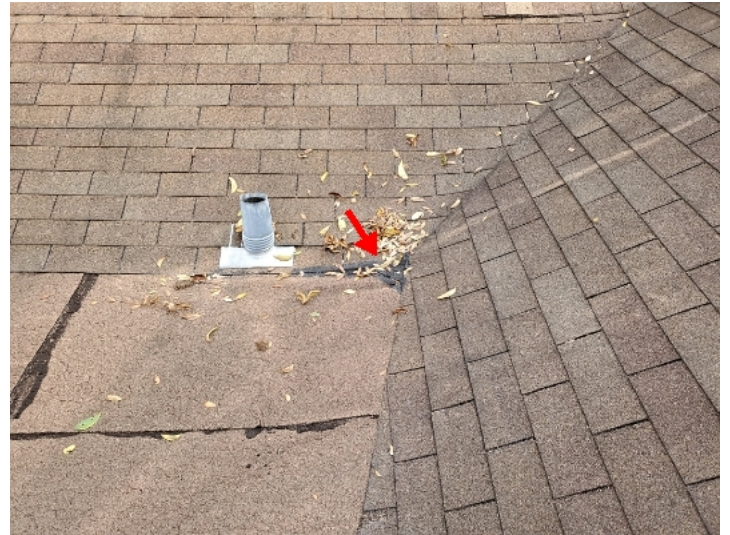
Evidence of sealing leaks.
