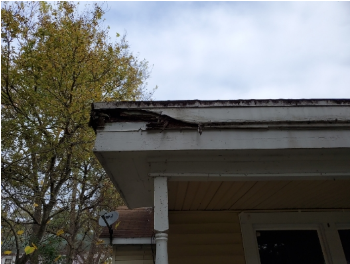
Damaged fascia board on left front of porch.
