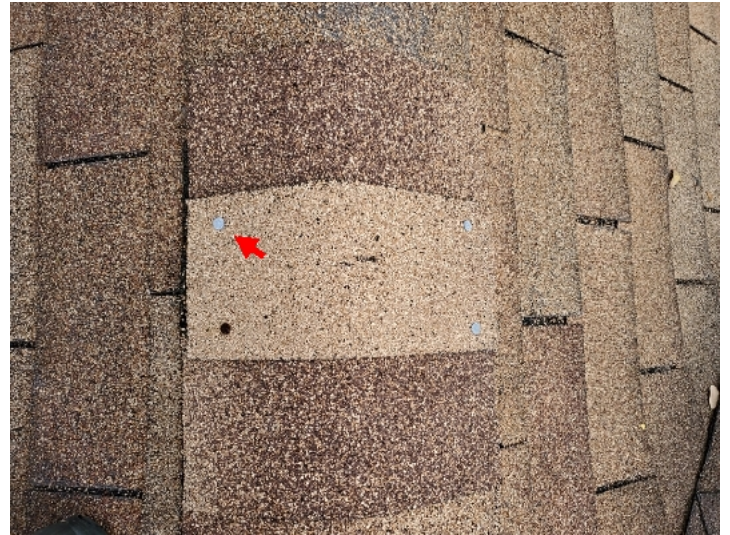
Multiple exposed nail heads.
