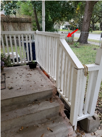
The hand rail on the front steps needs to be stabilized.
