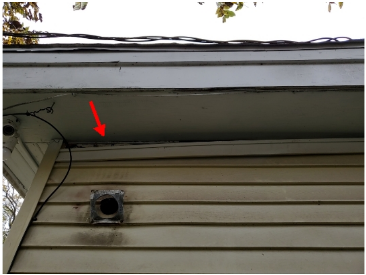
Loose vinyl siding on left rear of house.
