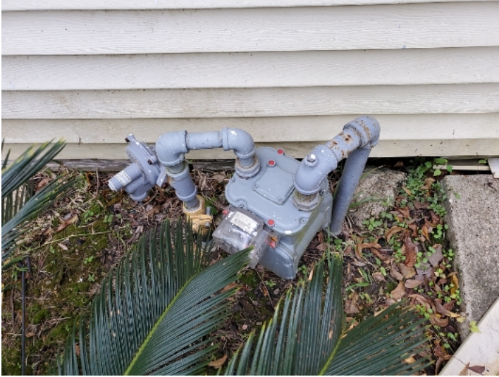
Gas meter is still present.
