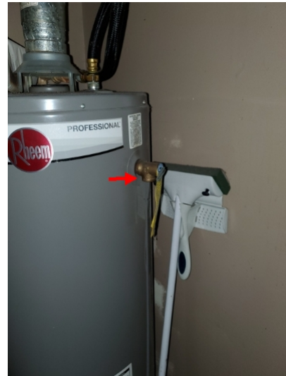
The TPR valve is not plumbing to a safe location.
