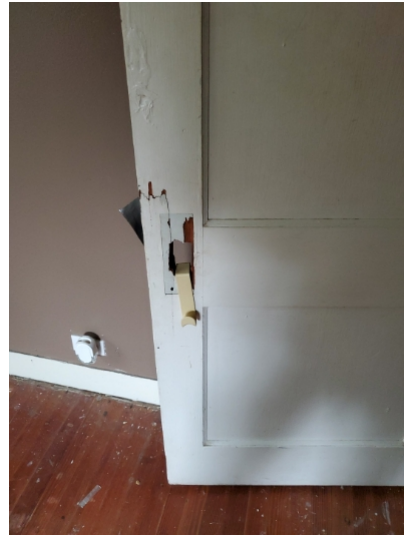
Various damage to interior doors and hardware.
