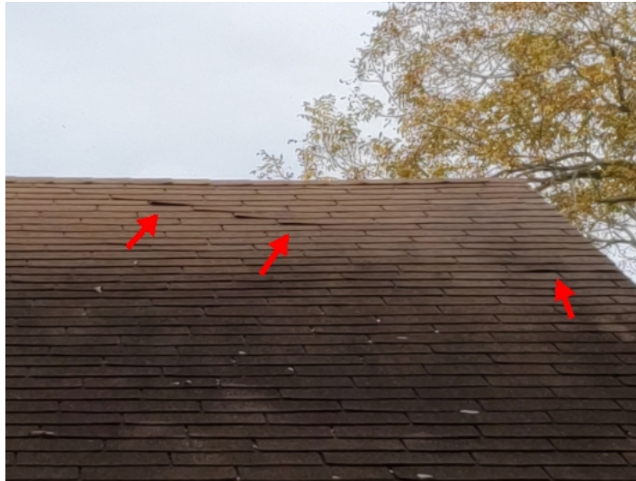
Various lifted shingles on roof.
