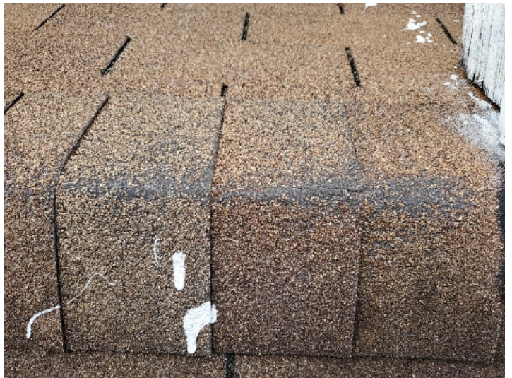
Wear on ridge cap shingles.
