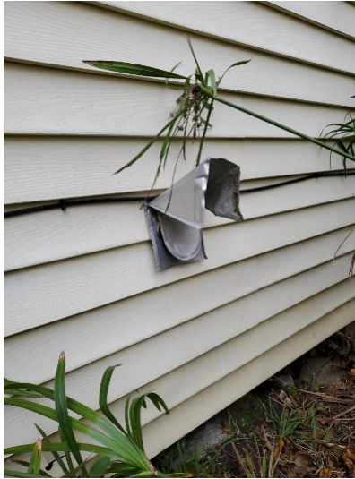
Damaged dryer vent damper is in need of replacement.
