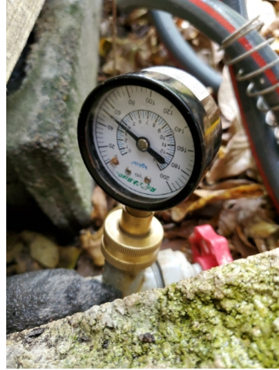
The anti static water pressure was observed between 45-55 PSI. Acceptable water pressure is between 40 and 80 psi.
