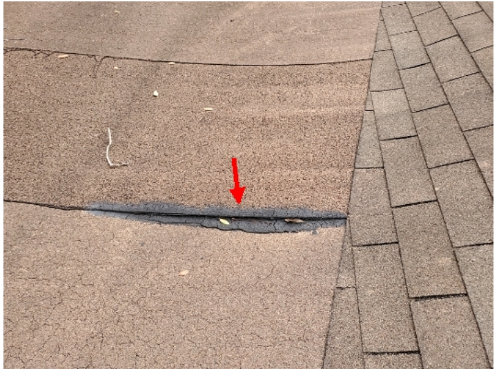
Evidence of sealing leaks.
