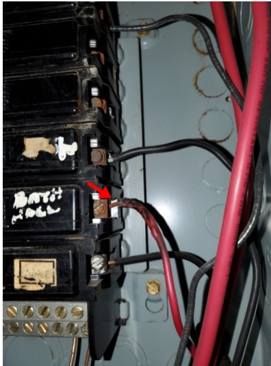
Charred wire in sub panel.
