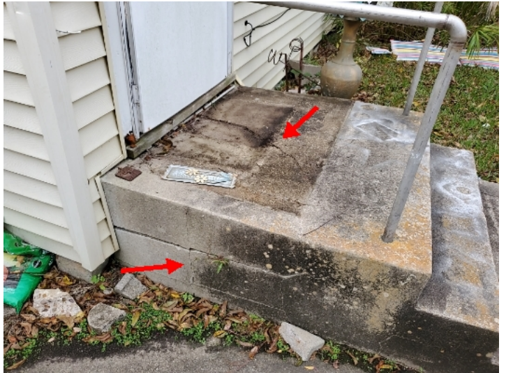
Large settlement cracks on back door steps.
