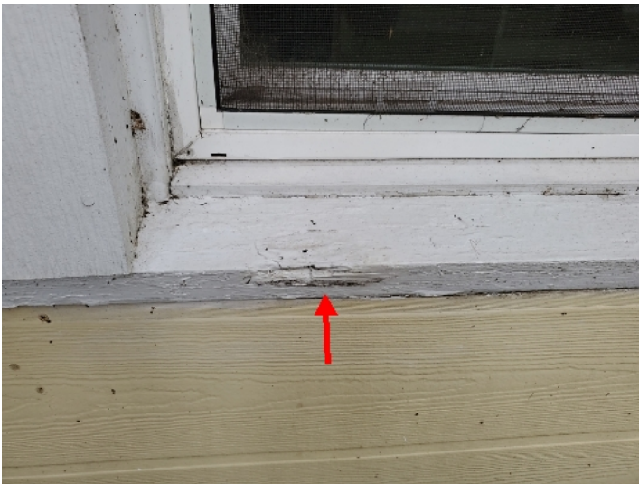
Various damaged window sill around exterior of the house.
