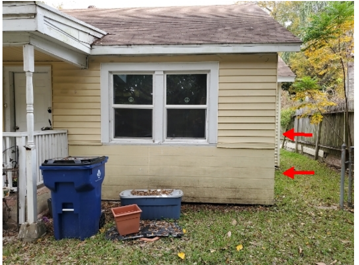
Mismatched of exterior siding on front of house.
