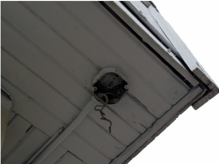
Exposed outlet box on rear of house above back door.
