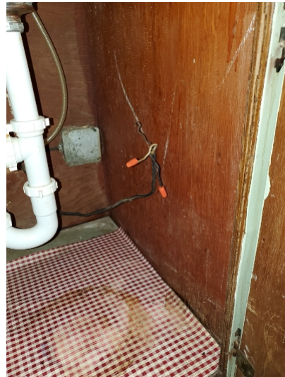
Exposed wires underneath kitchen sink.
