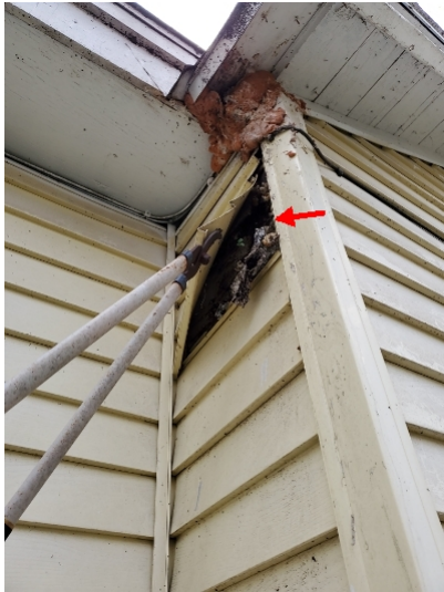
Water damaged siding in left middle of exterior.
