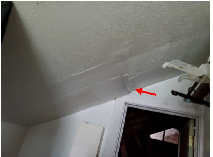
Various ceiling drywall damage in converted attic space.
