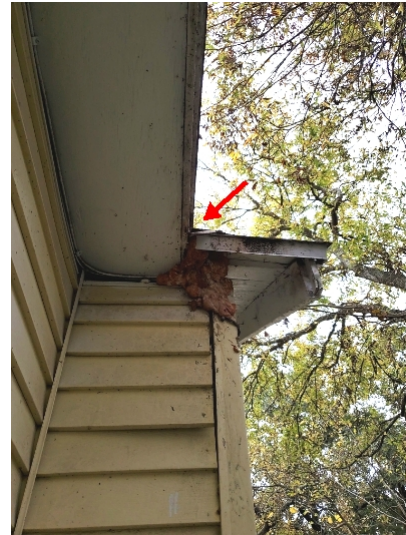
Improper/flashing that is not working properly on left middle of exterior.
