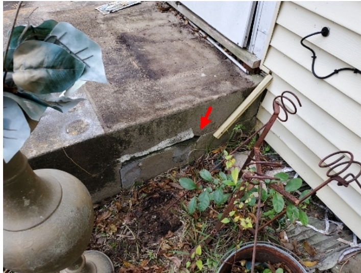
Large settlement cracks on back door steps.
