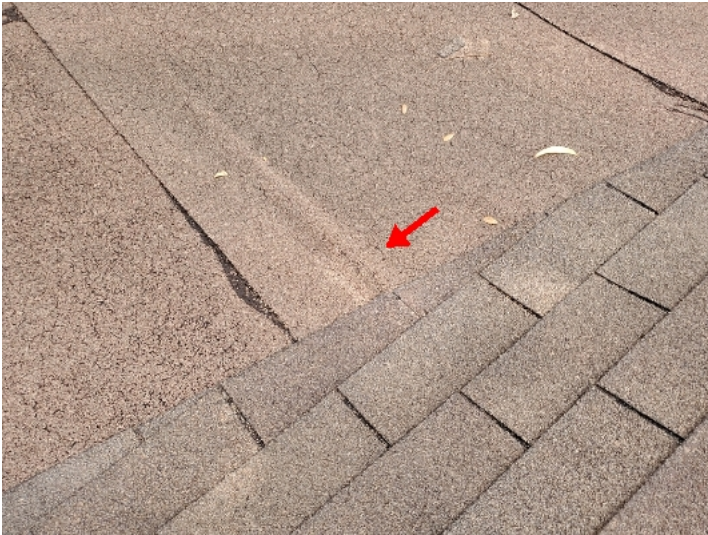
Wrinkled roll roofing material.
