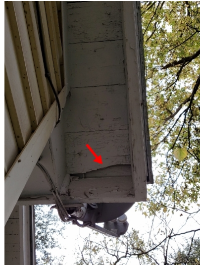
Decking and fascia damage on left middle of exterior.
