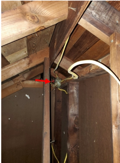
Open junction boxes and light fixtures that are not properly installed in attic.
