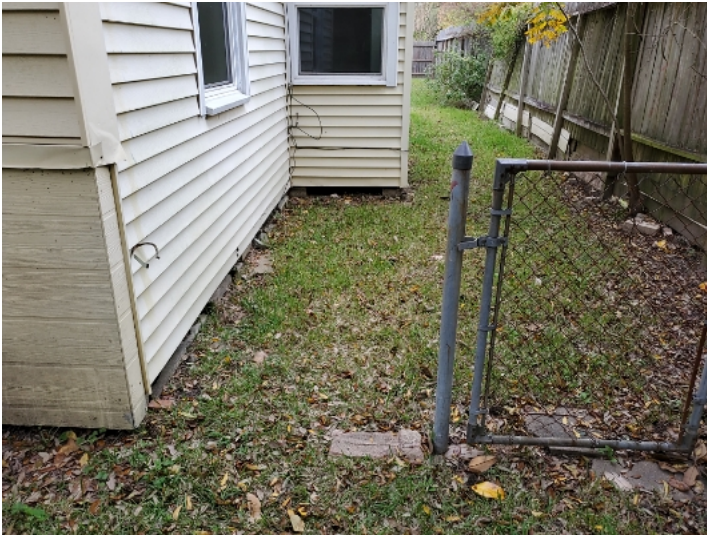
Missing section of fence on right front of house.
