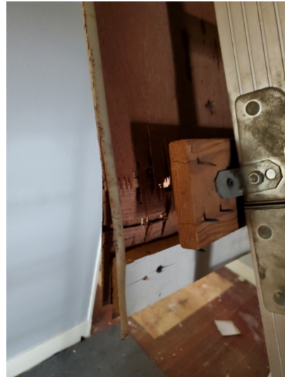
Damaged attic access ladder recommended repair/replace.
