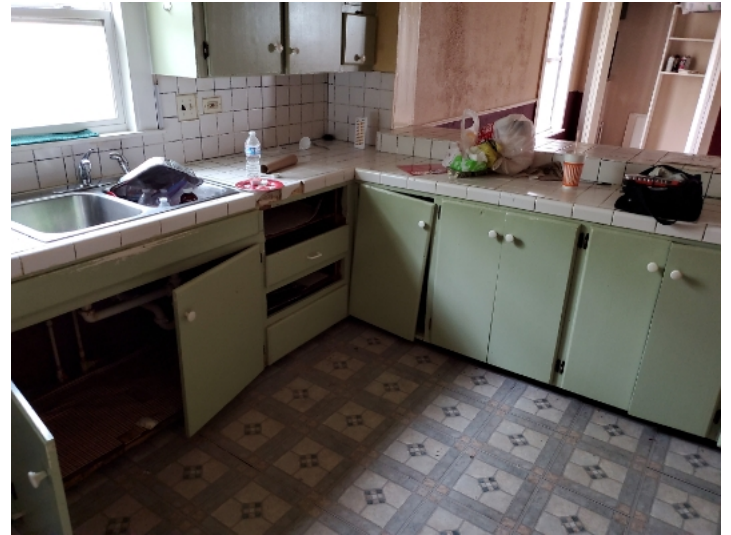
Kitchen cabinets are in poor condition and will need to be replaced.
