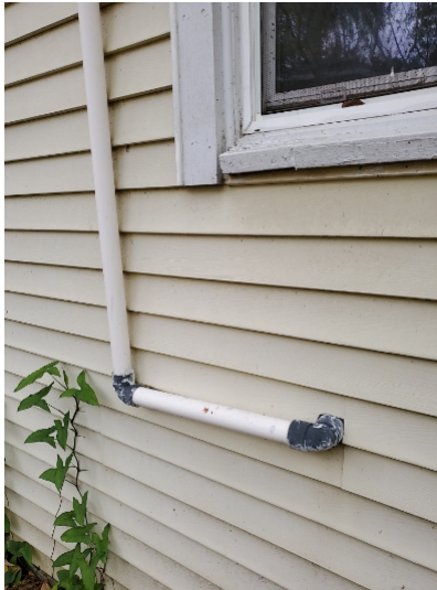
Kitchen sink vent stack in installed on the exterior of the house.
