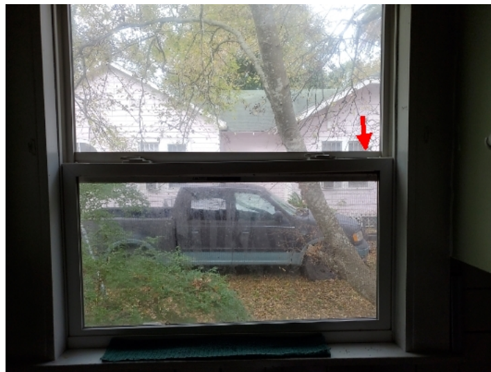
The frame for the window above the kitchen sink appears to be bent.
