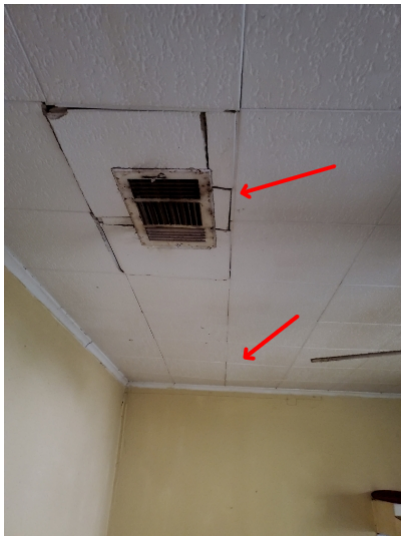
Damaged sections of kitchen ceiling.
