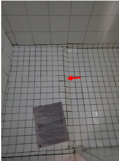
Loose tiles in Master bathroom shower.
