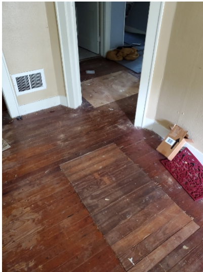
House will require new floors throughout.
