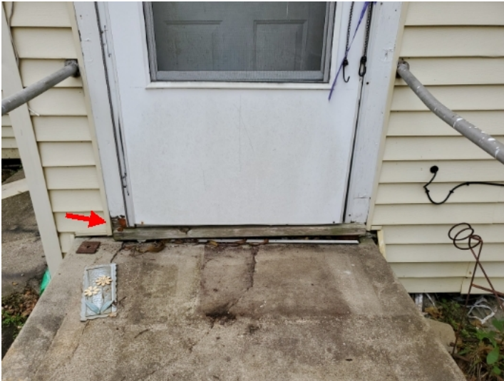
Damaged trim at the bottom of the back door.
