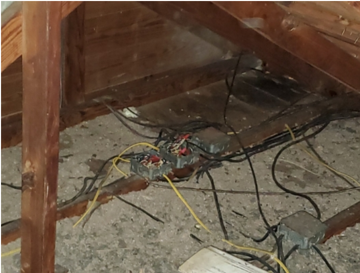
Open junction boxes and light fixtures that are not properly installed in attic.
