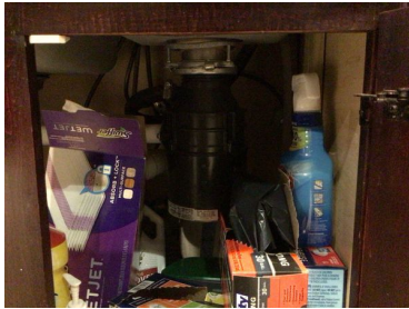
General Photos of Range Hood/Exhaust Systems:
