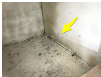
Under furnace/evaporator unit
