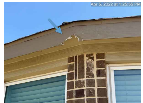
Damaged fascia board on back side of home
