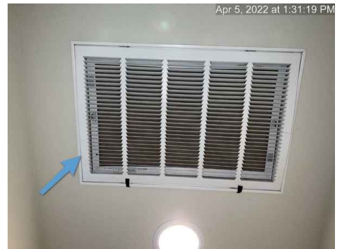
Filter cover located in front of master bedroom is bent and will need repair/replacement
