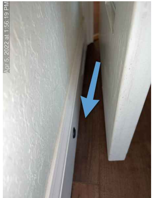
Not all door stops are in place.
