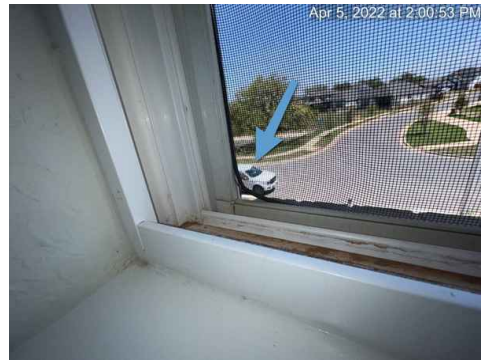
Upstairs window in family room has a torn screen
