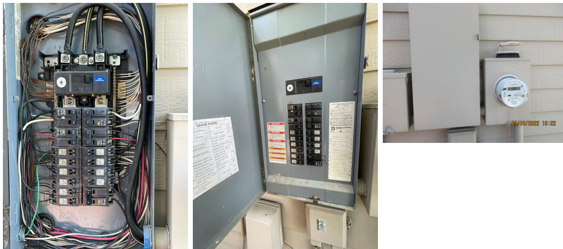
Amperage rating for main service disconnect: 200 Amps
