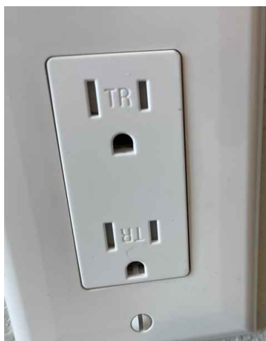
Tamper Resistant Outlet With The “TR” Embedded
