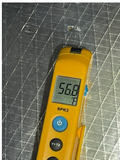
Temperature Differential Between The Return & Supply Air: Recommend having the HVAC system cleaned and serviced prior to closing, 13° - The temperature differential is normally expected temperature is between 15 and 21 degrees. This is where the inspector is taking a temperature reading from the supply air and subtracting it from the return air to get a total.
