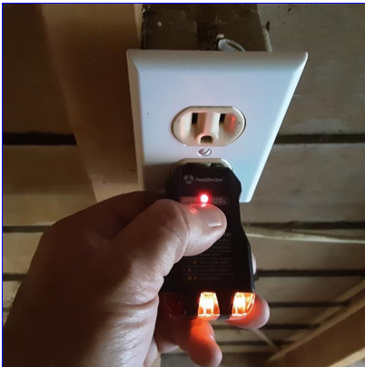
B. Item 3(Picture) Garage outlets
