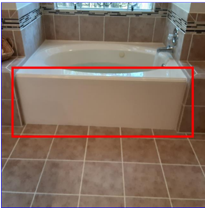
D. Item 1(Picture) No motor access
