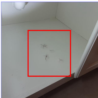
L. Item 2(Picture) 2nd floor guest bathroom, under right sink
