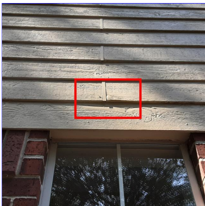
E. Item 2(Picture) Left side above bathroom window
