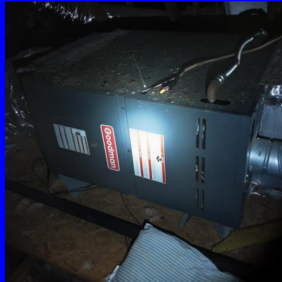
Goodman furnace in attic
