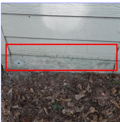
E. Item 4(Picture) Back of garage
