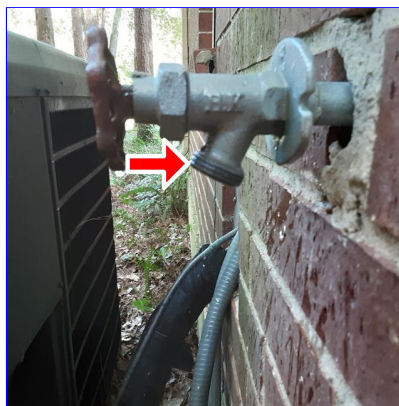
A. Item 7(Picture) Hose bibs
