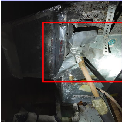
B. Item 4(Picture) At evaporator coil
