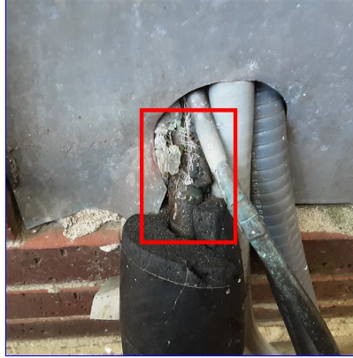
B. Item 2(Picture) At condensing unit
