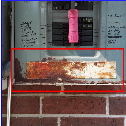
A. Item 3(Picture) Main panel
