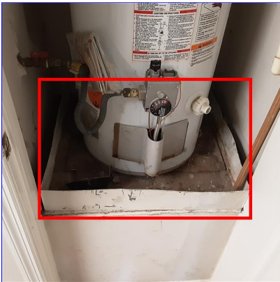
C. Item 6(Picture) Does not drain outside
