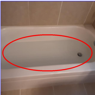
B. Item 2(Picture) 2nd floor guest bathroom tub
