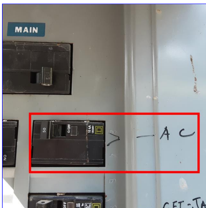
B. Item 14(Picture) 50 amp breaker for AC in main panel
