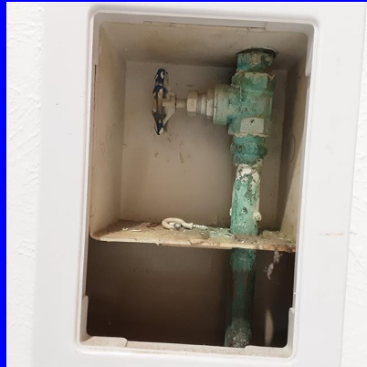
Main water shutoff in laundry room
