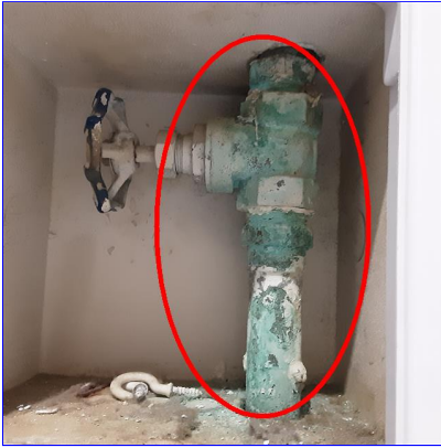
A. Item 1(Picture) Main water shutoff
