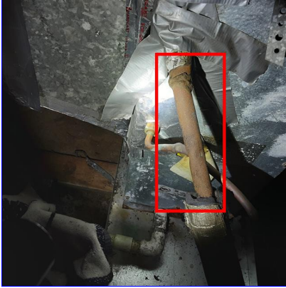
B. Item 1(Picture) At evaporator coil in attic
