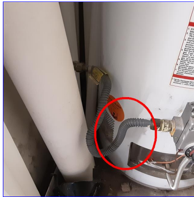
C. Item 3(Picture) No drip leg
