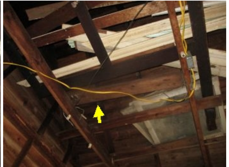
The exposed romex (electrical wire) in the garage area is required to be in protective conduit for safety reasons.
