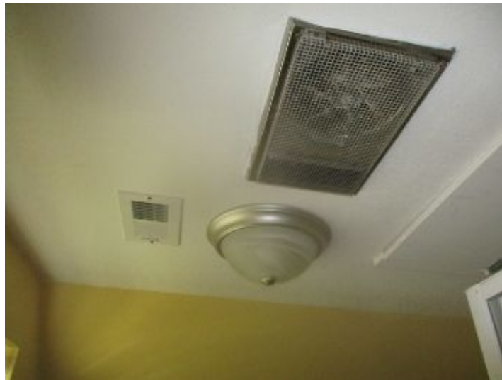
Heater / fan in upper bathroom did not function.
