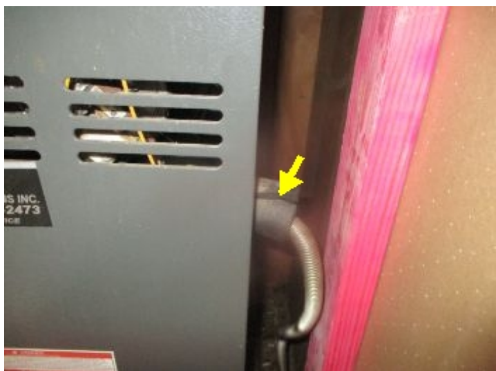
Lower: Use of flex gas line to the interior of housing, standards require hard pipe to be used inside of housing, does not meet industry standards.
