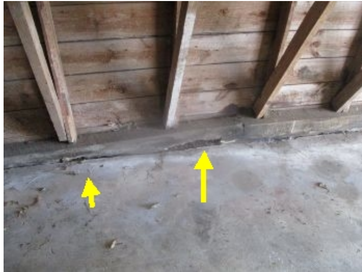
Rot to lower seal plates at garage.
