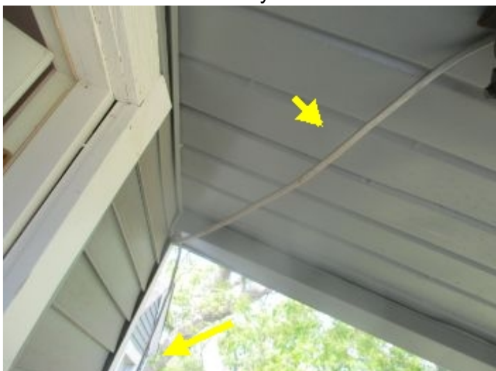
The exposed romex (electrical wire) at rear upper porch is required to be in protective conduit for safety reasons.
