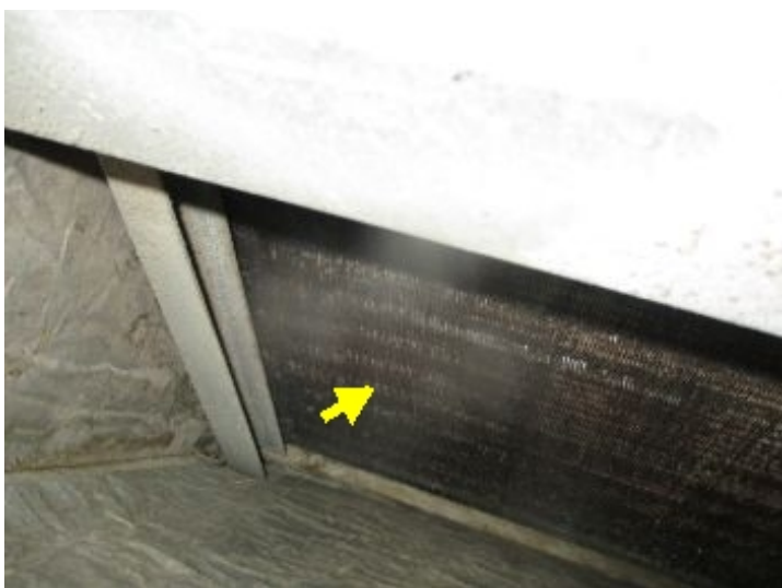
Coils are very dirty.
