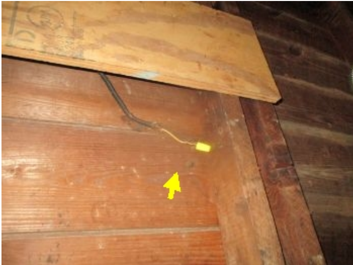
Non standard termination of romex (electrical wire) in garage.
