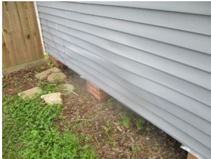
Warped exterior vinyl siding at left wall of home.
