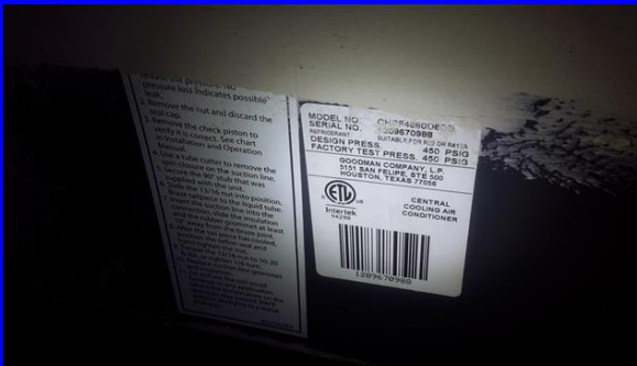
2012 Goodman 4 - 5 ton evaporator coil in attic
