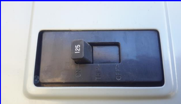
125 amp main service disconnect
