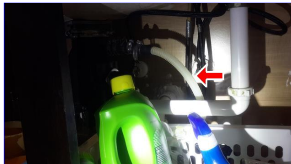
A. Item 2(Picture) Drain line
