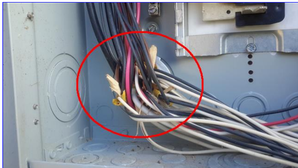
A. Item 1(Picture) Main panel
