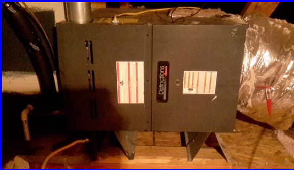
Amana furnace in attic
