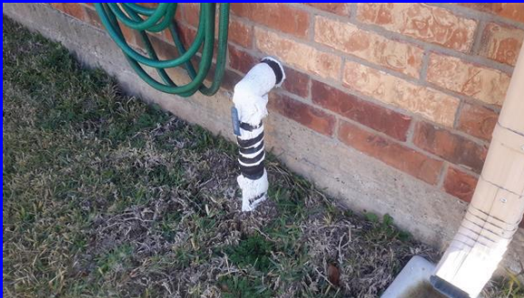
Main water shutoff
