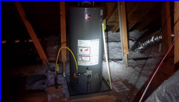
Water heater in attic
