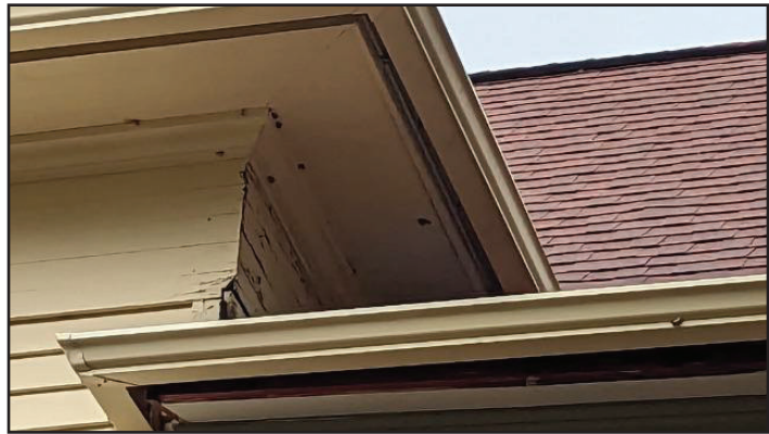
15. Vents - ineffective / missing
