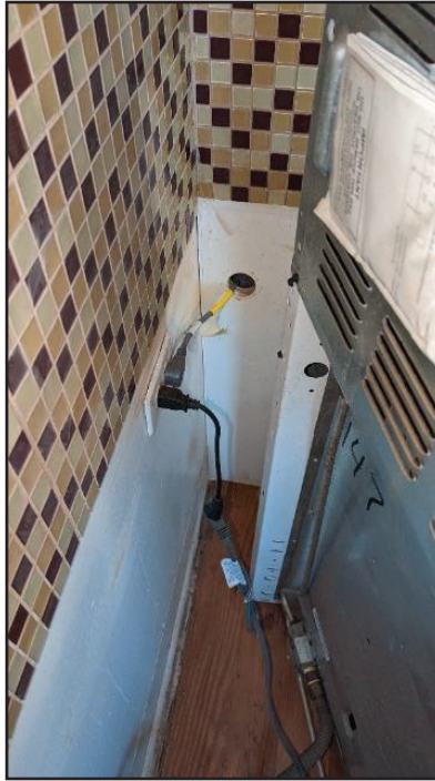
141. Anti-tipping device missing
