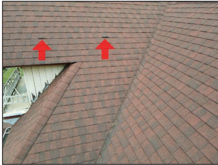
3. Missing, loose or torn
