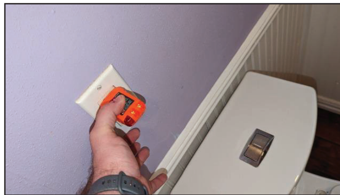
70. No GFCI/GFI (Ground Fault Circuit...)
