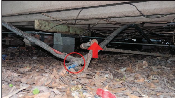
95. Split, damaged, crimped
