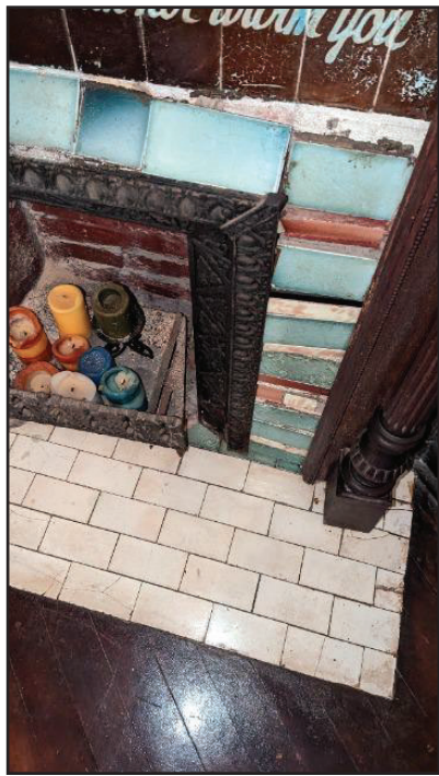
79. Gaps or cracks
