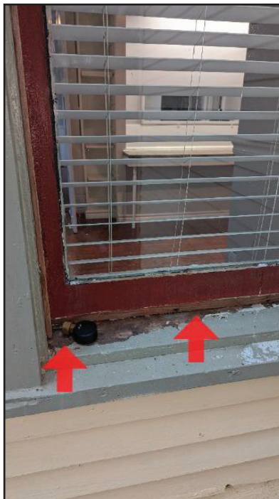
19. Caulking missing, loose or deteriorated
