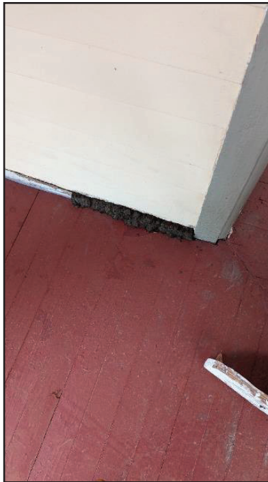
12. Siding - incomplete / missing
