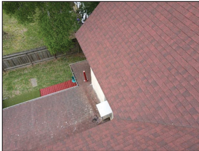
4. Slope too low
