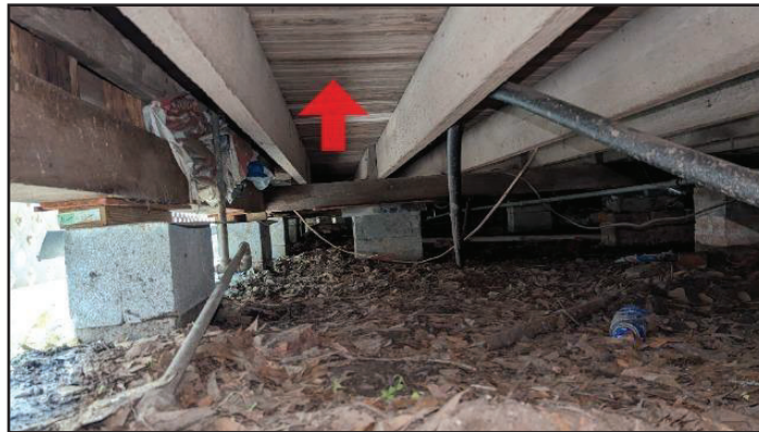
44. No blocking, bracing or bridging
