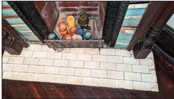
78. Deteriorated, missing or loose masonry or...
