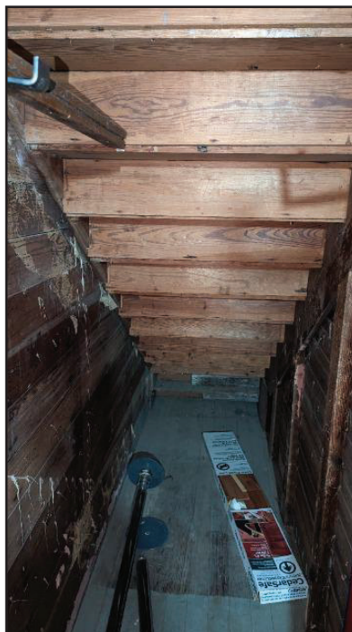
139. Drywall missing or incomplete on underside...
