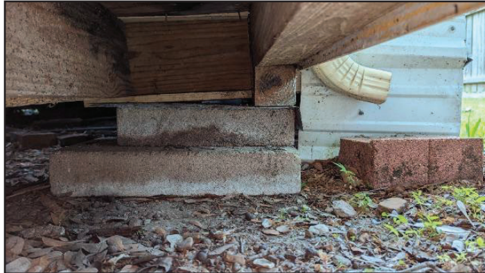
11. Should discharge 6 feet from building
