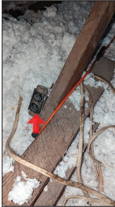
61. Cover loose or missing
