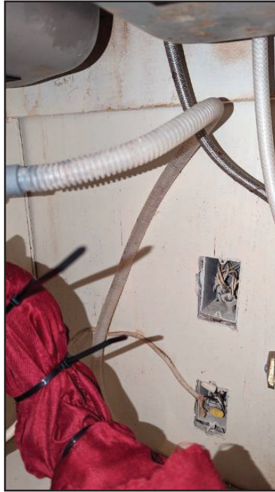
144. Backflow prevention high loop missing
