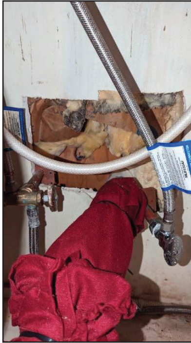
137. Pieces missing or loose
