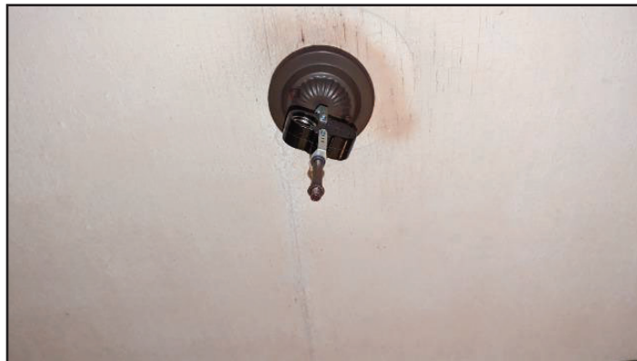
74. Exposed to mechanical damage (No cage or...
