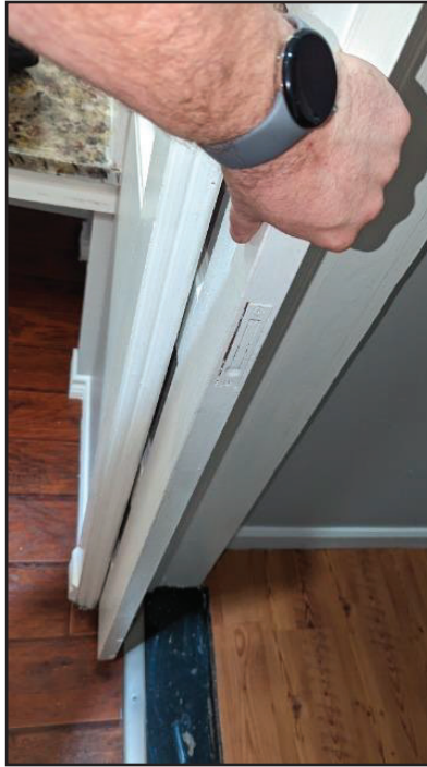
135. Does not latch properly
