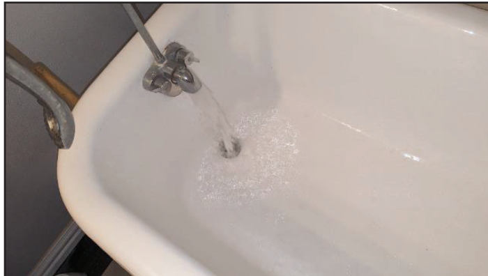
103. Drain stop ineffective
