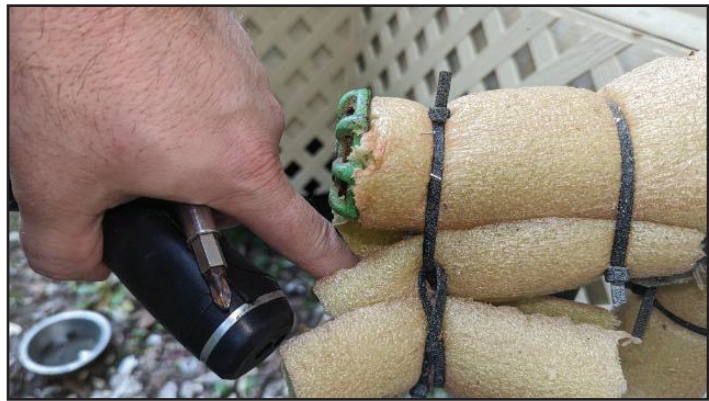
99. Backflow prevention missing
