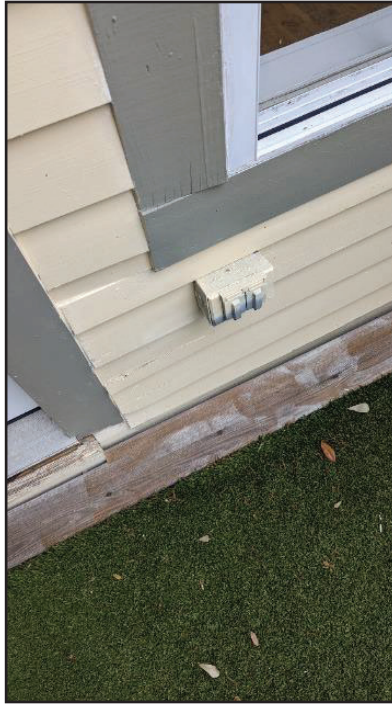
68. GFCI/GFI needed (Ground Fault Circuit...
