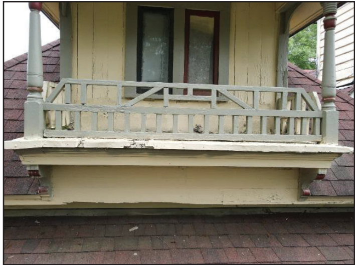
14. Paint or stain - deteriorated / missing
