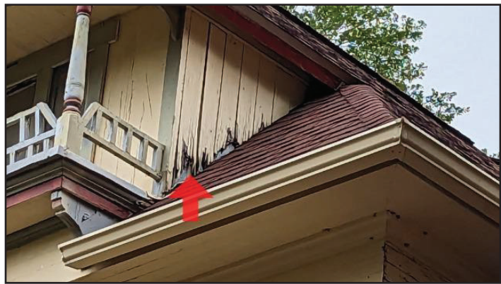
7. Siding not cut back
