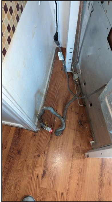
98. No drip leg (sediment trap, dirt pocket)
