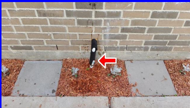
Main water shutoff
