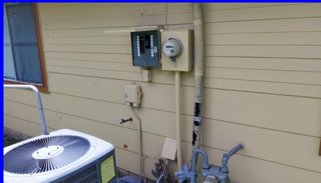
Underground service and meter
