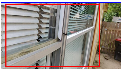
H. Item 1 (Picture) Most plastic dividers were damaged or missing
