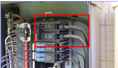
A. Item 5 (Picture) Electrical panel
