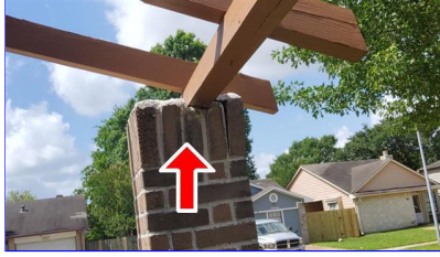
K. Item 2 (Picture) Beam has rolled
