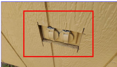
E. Item 17 (Picture) Left side
