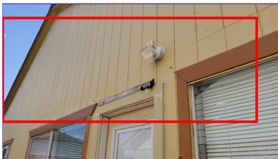
E. Item 19 (Picture) No Z-Flashing installed at horizontal seams
