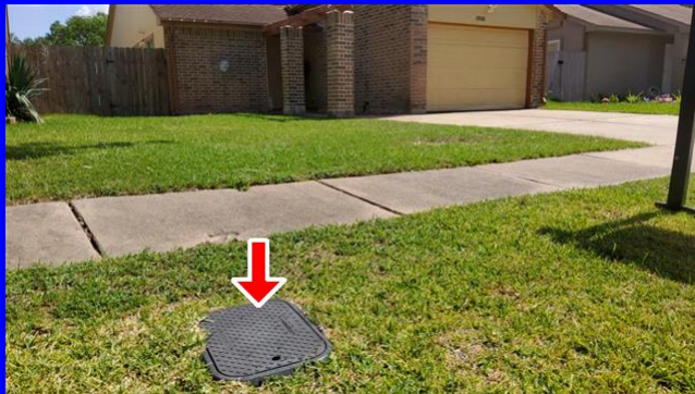
Water meter located in front yard
