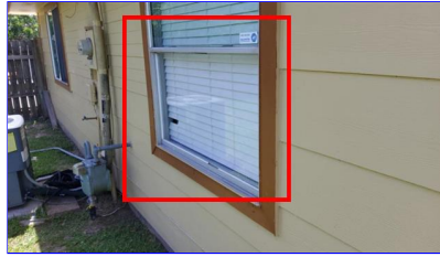
H. Item 6 (Picture) Rear, 1 missing
