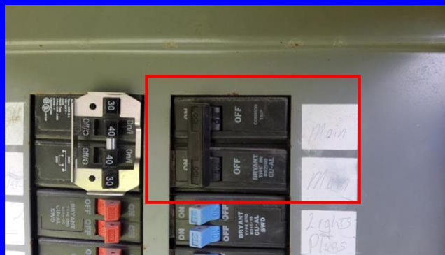
100 amp main disconnect
