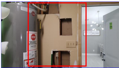
D. Item 2 (Picture) Wall at kitchen needs insulation and drywall repairs
