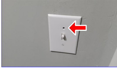
B. Item 16 (Picture) left rear bedroom closet, missing screw
