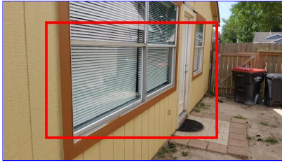
H. Item 5 (Picture) Left side, 3 missing
