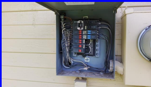
Inside electrical panel
