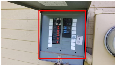
B. Item 4 (Picture) Electrical panel
