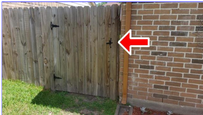
L. Item 6 (Picture) Gate was difficult to operate/latch
