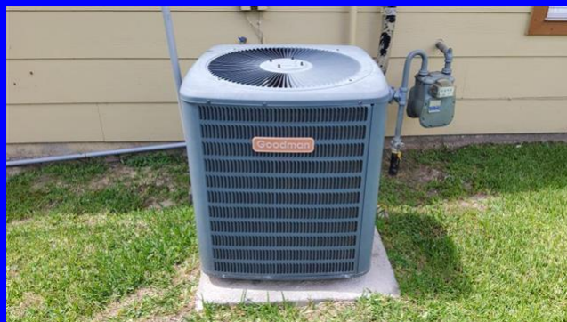
HVAC Outside Condenser
