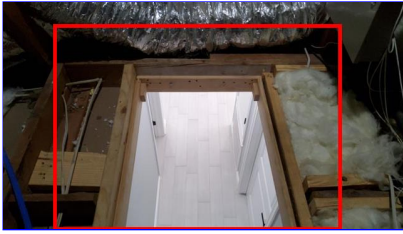
D. Item 6 (Picture) Framing not doubled
