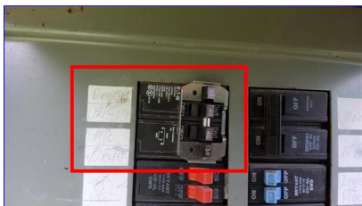
B. Item 5 (Picture) Eaton breakers in Bryant panel
