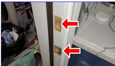
G. Item 3 (Picture) Garage, missing hardware
