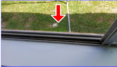
H. Item 7 (Picture) Master bedroom, damaged
