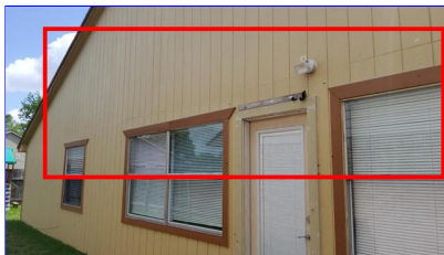
E. Item 18 (Picture) No flashing installed at projecting wood trim
