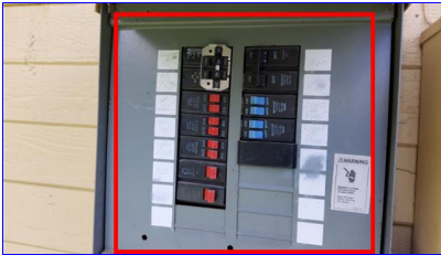
A. Item 4 (Picture) Electrical panel
