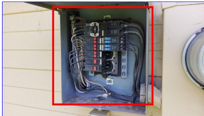
A. Item 6 (Picture) Electrical panel
