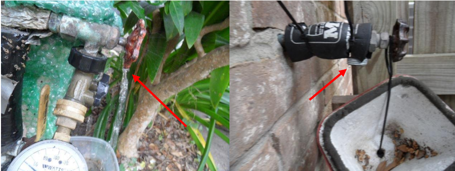
Valve stem leak
