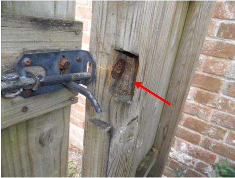
Latch plate missing
