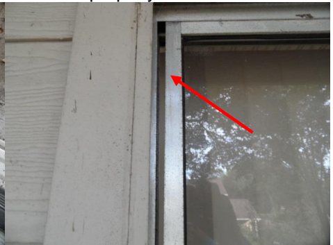
not close and sealed properly
