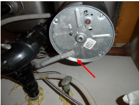
Connector is missing
