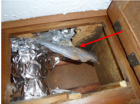
Damaged vent hose
