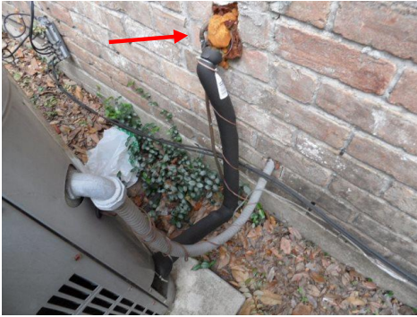
No wall flashing
