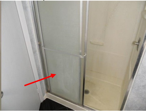
no safety label observed
