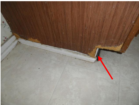
Damaged base cabinet
