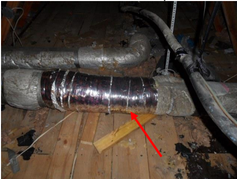
Previous duct repair
