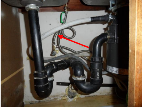
No air gap in drain line
