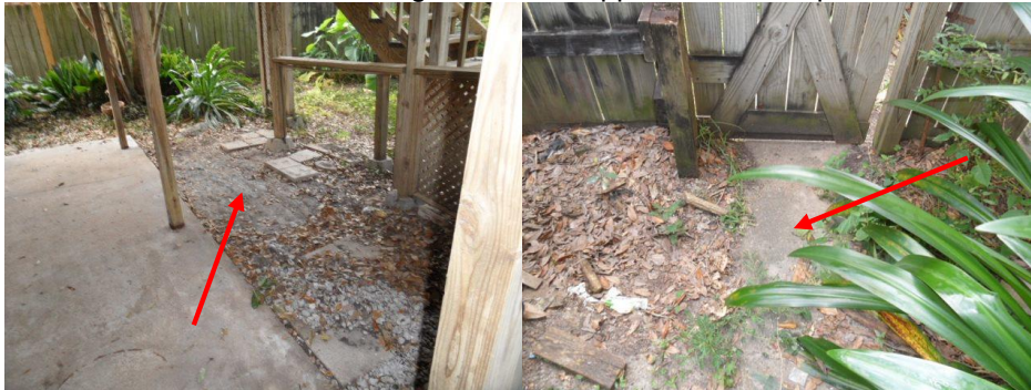
possible ponding areas
