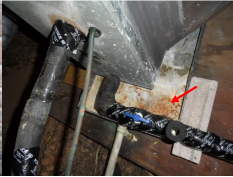
recommend float switch in pan
