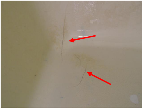
Cracks in shower base
