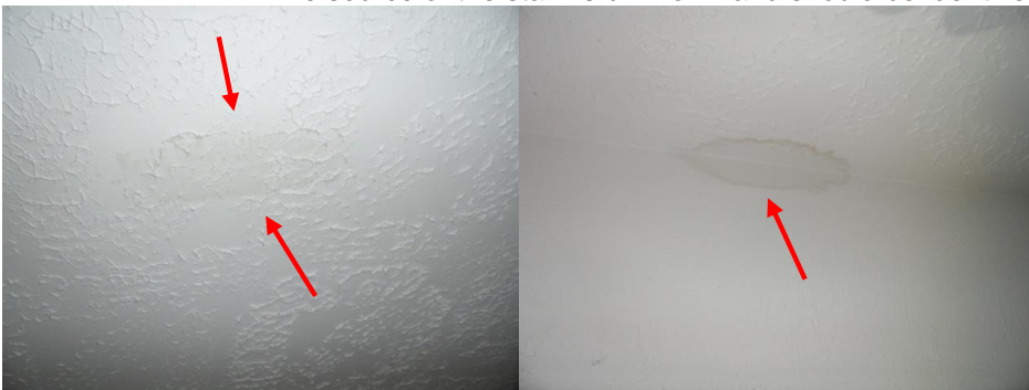
Stain on bedroom ceiling
