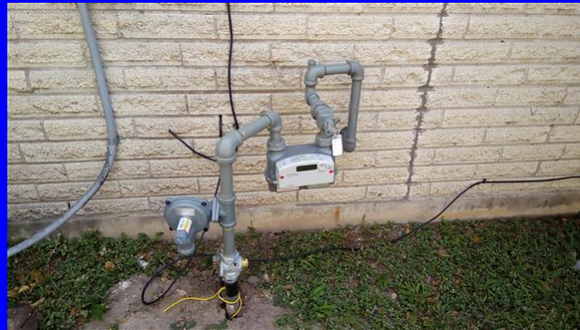
Gas meter located on the right side of the home
