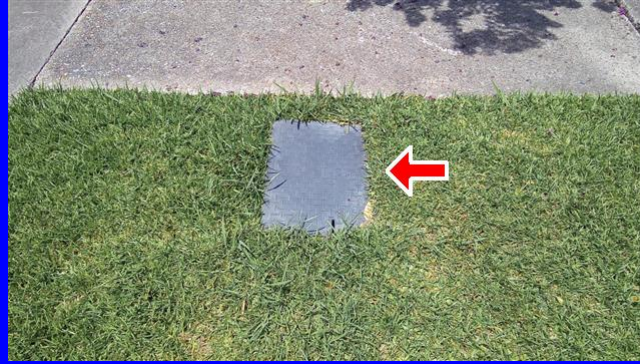
water meter located at the street on the left side
