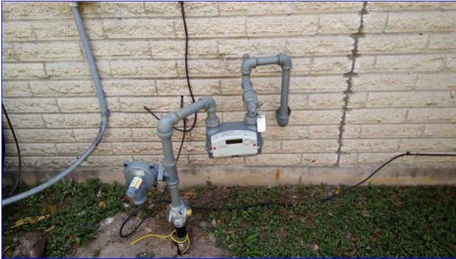
A. Item 1(Picture) at gas meter
