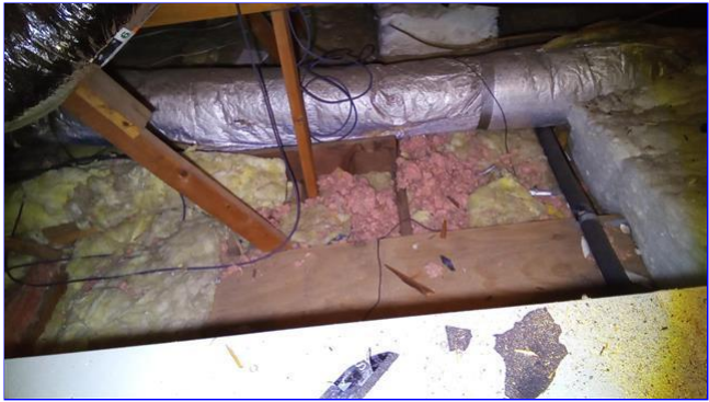
D. Item 2(Picture) additional insulation needed
