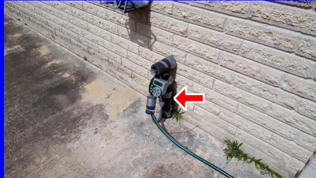
main water shutoff valve located on the left side of the home
