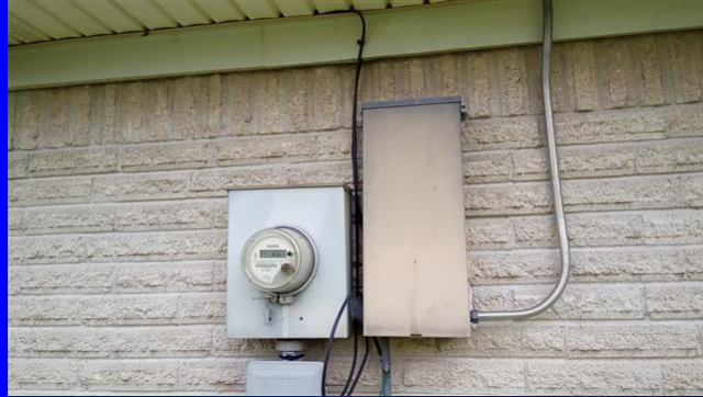
underground electrical service entrance and 100 amp electrical panel located on the rear of the home
