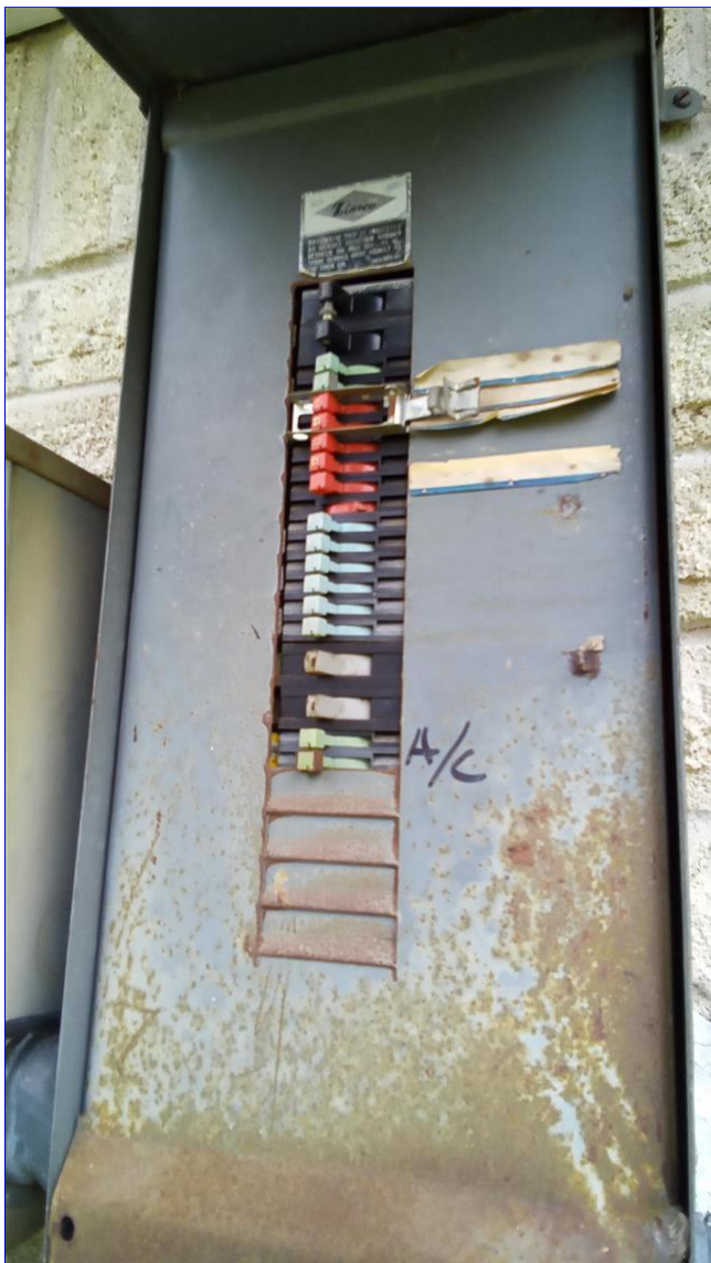
A. Item 5(Picture) no surge protector
