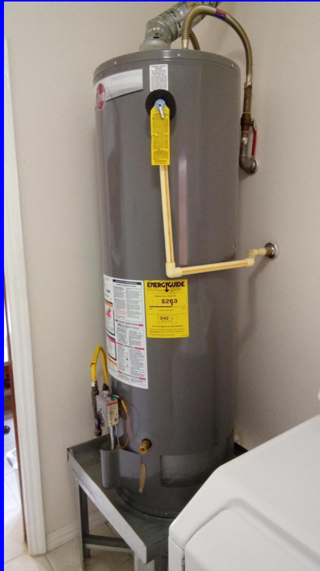
Rheem 40 gallon gas water heater located in the laundry room
