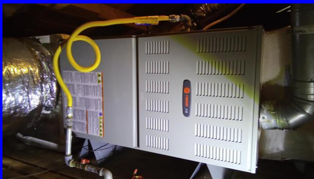
Trane gas furnace located in the attic
