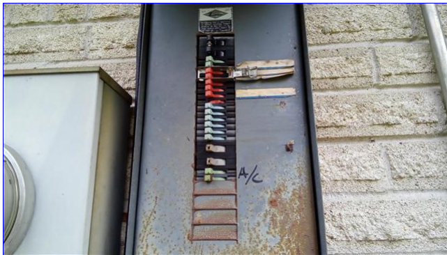
A. Item 4(Picture) clear labeling needed
