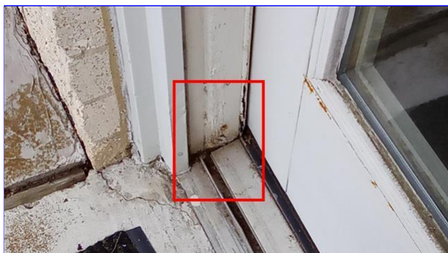
G. Item 3(Picture) right living room rear door at jamb
