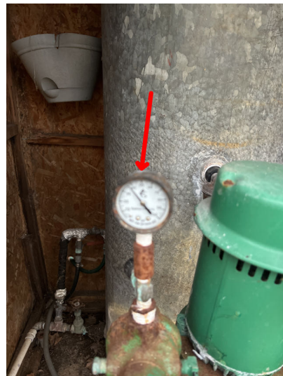
Even though the well is running, and the valves are open, no water pressure reaches the house.
