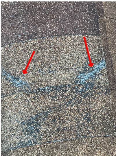
Damaged roof shingles noted, repairs to the roofing are recommended. Damaged or missing roofing material should be repaired. All roof penetrations should be examined and sealed as necessary.
