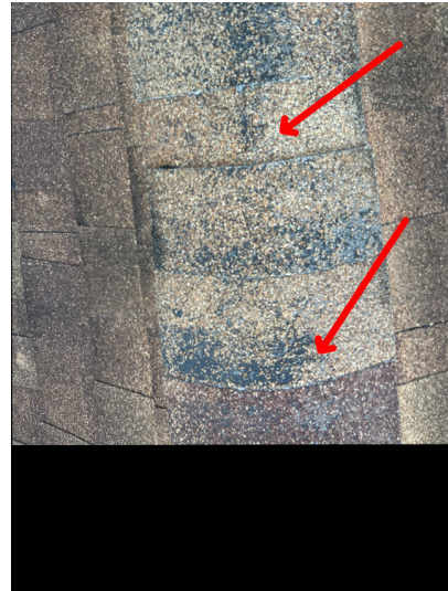
The roofing is nearing the end of its life cycle. Minor repairs are recommended in the short term to maintain the weather tightness of the roof. Damaged or missing roofing material should be repaired. All roof penetrations should be examined and sealed as necessary.
