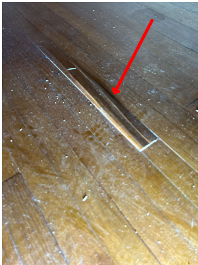
The floor covering is damaged and may be in need of repair or replacement.
