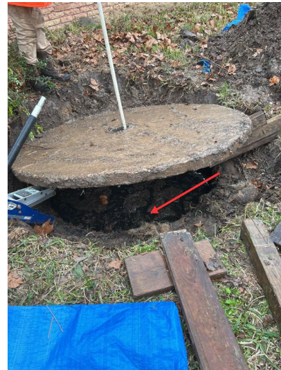
There appears to be debris in the bottom of the septic tank, recommend having it pumped and debris removed .
