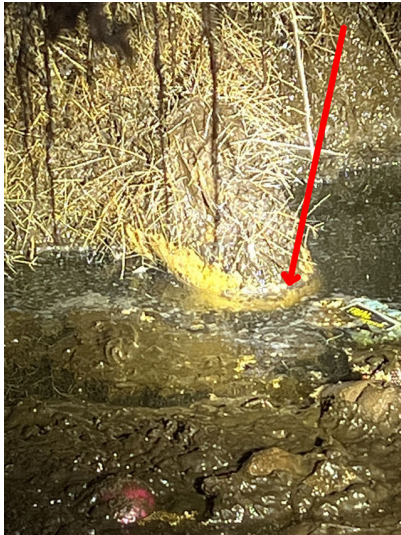
The Liquid level in the tank was noted to be above the drain lines in the tanks into the baffles. Recommendation is to have the tanks pumped out. Septic tank interior was not inspected.
