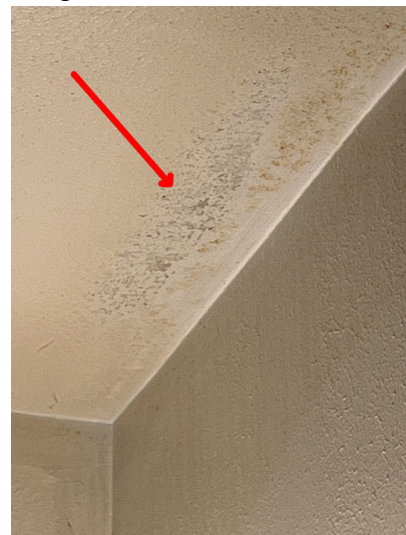
Dark Organic growth was observed on the ceiling of the master bathroom, this condition should be investigated further and re-pairs made if needed.
