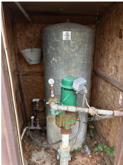
Even though the well is running, and the valves are open, no water pressure reaches the house.
