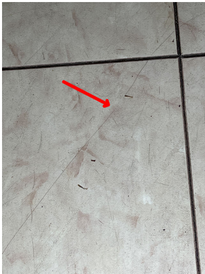
Tile in the was noted to be cracked/damaged.
