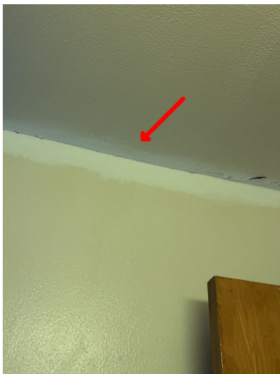
Evidence of repairs was noted on the ceiling of the dining room and the first bathroom.
