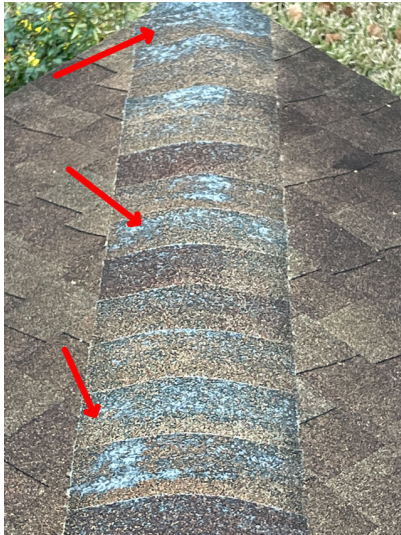
Damaged roof shingles noted, repairs to the roofing are recommended. Damaged or missing roofing material should be repaired. All roof penetrations should be examined and sealed as necessary.
