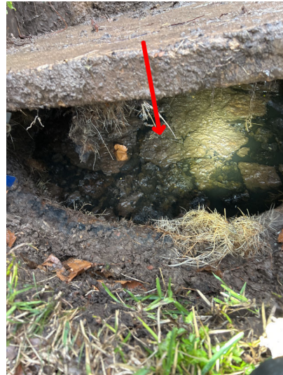
The Liquid level in the tank was noted to be above the drain lines in the tanks into the baffles. Recommendation is to have the tanks pumped out. Septic tank interior was not inspected.
