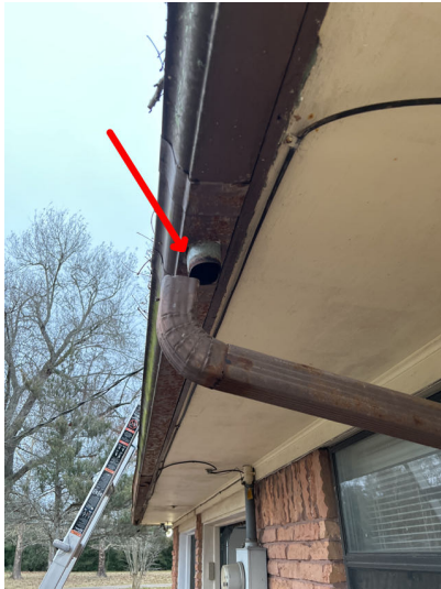
Damaged/leaking gutters noted, repairs may be necessary to help the runoff of water onto or near the structure.
