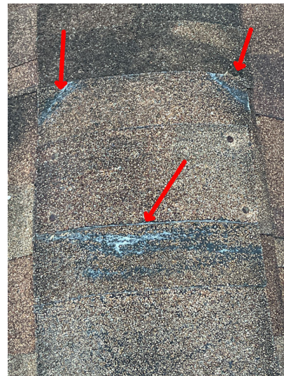
Damaged roof shingles noted, repairs to the roofing are recommended. Damaged or missing roofing material should be repaired. All roof penetrations should be examined and sealed as necessary.
