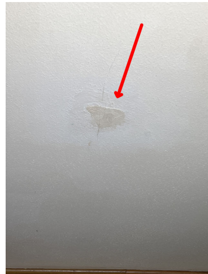
Evidence of repairs was noted on the ceiling of the dining room and the first bathroom.
