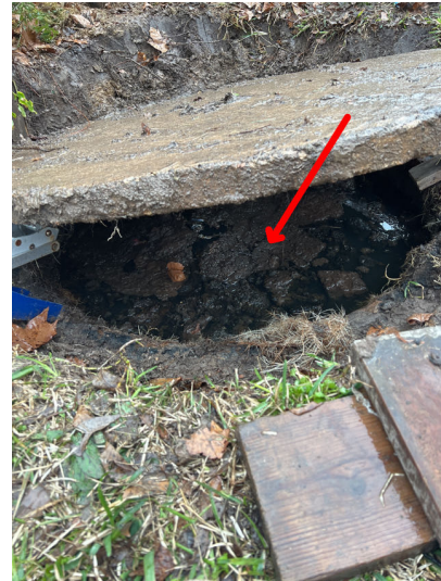
The Liquid level in the tank was noted to be above the drain lines in the tanks into the baffles. Recommendation is to have the tanks pumped out. Septic tank interior was not inspected.
