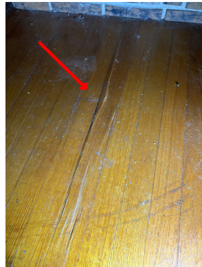
The floor covering is damaged and may be in need of repair or replacement.
