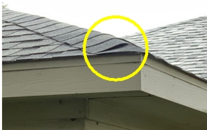
Lifting hip shingle on the left rear corner of the patio.
