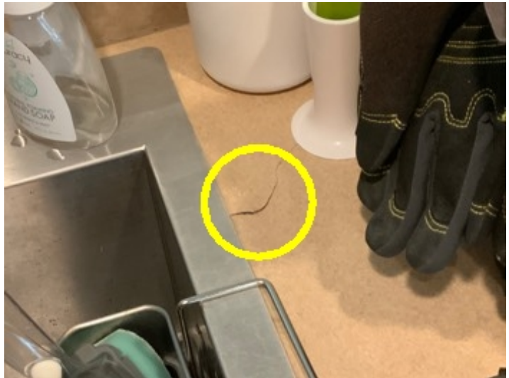
Damaged countertop at the kitchen sink.
