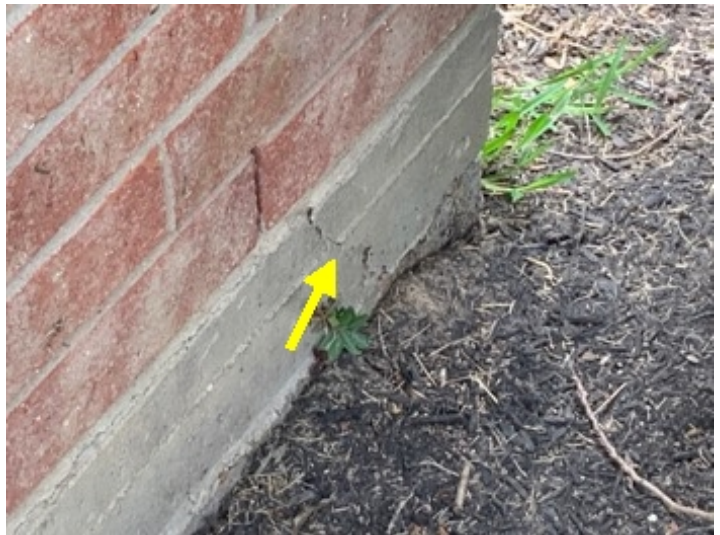
Crack on the right front corner of this home.
