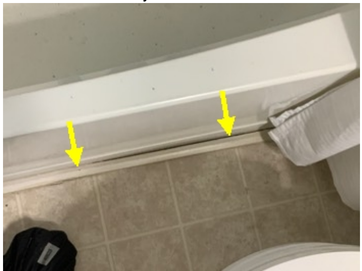
Loose trim at the front of the guest bathtub.
