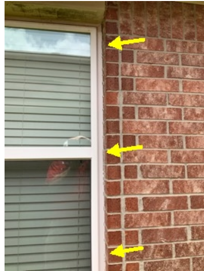
Sealant gaps and uneven gapping at the right rear family room window.
