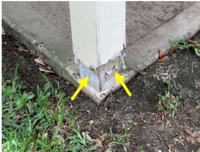
Missing trim and damaged siding on the left rear patio post.
