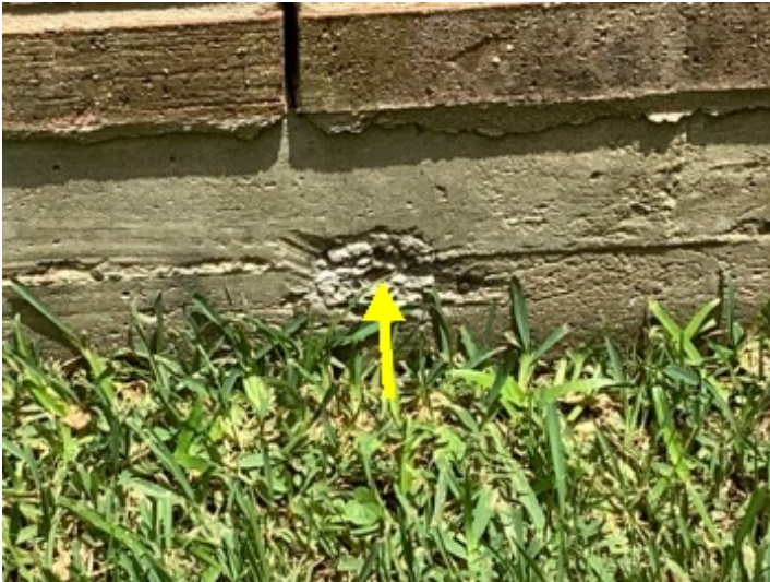
Exposed post tension cable end on the right side of this home.
