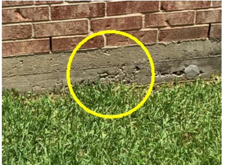
Honeycombing on the right side of this home.
