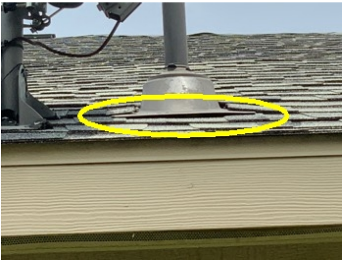
Lifting vent boot flashing on the right side of this home.
