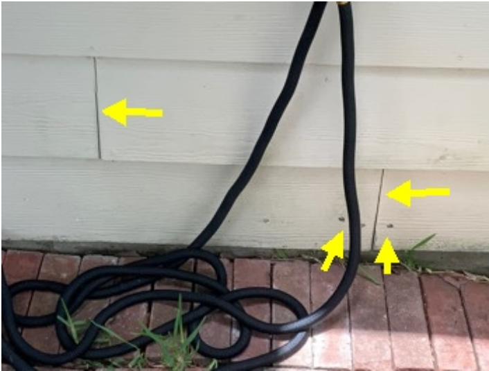
Gaps at the siding seams and exposed nail heads on the rear of this home.
