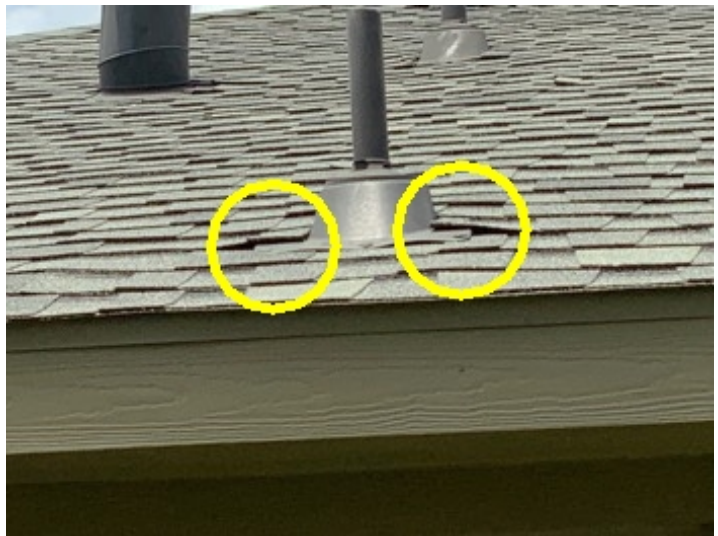
Lifting vent boot flashing and shingles on the rear of this home.
