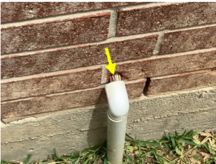
Gap around the sprinkler cable conduit on the right side of this home.
