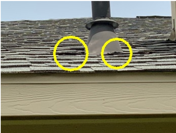
Lifting combustion exhaust vent flashing on the right side of this home.
