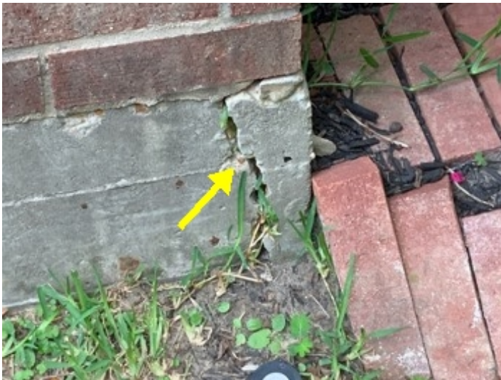
Corner pop on the left front corner of this home.
