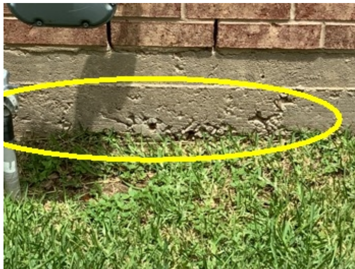
More honeycombing on the right side of this home.
