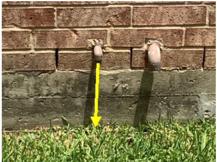
TPR valve drain pipe terminates to far above grade on the right side of this home.
