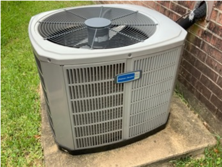
American Standard condensing unit on the left side of this home.
