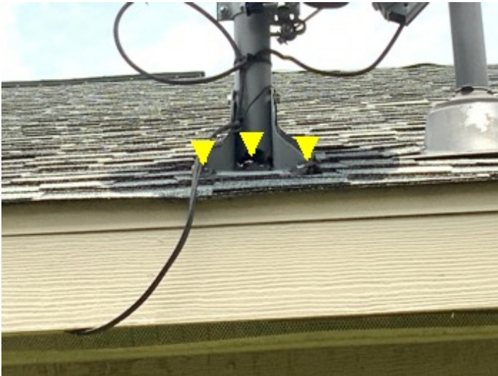
Exposed bolt heads at the satellite dish mount.
