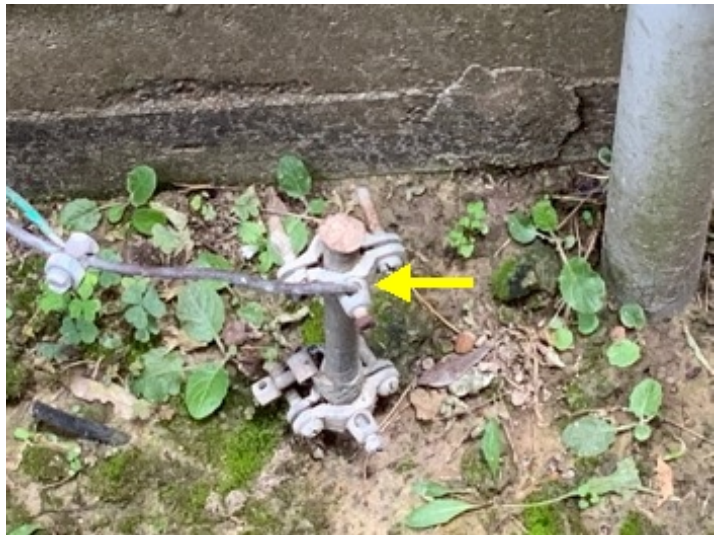
Pipe clamp on the ground rod.
