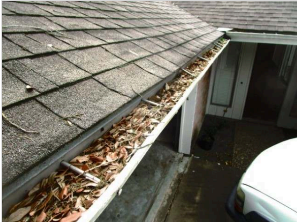
Debris in gutters
