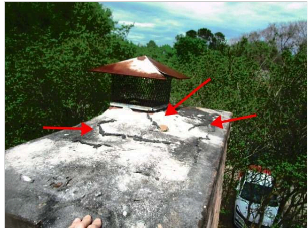
Indications of repair - Chimney crown
