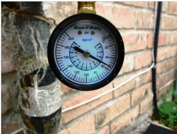
Water pressure reading
