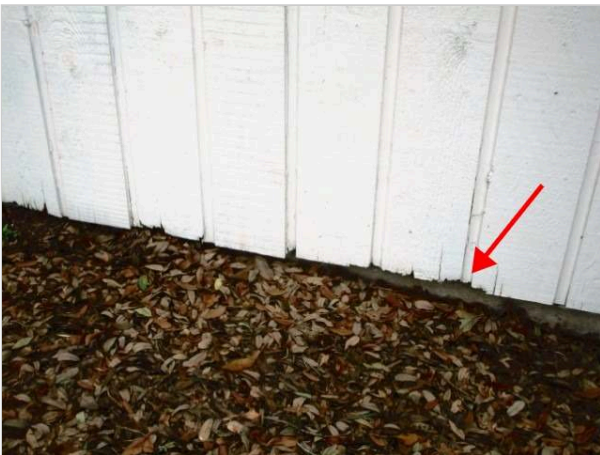
Wood damage - front wall of the garage
