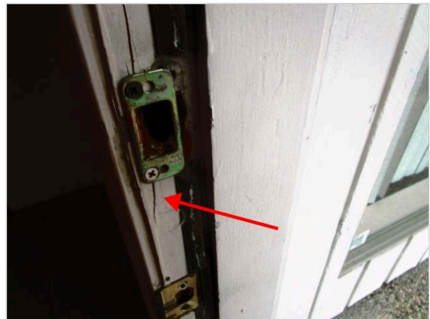
Crack in door frame - exterior door from kitchenette
