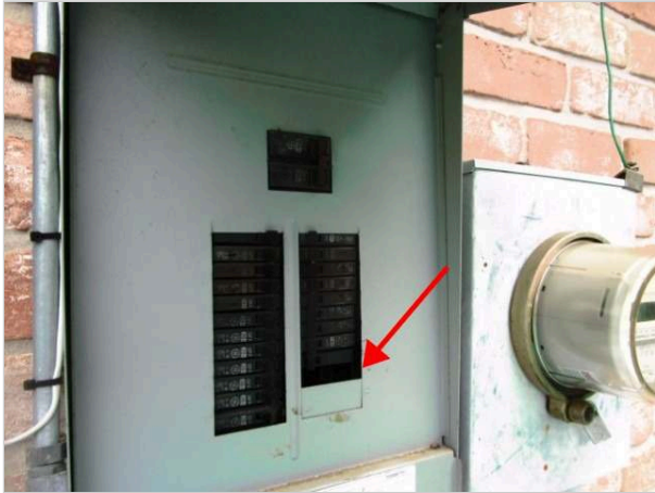
Main Service Panel / Knockout missing
