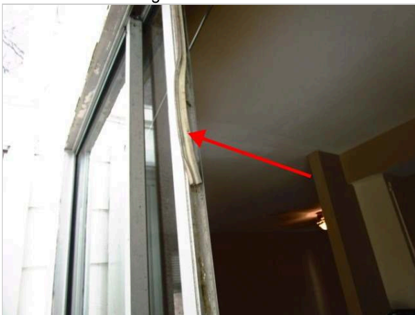
Weatherstripping - damaged / missing at the sliding glass door to right porch
