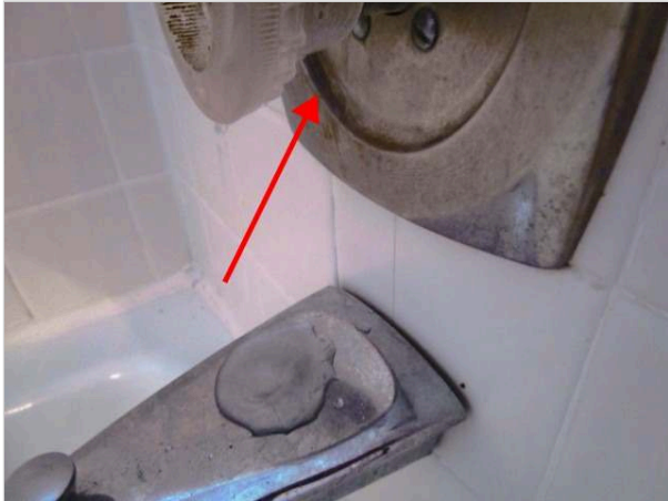
Control knob leak - hallway bathroom bathtub
