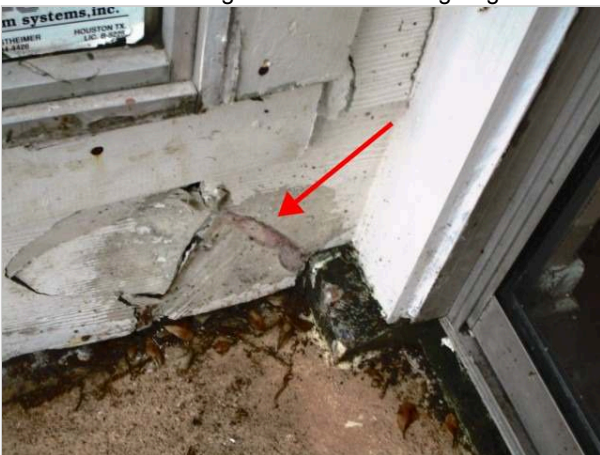
Damage - rear wall behind living room
