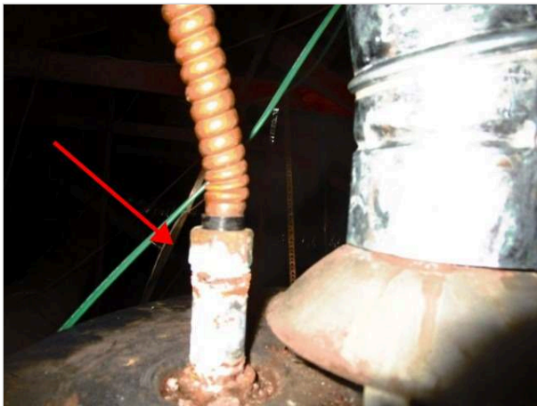
Rusted / corroded connection
