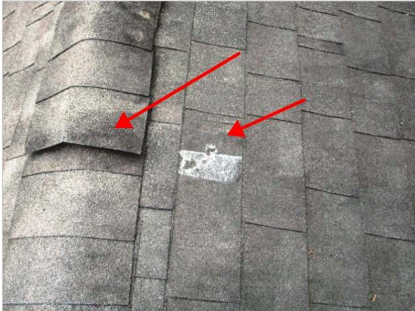
Damaged shingles - over master bedroom
