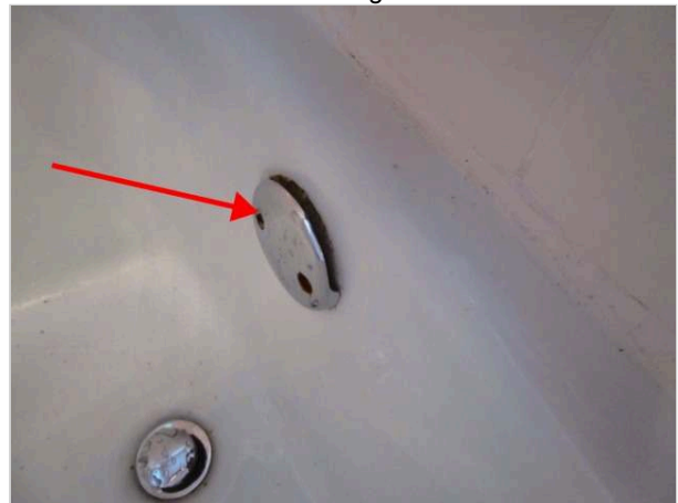
Overflow plate upside down
