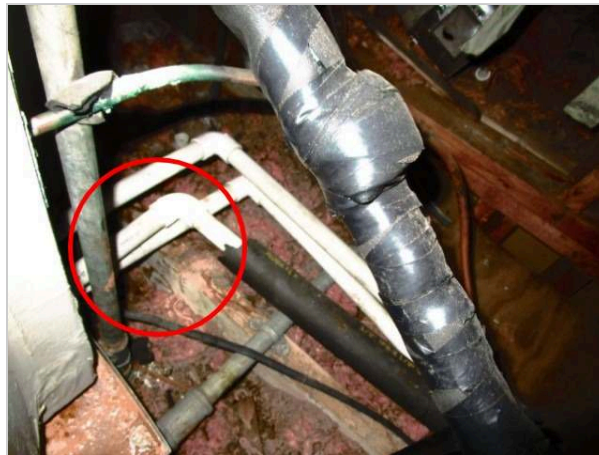
Needs insulation on the primary line at the evaporator coil
