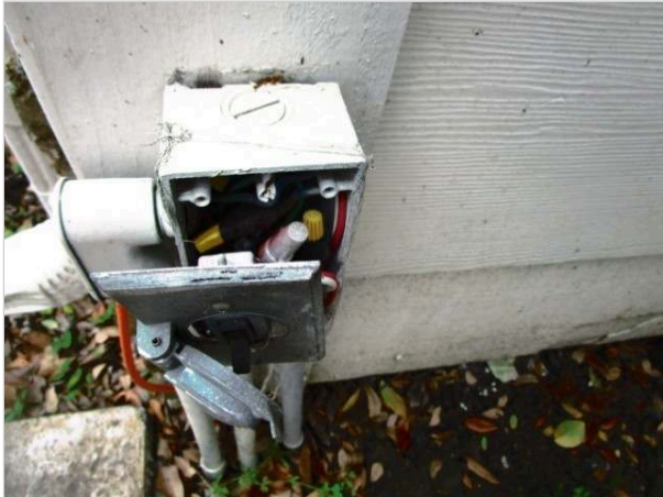
Front plate off light switch (splices exposed)
