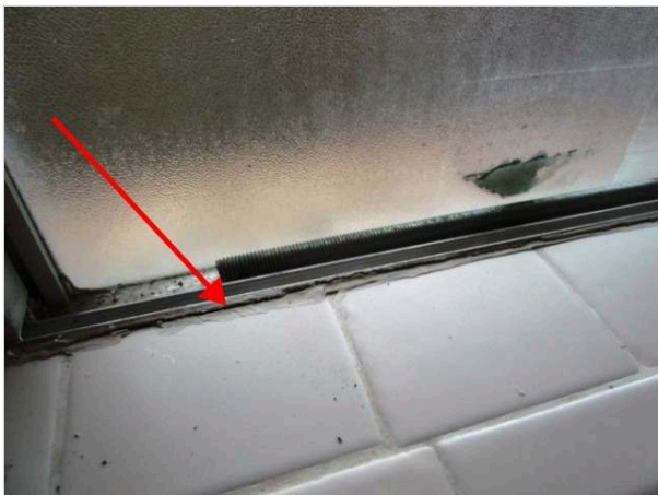
Gap between tile and window frame
