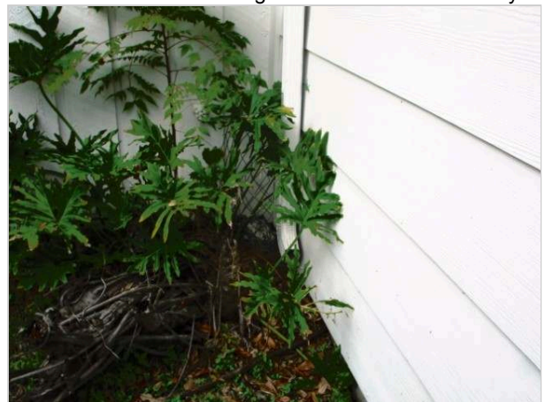
Vegetation in contact with walls
