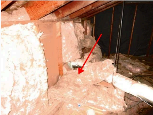
Fallen vertical insulation
