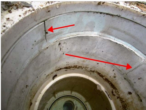
Cracks in skimmer
