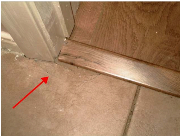
Crack in floor tile in master bathroom
