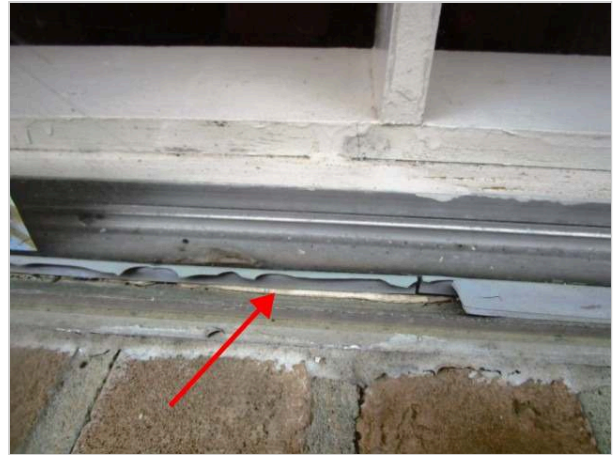
Glazing bead damage - kitchenette window
