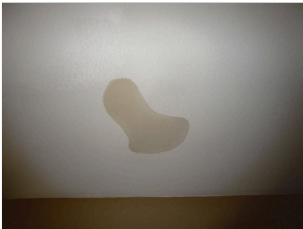
Indication of water penetration - back hallway ceiling
