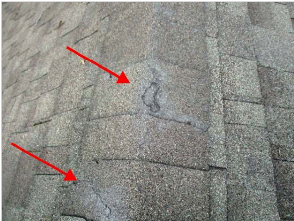
Damaged shingles over garage
