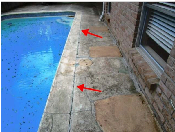
Cracked / shrunken sealant between coping and decking
