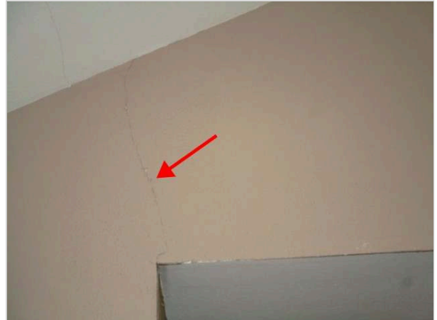
Crack in living room
