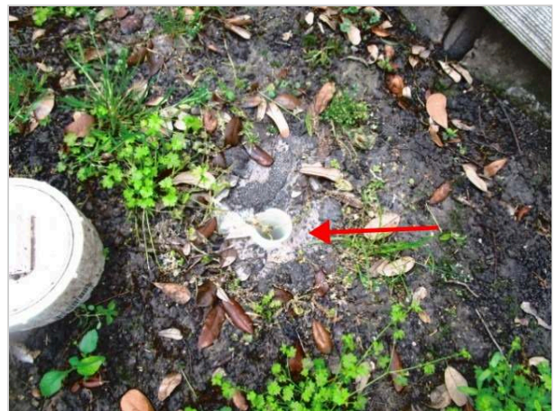
Damage to pipe between pool and equipment
