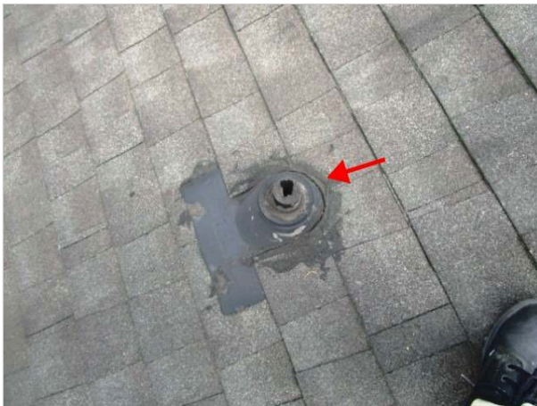
Vent terminating less than 6" above the roof
