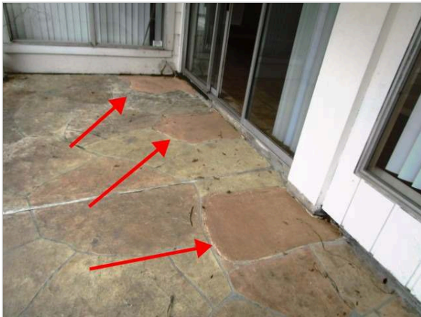
Pier marks - Porch behind living room
