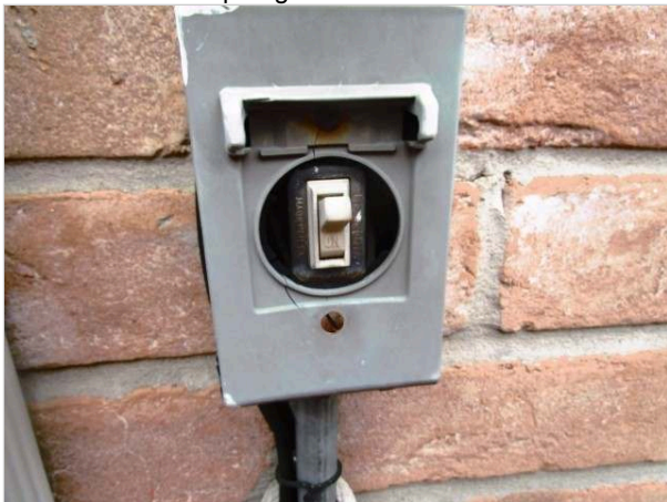
Exterior switch (left wall) missing weather cover
