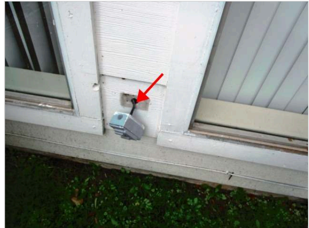
Exterior receptacle not mounted - behind living room
