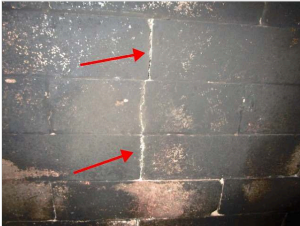
Crack in firebox
