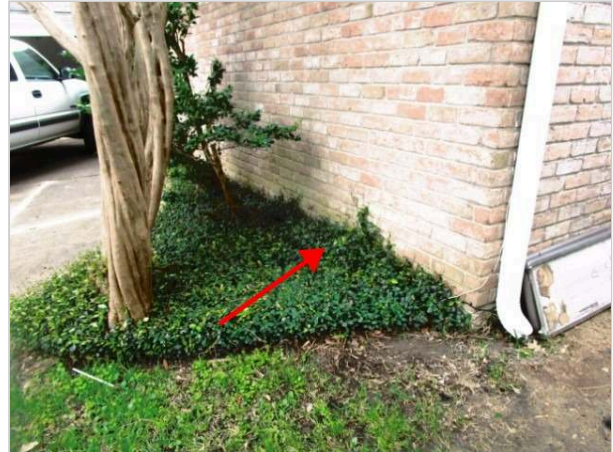
Vegetation against the brick veneer
