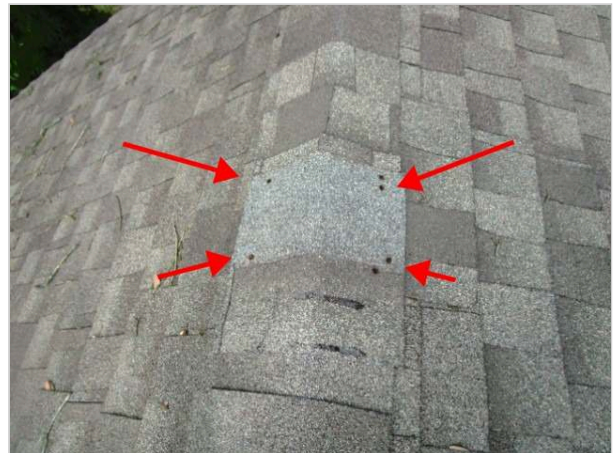
Exposed nails over garage
