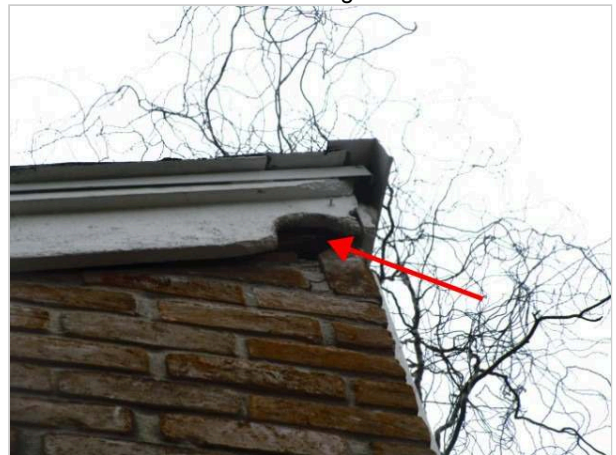
Hole in the brick wall - right side behind the chimney
