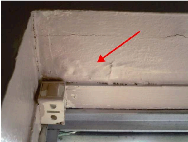
Indication of water penetration - living room center window
