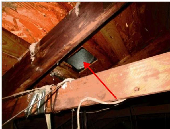
Dryer exhaust termination missing pipe
