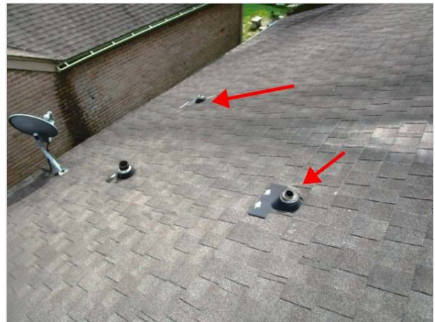
Vents terminating less than 6" above the roof
