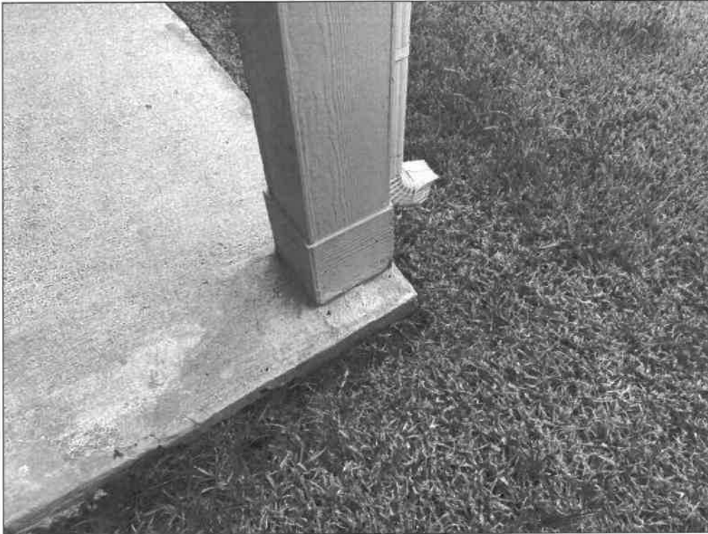
E. Item 10 (Picture) Damaged siding was observed at the bottom of the columns in the backyard.
