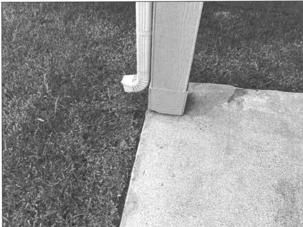
E. Item 11 (Picture) Damaged siding was observed at the bottom of the columns in the backyard.
