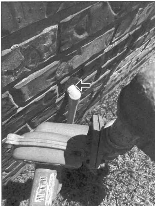
E. Item 5 (Picture) Areas observed where wall penetrations, panels, outlets, and/or fixtures need to be sealed to the wall with an appropriate sealant.
