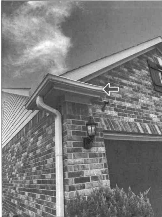
B. Item 7 (Picture) A damaged gutter was observed at the front left corner of the home.
