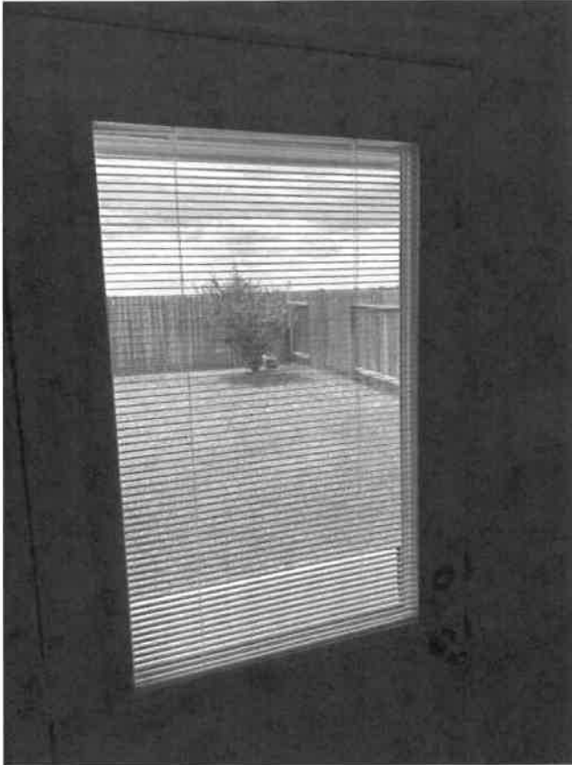
G. Item 2 (Picture) The blinds built into the back door window do not function. Recommend correction.
