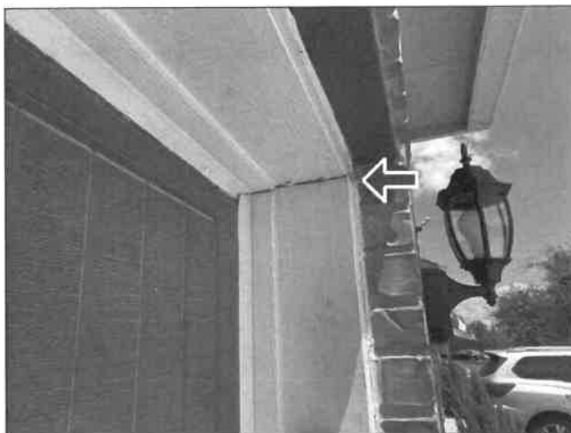
E. Item 3 (Picture) Areas were observed where the brick, siding, and/or trim had gaps that need to be sealed with an appropriate sealant.
