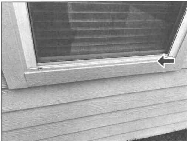
H. Item 1 (Picture) The perimeter sealant, has failed on some windows.
