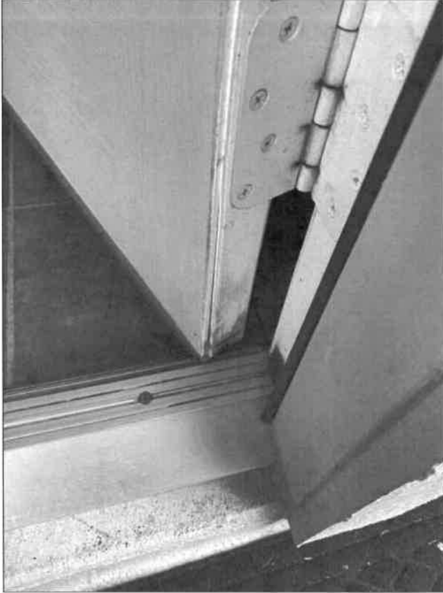
G. Item 1 (Picture) Water damage was observed at the bottom of the inside of the back door.
