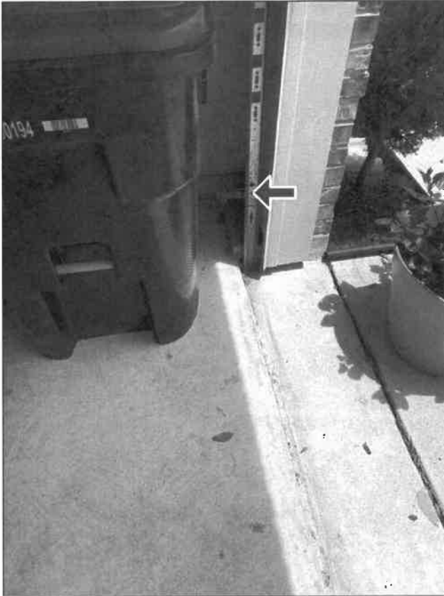
G. Item 1 (Picture) The door sensors appear mounted too high. Maximum height for sensors is generally no greater than 8 inches above the floor. Check the manufacturers' installation instructions for correct maximum height of sensors.
