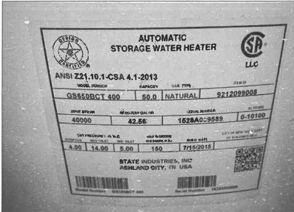
C. Item 1 (Picture) Water heater service tag. Manufacture date 2015.
