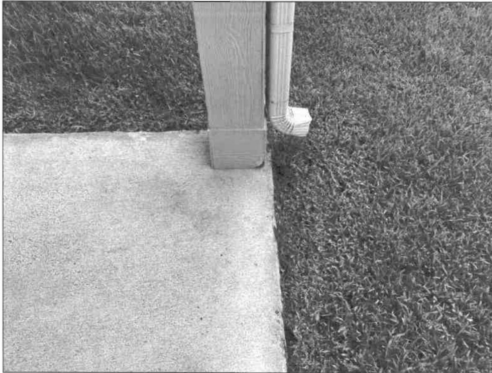
E. Item 12 (Picture) Damaged siding was observed at the bottom of the columns in the backyard.
