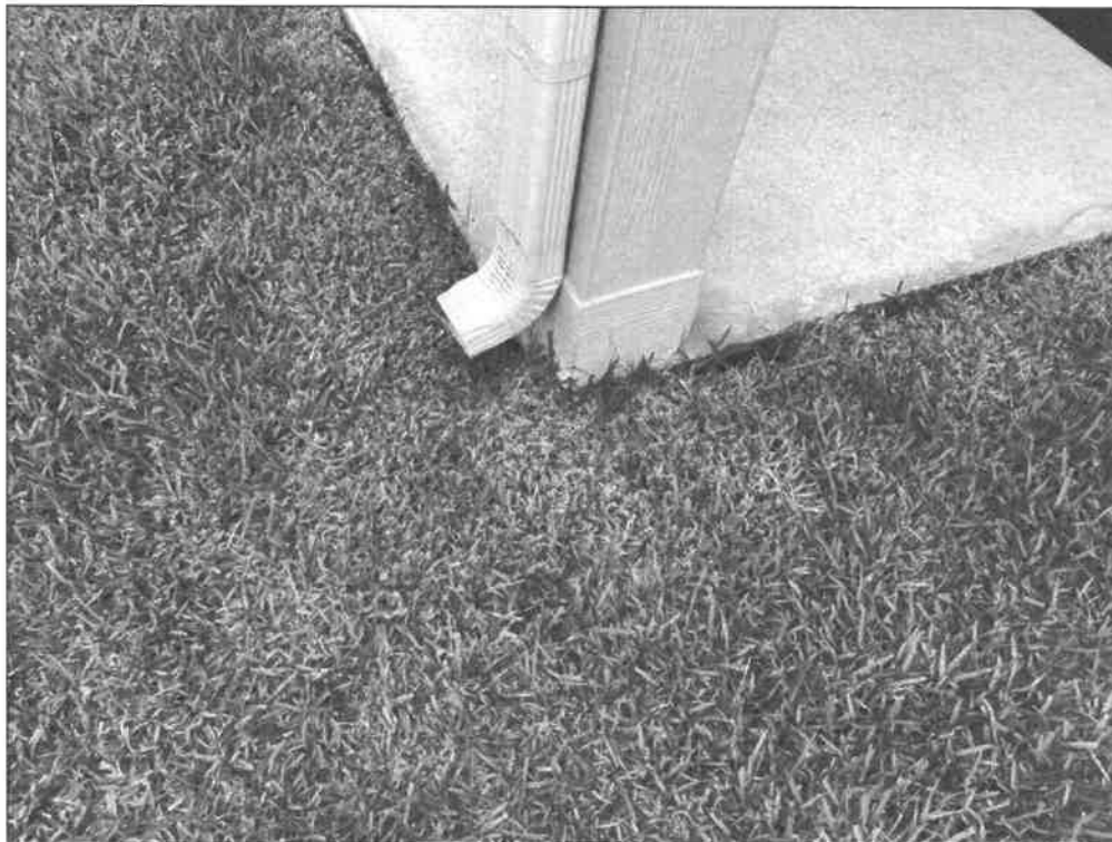
E. Item 13 (Picture) Damaged siding was observed at the bottom of the columns in the backyard.
