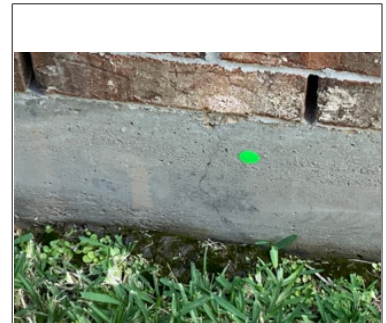
Shrinkage crack on right side
