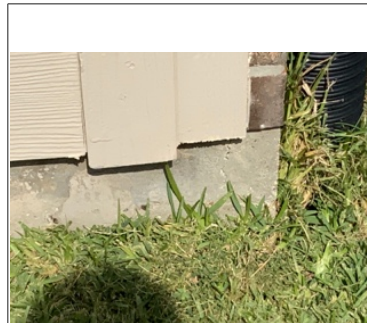
Broken left rear corner
