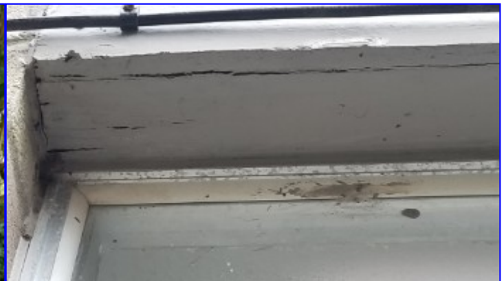
Water damage was observed above the left window on the left wall of the breakfast area. Repairs should be undertaken to prevent further damage.
