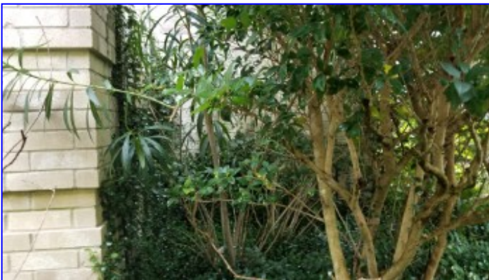
Vegetation is in contact with exterior walls. It is recommended vegetation be cut back at least 6 inches from exterior walls.
