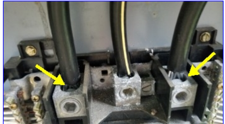
Antioxidant mastic is not applied to the aluminum main service feed wires to prevent oxidation. Repairs recommended.
