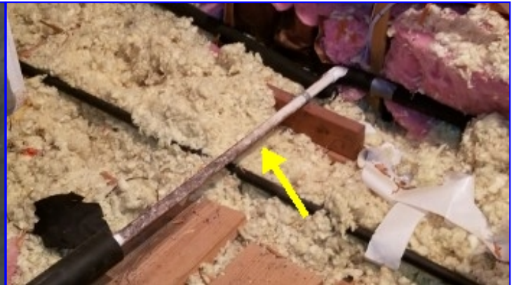
Missing insulation on primary condensate lines should be repaired/replaced to prevent moisture damage to the adjacent materials.
