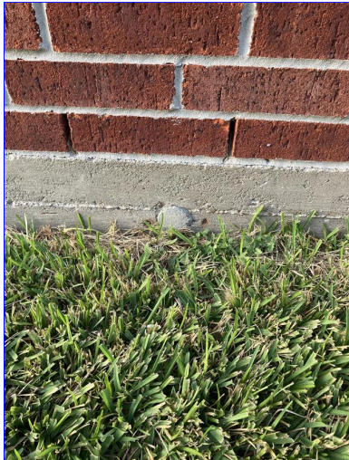
A. Item 1(Picture) Post tension anchor point
