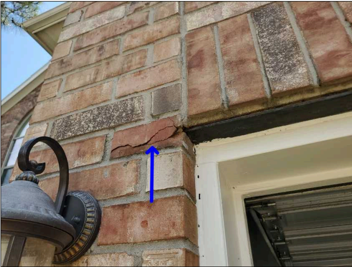
Damaged/cracked brickwork noted. Mainly at - front
