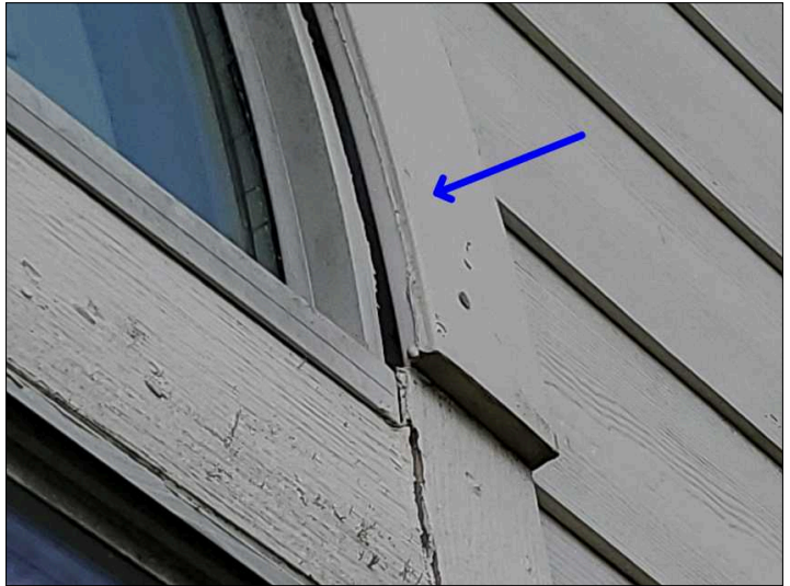
- There is loose trim on the home, recommend securing to help prevent future damage and water penetration. Mainly at - rear
