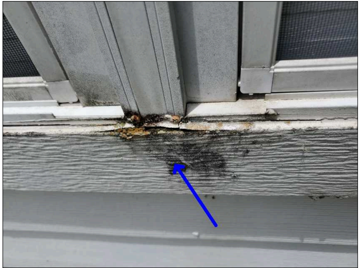
- Deterioration was noted at the trim, recommend replacing all deteriorated trim. Unable to determine the condition of the underlying materials. Mainly at - rear
