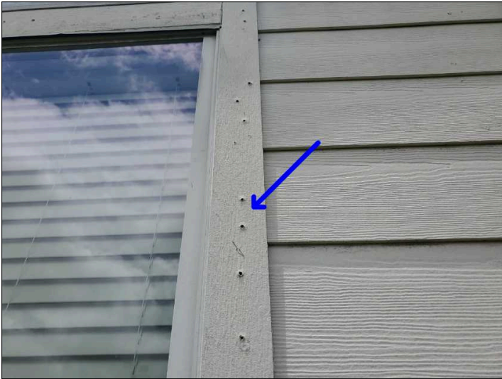
- Seal all gaps and holes in brick or siding to help prevent moisture intrusion. Mainly at - rear
