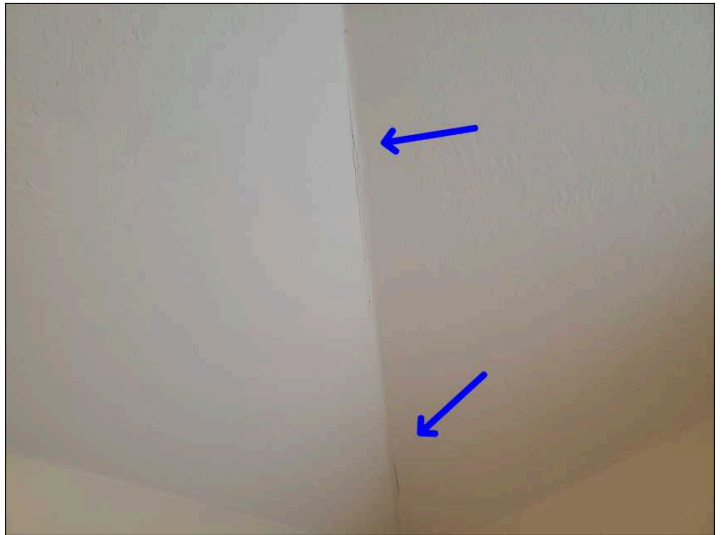
- Settlement cracks were noted at the tape joint in the drywall. Mainly at - upstairs rear right bedroom
