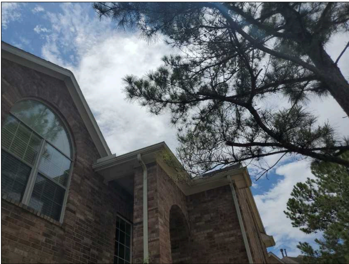
- Tree limbs should be kept trimmed at least 5' from roof to help prevent damage to the roof during windy conditions.
