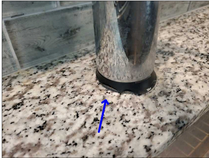
Faucet base damaged. Mainly at - kitchen
