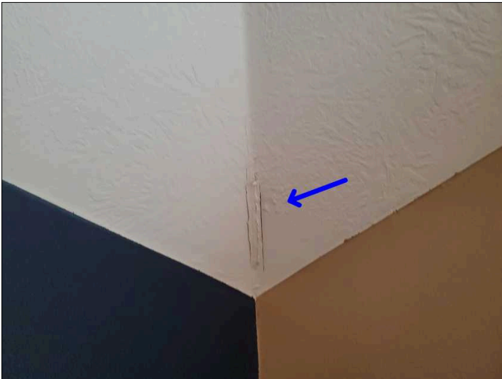
- Settlement cracks were noted at the tape joint in the drywall. Mainly at - upstairs family room
