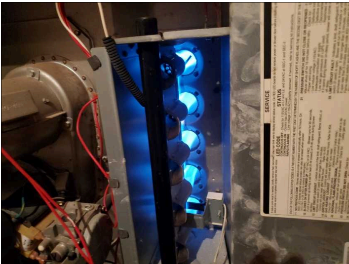
Overview of furnace burner compartment.
