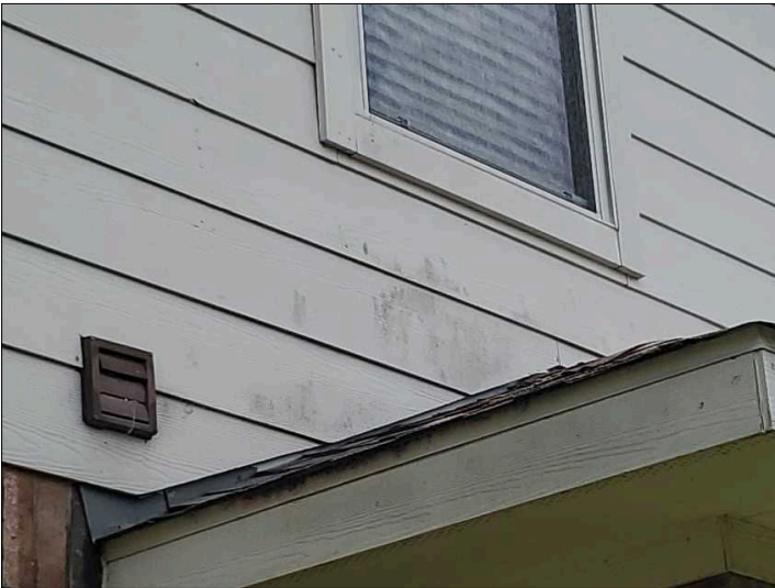
- There are signs of growth on exterior brickwork/siding, recommend cleaning to help prevent deterioration.
