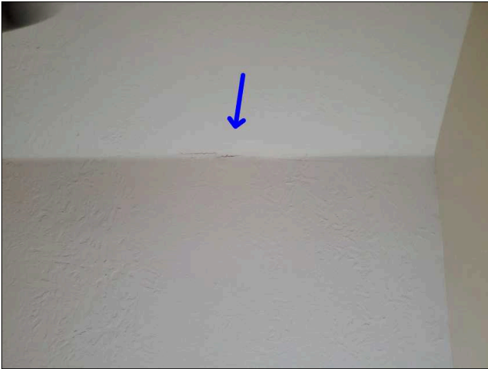
- Settlement cracks were noted at the tape joint in the drywall. Mainly at - upstairs rear right bedroom
