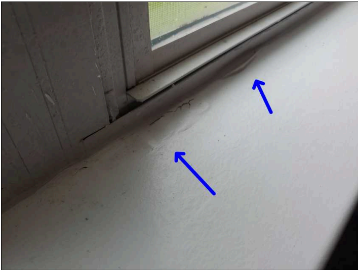
- Paint is cracked and peeling, recommend repairs to help prevent deterioration. Mainly at - master bedroom window sill
