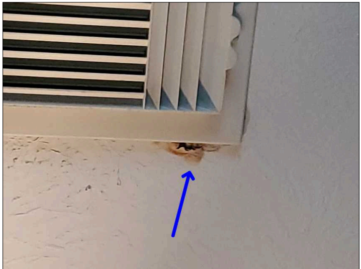
- There are indications of water penetration to the ceiling evident mainly by deterioration. Unable to determine condition of the underlying materials. Mainly at - upstairs family room
