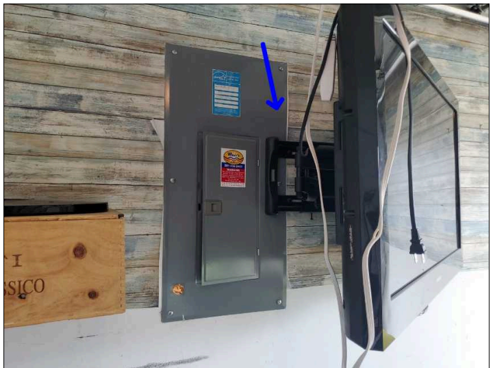
- There was no access to the electrical panel.
