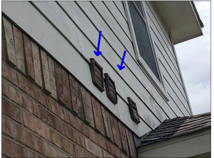
- Seal all vents at wall connection to help prevent water penetration into walls. It is a good idea to leave a small opening at the bottom to allow any water penetrating to escape.
