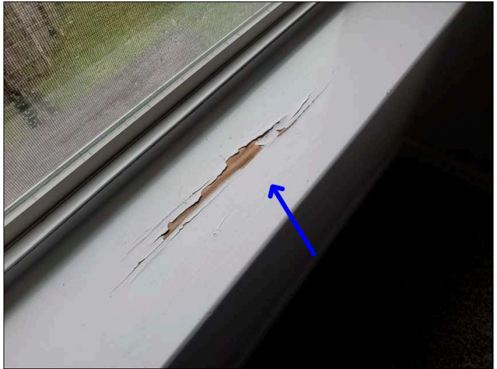
- Paint is cracked and peeling, recommend repairs to help prevent deterioration. Mainly at - upstairs rear right bedroom window sill
