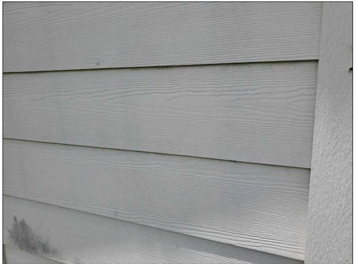
- Paint is chalking meaning it is losing its protection values, recommend repainting.
