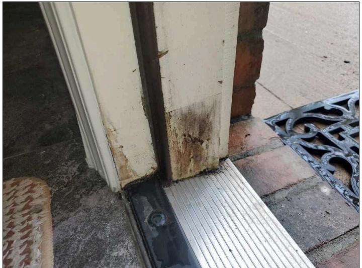
- Deterioration was noted at the trim, recommend replacing all deteriorated trim. Unable to determine the condition of the underlying materials. Mainly at - rear door
