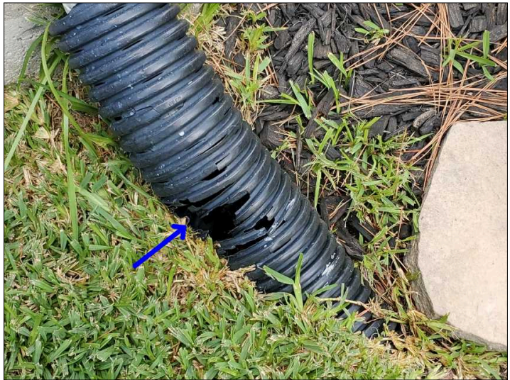
Gutter extensions damaged. Mainly at - front left
