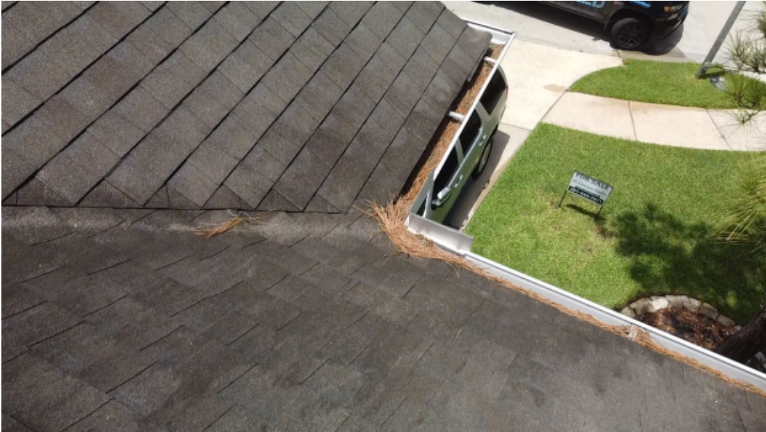
Debris in Valley and in Gutter.
