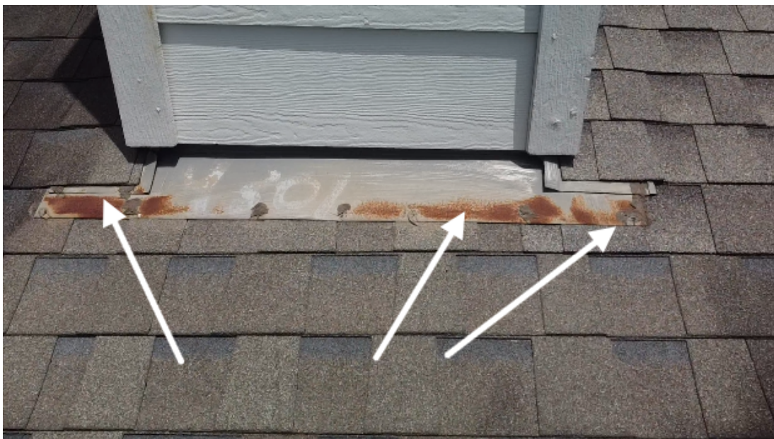
Flashing has some surface rust and some nail heads are exposed.
