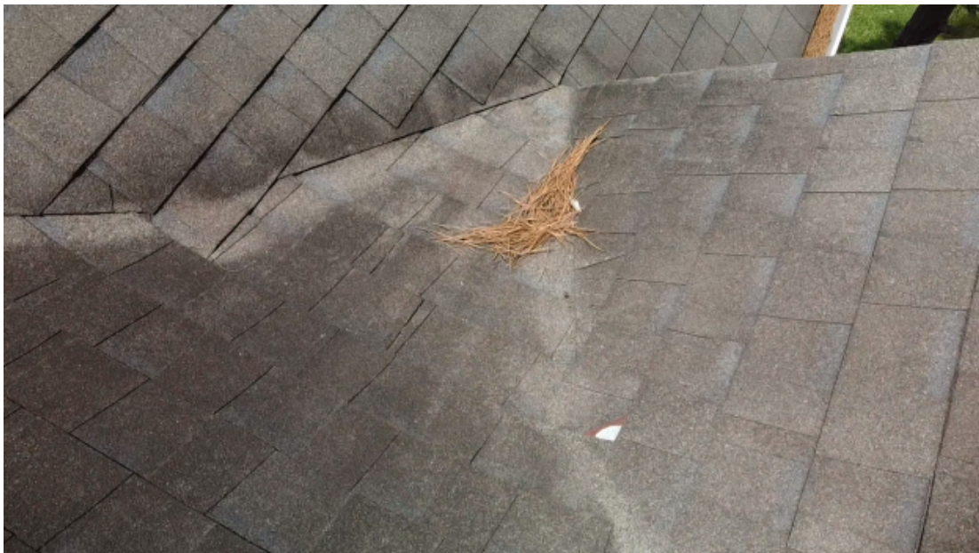
Debris in Valley
