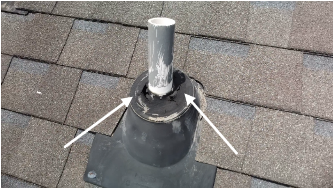
Damaged pipe boot
