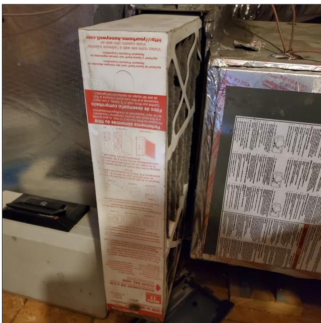
C. Item 2(Picture) Overview of air filter.
