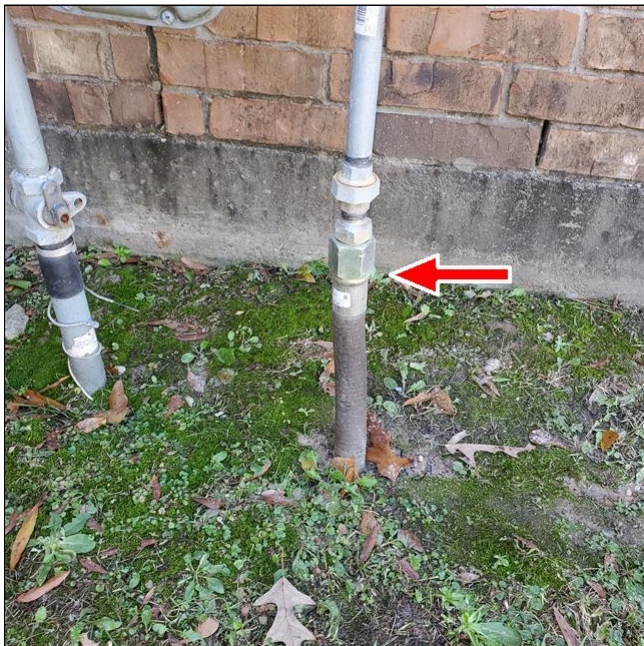
H. Item 1(Picture) Gas smell was present in this area.
