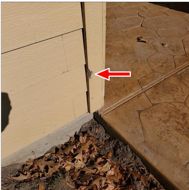
E. Item 2(Picture) Need to seal and paint siding trim to protect from deterioration.
