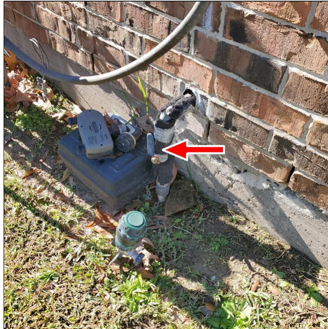
Main water valve is at the left side.
