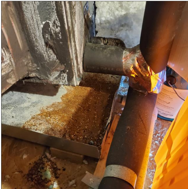
B. Item 3(Picture) Photo of drain pan.
