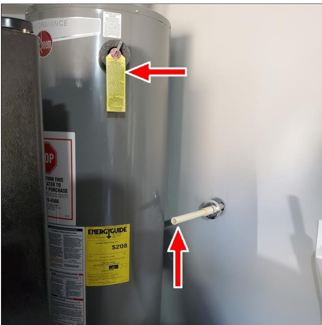
C. Item 3(Picture) PVC pipe should be connected to the TPR valve.
