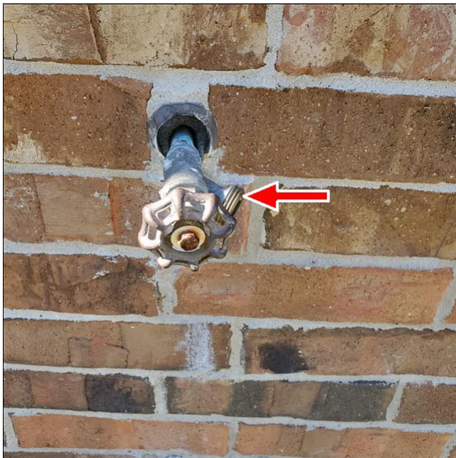
A. Item 1(Picture) Hose bib faces to the side.
