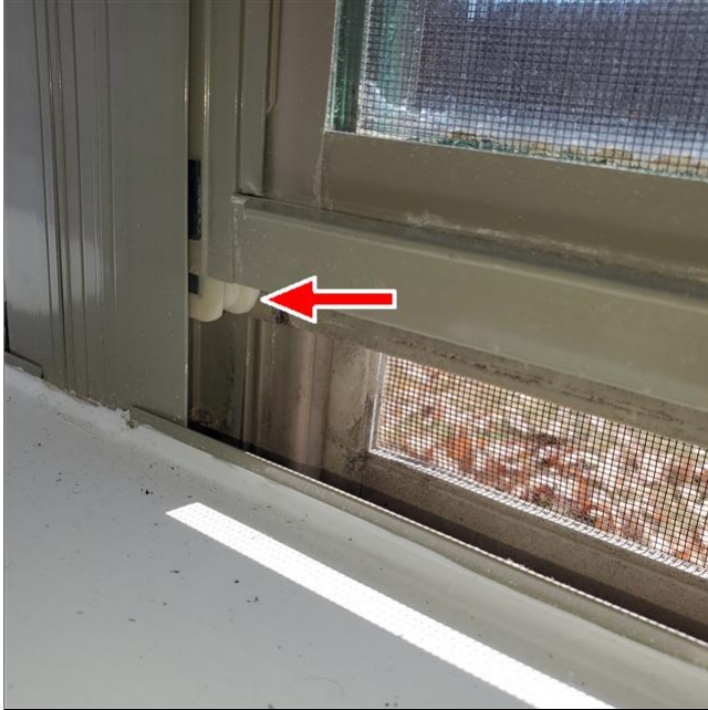
H. Item 1(Picture) Photo shows bottom of rod is visible.
