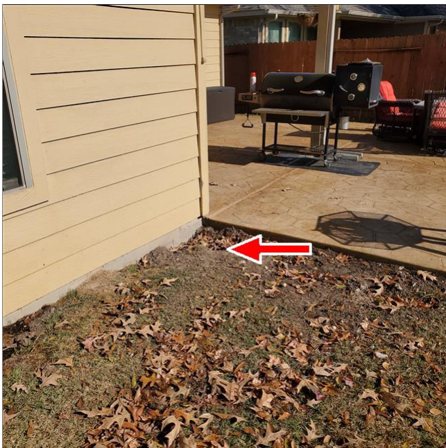
B. Item 1(Picture) Rain water will not be able to drain away from the home here.
