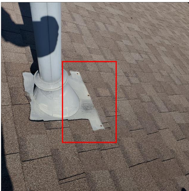
C. Item 6(Picture) Nails need to be sealed at all flashings.
