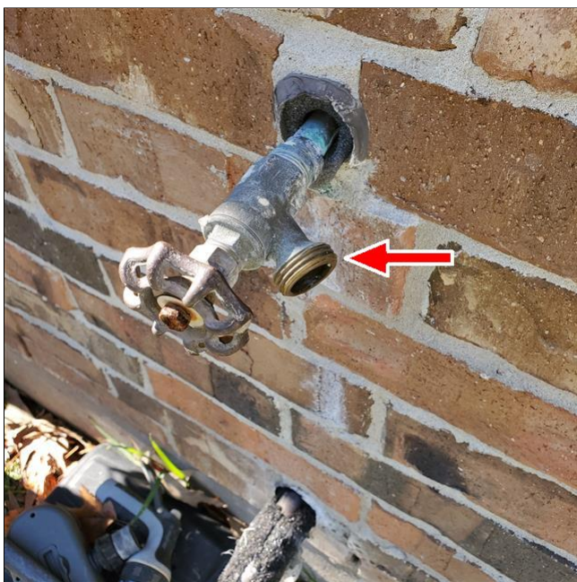
A. Item 2(Picture) No vacuum breaker at this hose bib.
