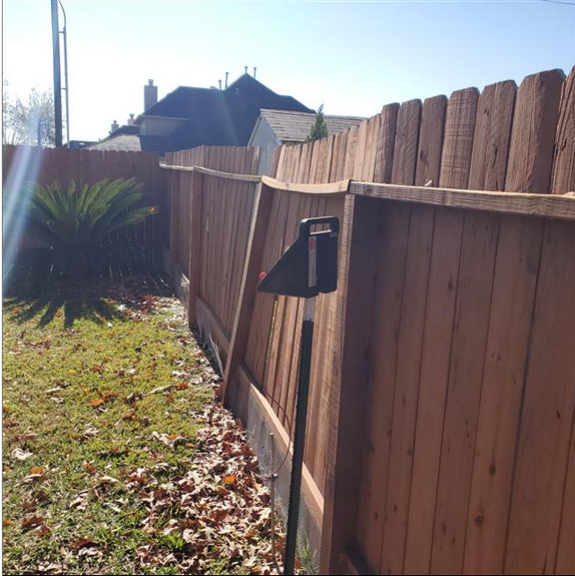
L. Item 1(Picture) Photo of leaning fence.
