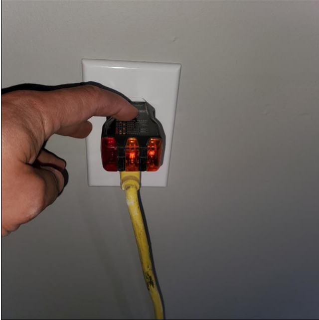
B. Item 3(Picture) Garage outlets did not trip when tested.
