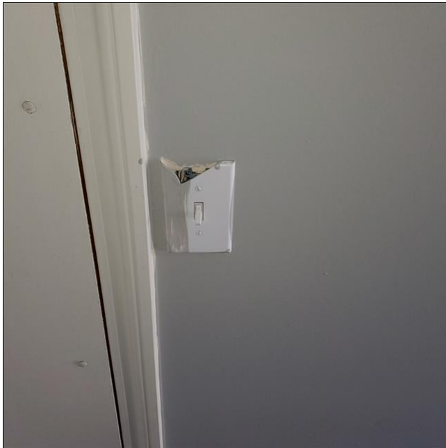
B. Item 1(Picture) Photo of damaged cover plate.
