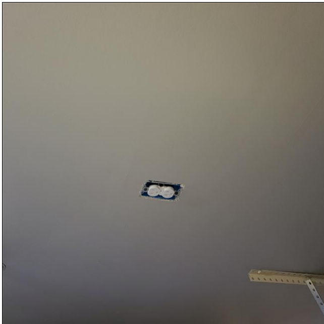
B. Item 2(Picture) Outlet missing a cover plate.
