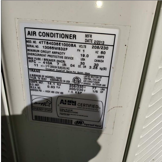
B. Item 1(Picture) AC unit manufactured in 2013
