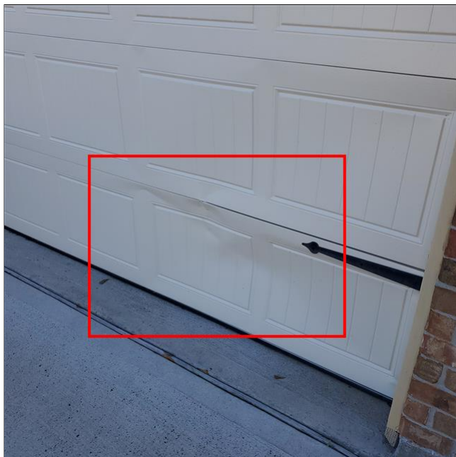
G. Item 2(Picture) Damage to garage door.
