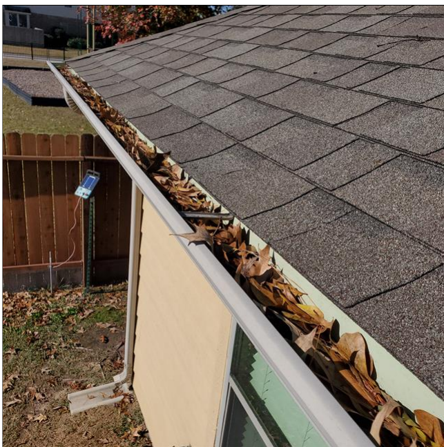
B. Item 2(Picture) Gutters need to be cleaned.
