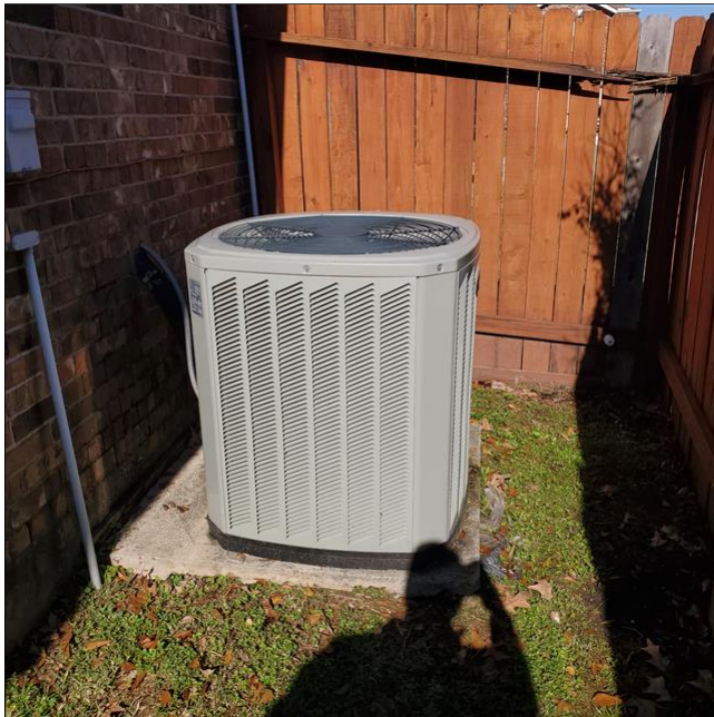
B. Item 2(Picture) Overview of AC unit.
