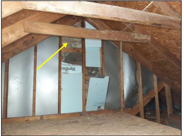
DAMAGED / MISSING MOISTURE BARRIER
