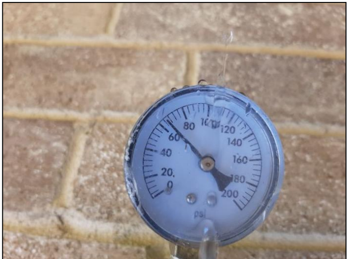
WATER PRESSURE OK
