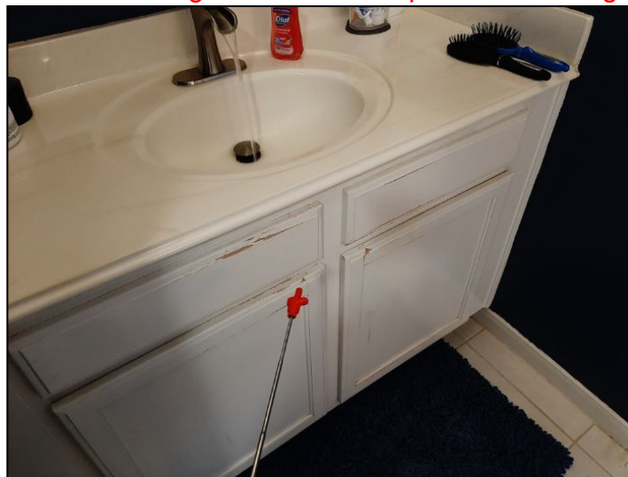
DETERIORATION / PAINT CHIPPING
