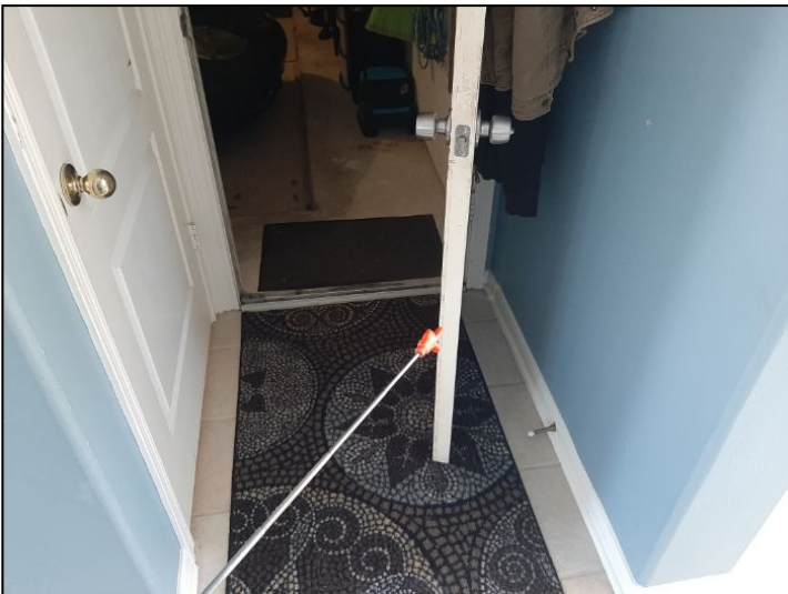
DOOR RUBBING ON FRAME
