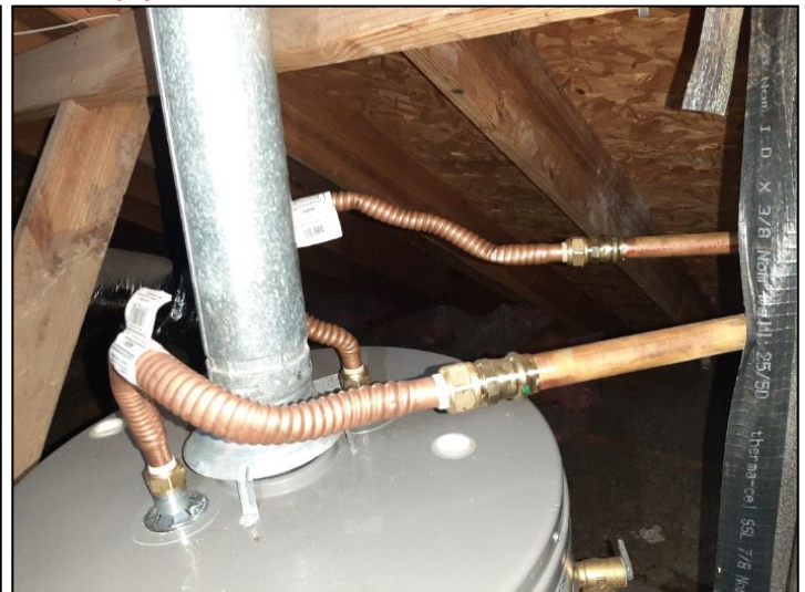
WATER HEATER CONNECTIONS OK
