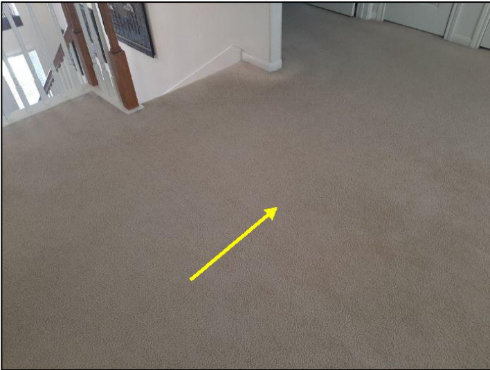
NOISY SUB FLOOR
