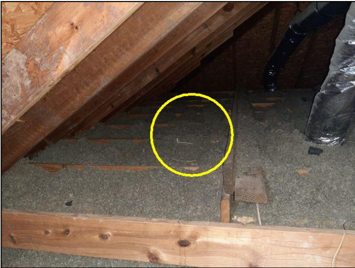
MINIMAL INSULATION PRESENT
