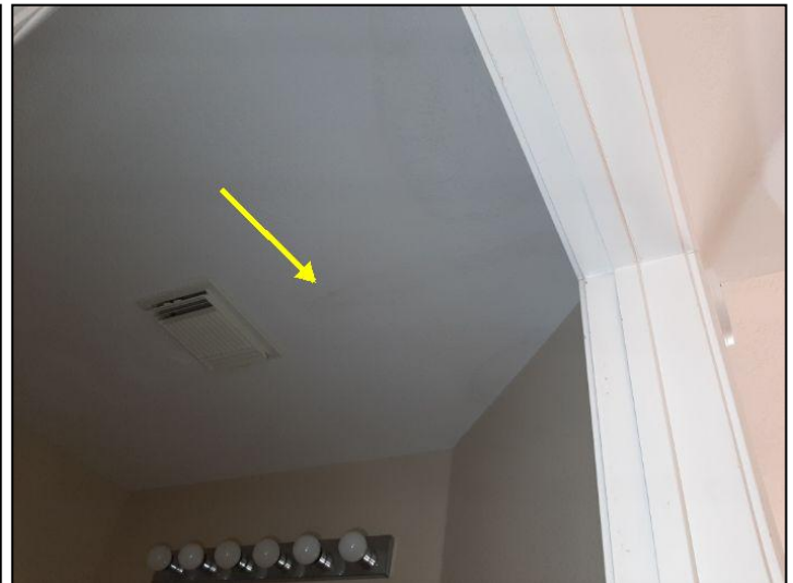
OLD WATER STAIN NEEDS TO BE PAINTED
