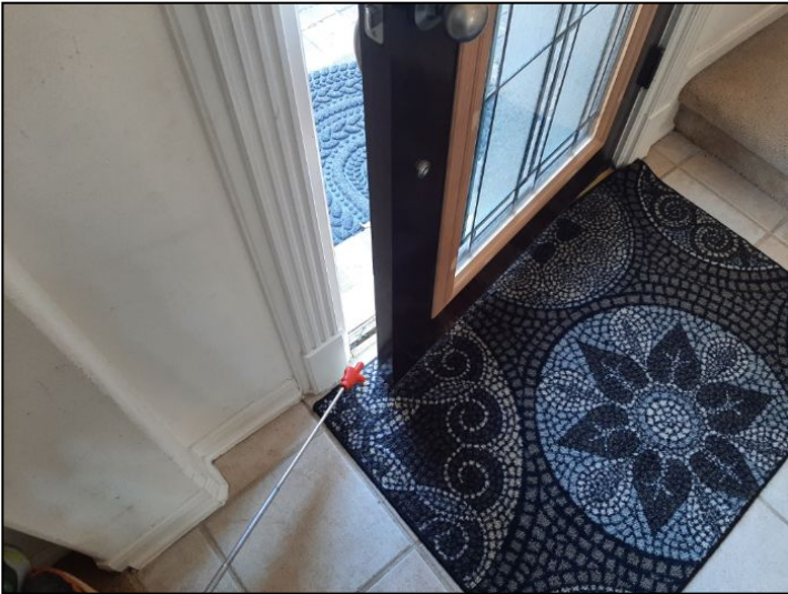
DOOR RUBBING ON FRAME
