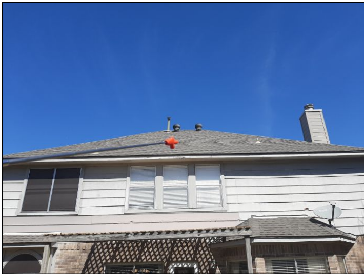
LIFTED SHINGLE / EXPOSED NAILS
