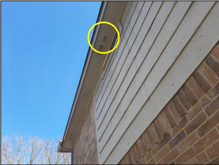
EVAPORATOR SECONDARY DRAIN PIPE ROUTED HERE
