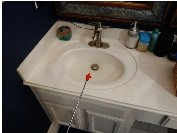
SLOW / CLOGGED DRAIN
