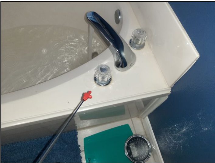
DAMAGED / LEAKING FIXTURE
