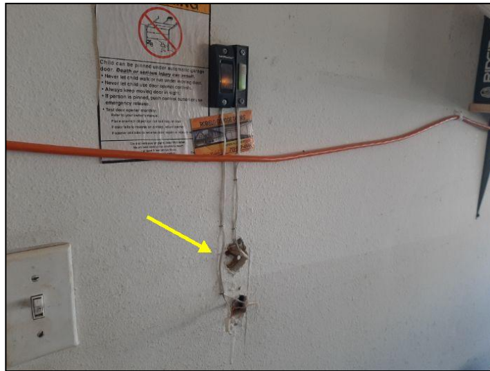
EXPOSED WIRES / DAMAGED WALL SECTION
