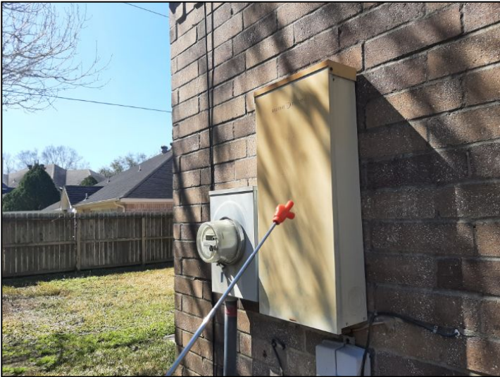
MINIMAL DETERIORATION AT PANEL
