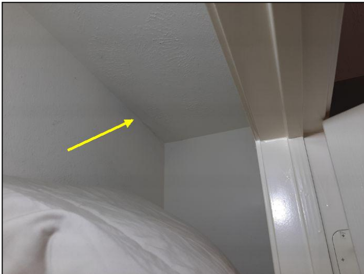
OLD WATER STAIN NEEDS TO BE PAINTED
