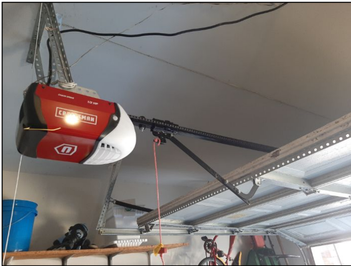
GARAGE DOOR OPENER OK
