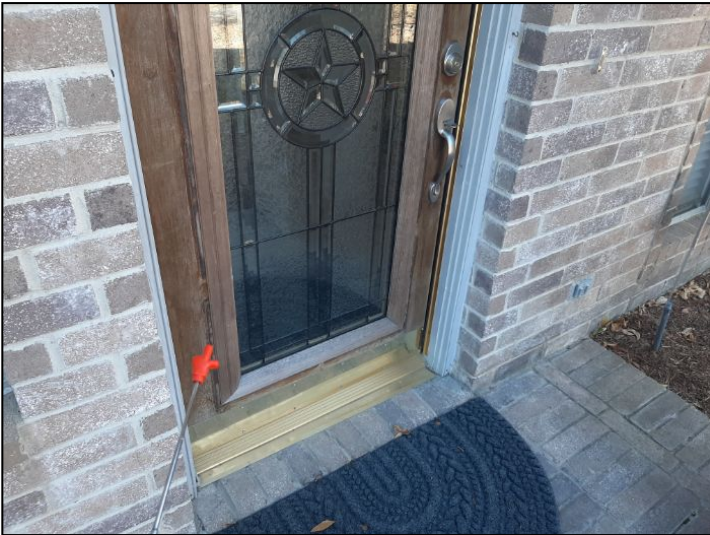
DETERIORATION TO DOOR FINISH
