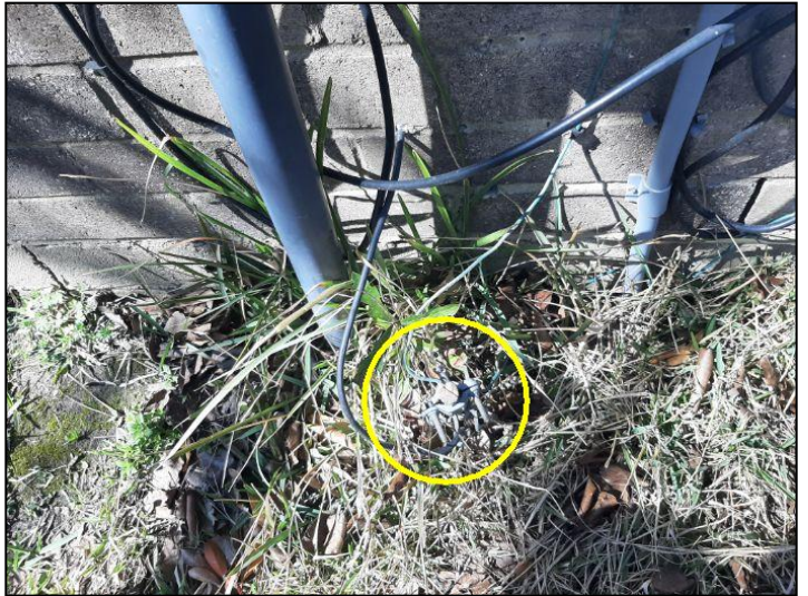
MAIN GROUNDING OK
