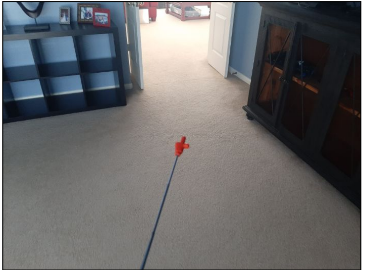
NOISY SUB FLOOR
