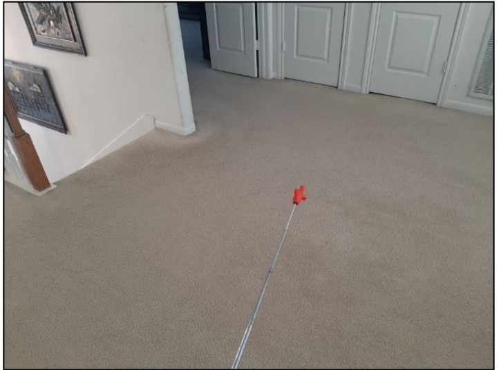
NOISY SUB FLOOR
