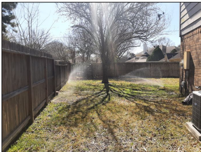
SPRINKLER ZONES OK
