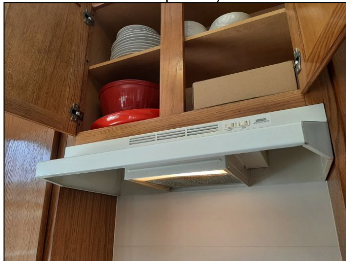
VENT HOOD OK
