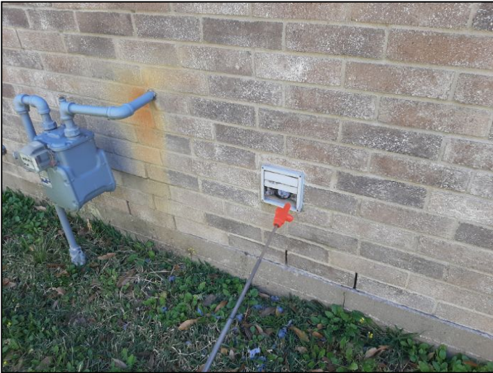
DAMAGED EXTERIOR VENT COVER
