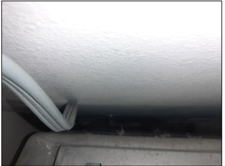
BOTH GAS AND ELECTRIC DRYER CONNECTIONS
