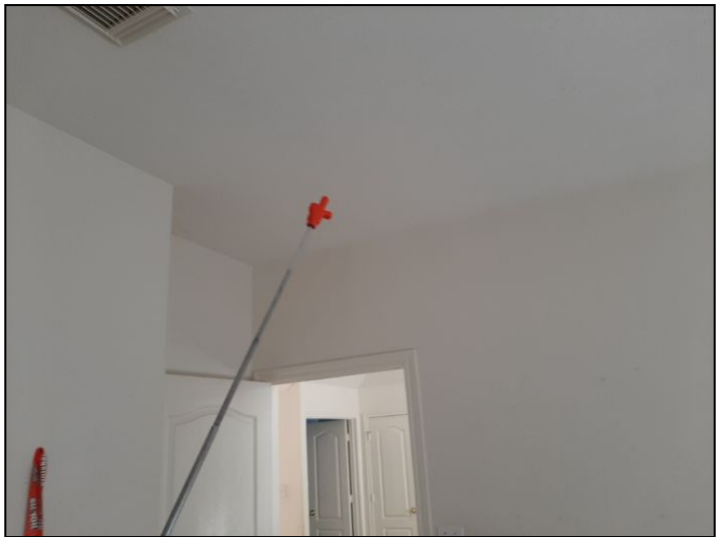
MISSING SMOKE DETECTOR
