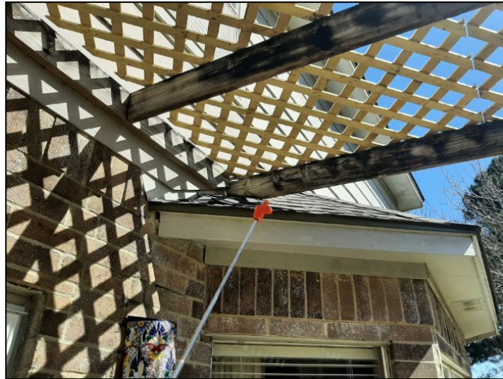
DAMAGED / UNSECURED PORCH COVER SECTION
