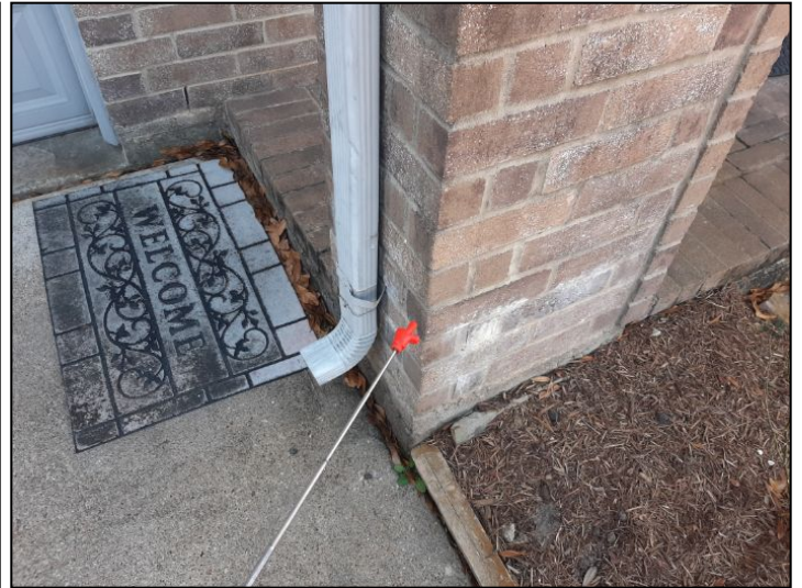
LOOSE GUTTER SECTION
