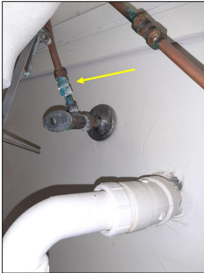
RUST / CORROSION AT CONNECTIONS
