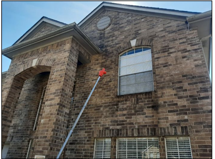
MINOR WALL STAINING DUE TO LEAKING GUTTERS
