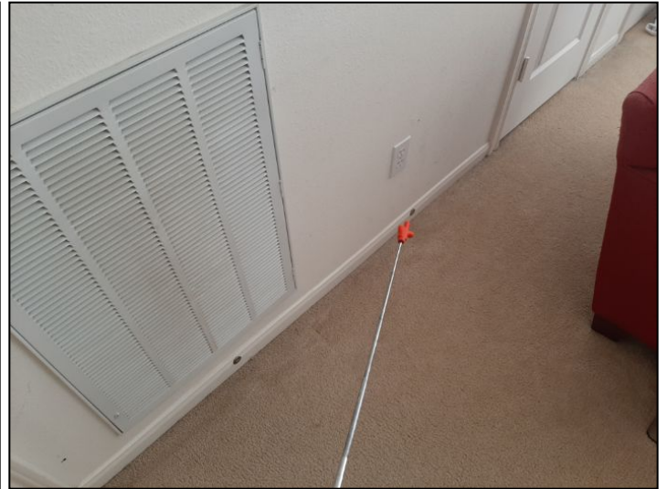
MISSING DOOR STOPPER
