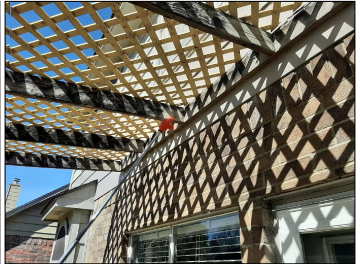
IMPROPERLY SECURED PORCH COVER
