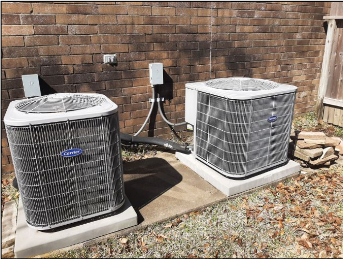
CONDENSING UNIT OK
