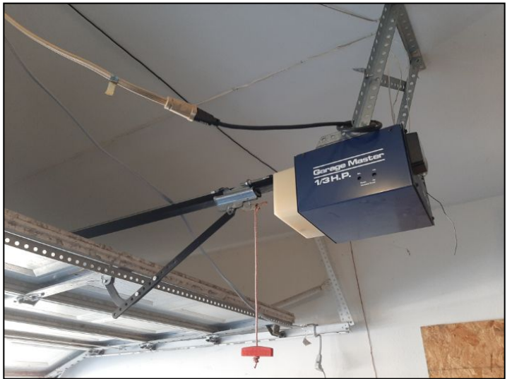
GARAGE DOOR OPENER OK
