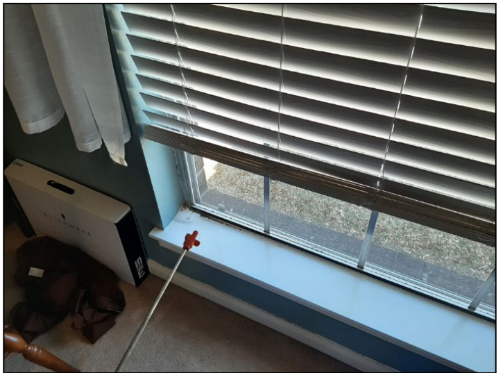
DAMAGED WINDOW SILL
