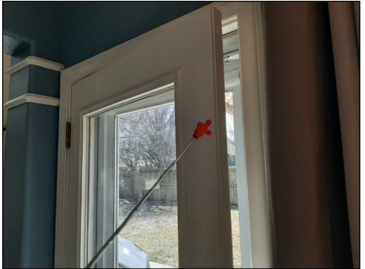
DOOR RUBBING ON FRAME
