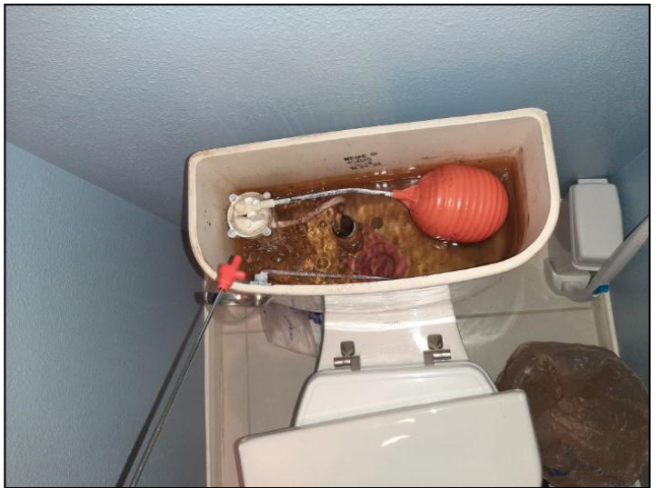
DAMAGED / LEAKING FLUSH VALVE
