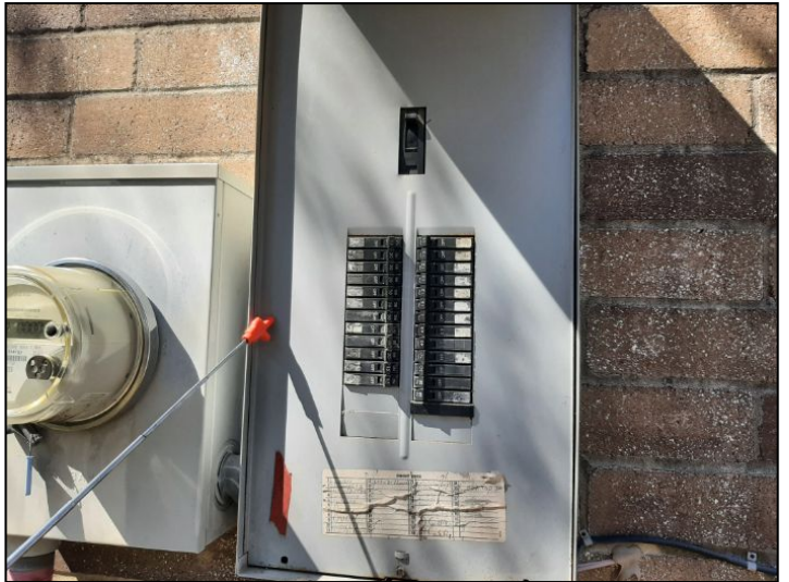
MISSING ARC FAULT BREAKERS
