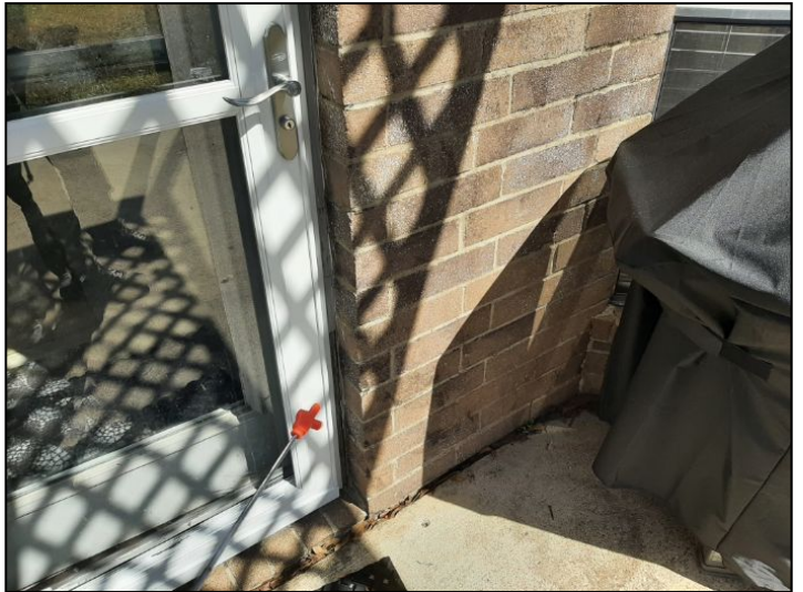
DOOR RUBBING ON FRAME
