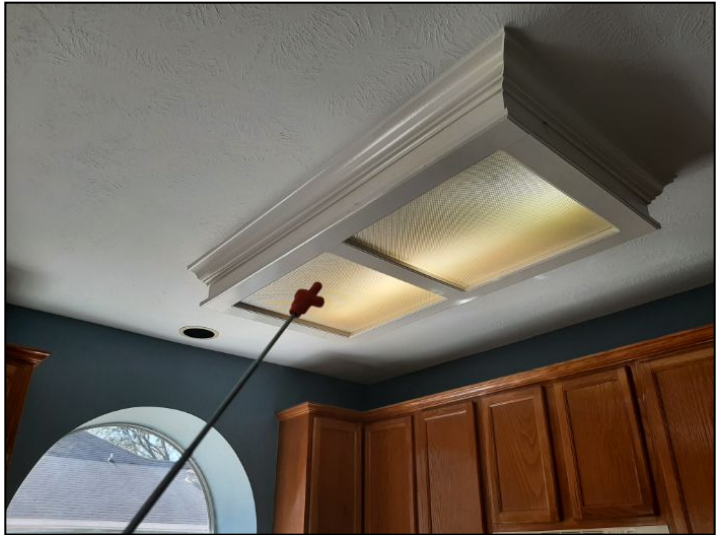
DAMAGED / INOPERABLE LIGHT FIXTURE
