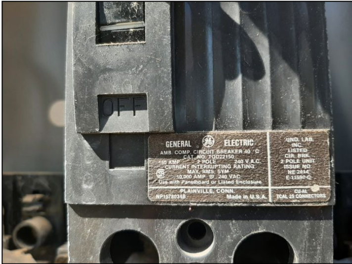
MAIN BREAKER OK
