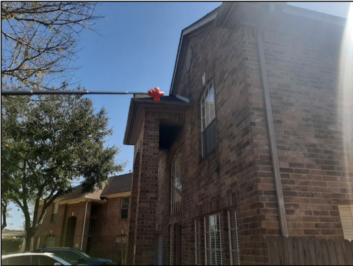
OPENING TO ATTIC AREA DUE TO VERMIN ACTIVITY
