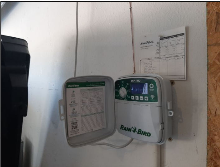
SPRINKLER CONTROL OPERATIONAL
