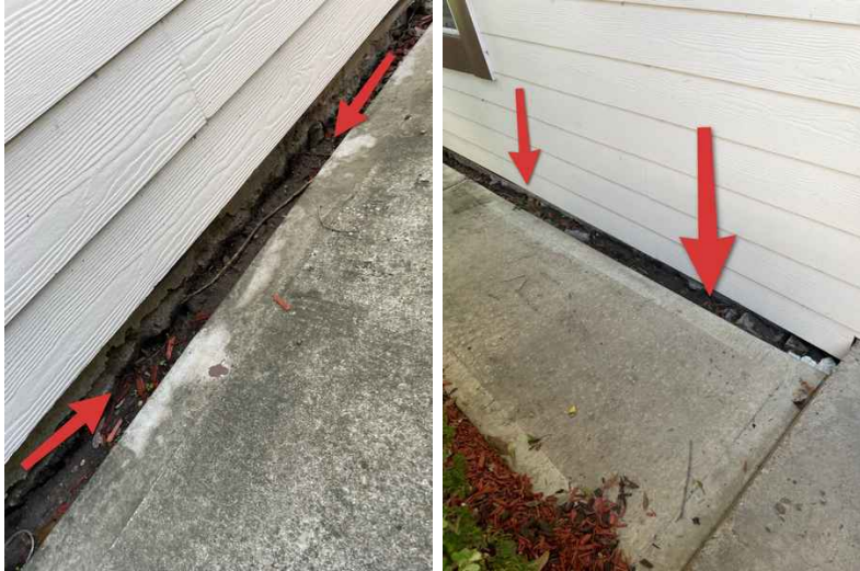
Water is getting stuck along front right elevation. Water should travel away from home.
