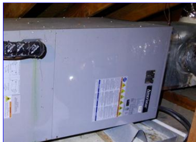
Attic WH unit
