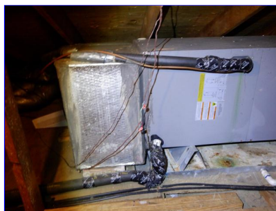
Attic evaporator unit,2013,9yrs old
