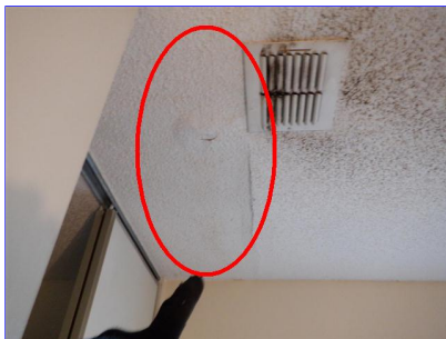
Upstairs bedroom ceiling
