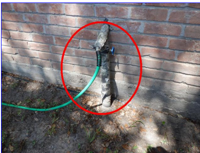
Left siding main water shut off valve
