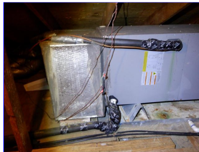
Attic evaporator unit,2013,9yrs old
