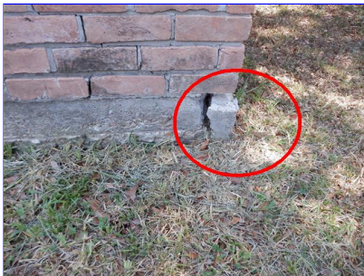
Rear foundation corner crack
