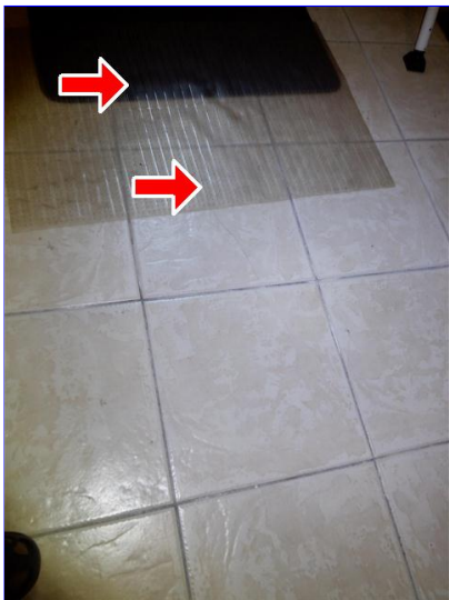
Front entrance tile crack
