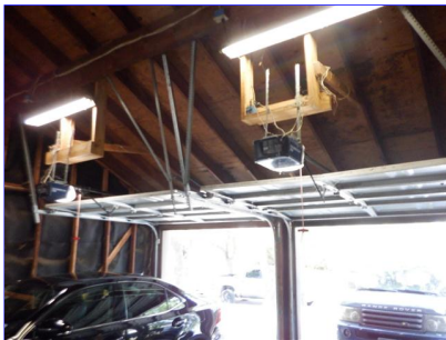
Garage two doors auto
