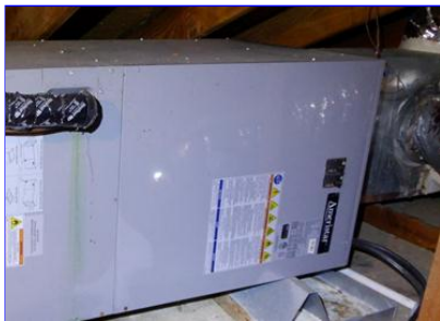
Attic WH unit
