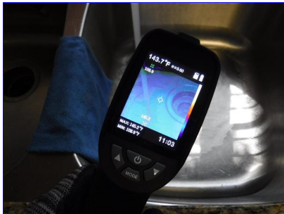
Hot water temperature Kitchen @143F
