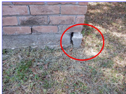
Rear foundation corner crack
