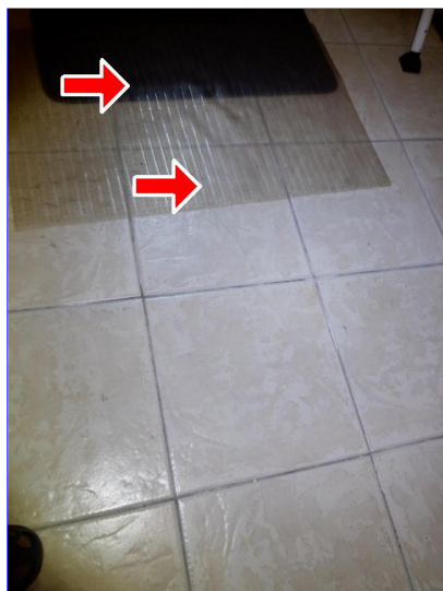
Front entrance tile crack
