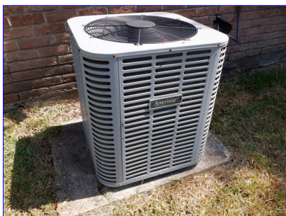
Outside AC unit
