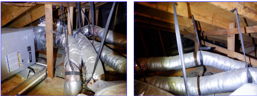
Attic registry & return duct lines
