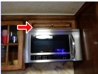
Kitchen exhaust vented NOT to exterior
