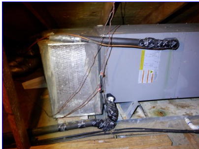
Attic evaporator unit
