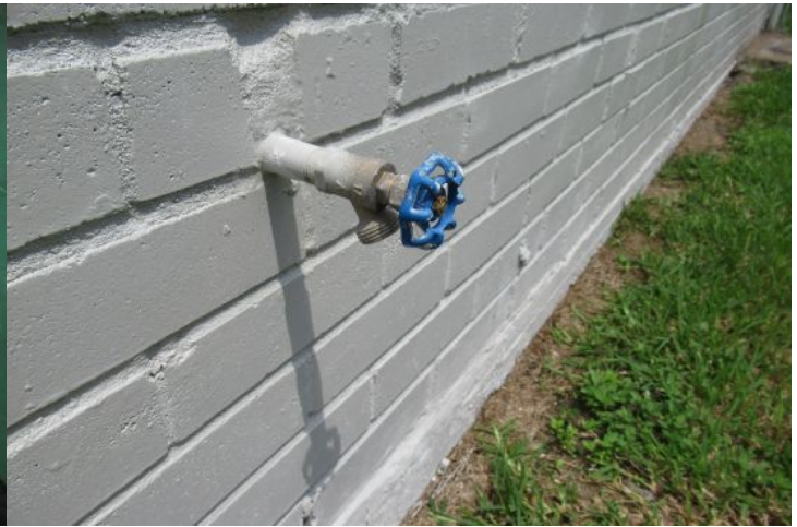
back flow preventers were missing
