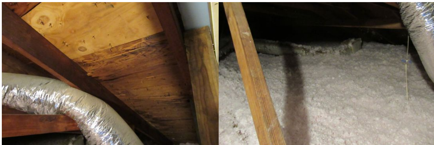
roof sheathing shows damage
