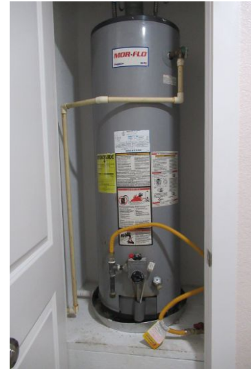
Unit is old, recommend replacement
