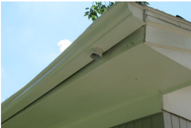
down spout missing
