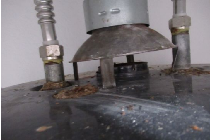
rust on top of unit
