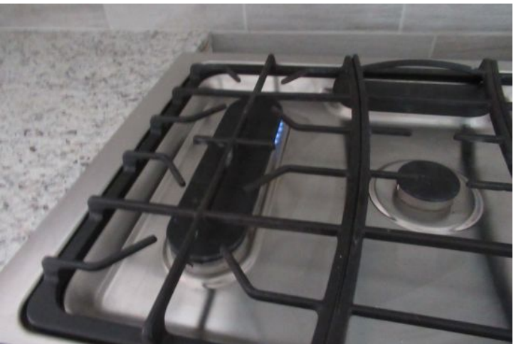
The burners: not all flames came on
