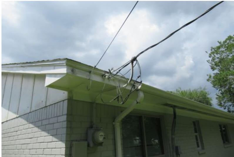
electric service line to close to the ground
