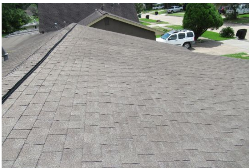
wave in the roof
