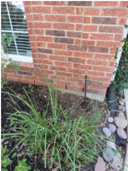
1. Soil Level / Spalling Crack
