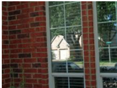
Window cracked front
