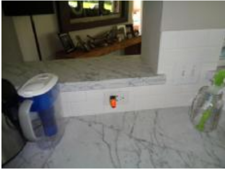
GFCI missing kitchen
