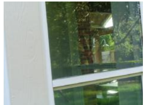
Window cracked right
