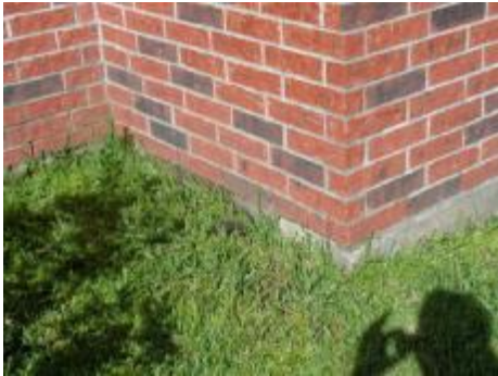
Popped corner left front
