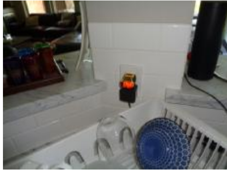
GFCI missing kitchen
