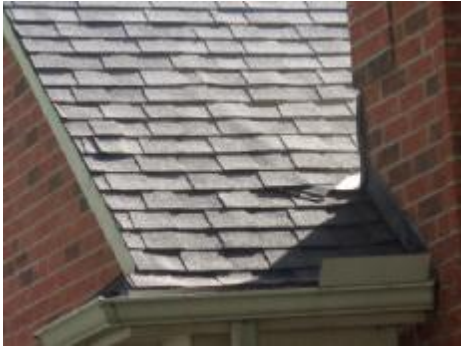
Roof shingle damage front garage
