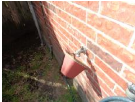
Backflow missing left
