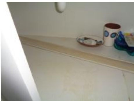
Leak under bathroom sink
