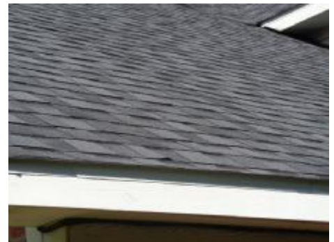
Roof raised shingle left
