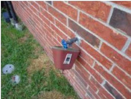
Backflow missing right
