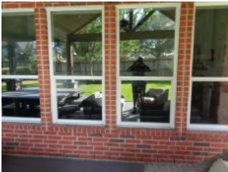
Windows missing screens
