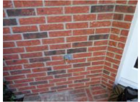
GFCI missing exterior front door
