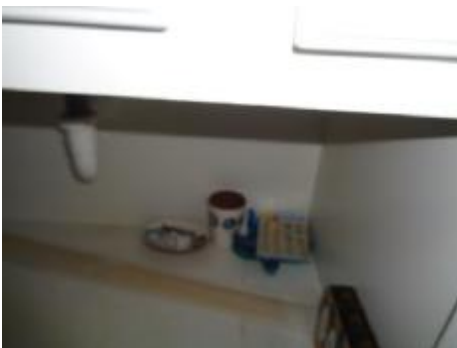
Leak under bathroom sink
