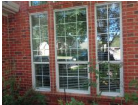
Windows missing screens
