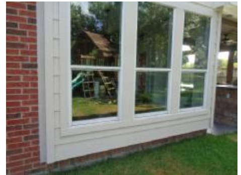
Windows missing screens
