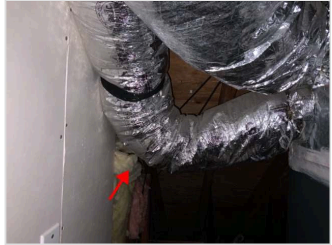
Upstairs heating unit
