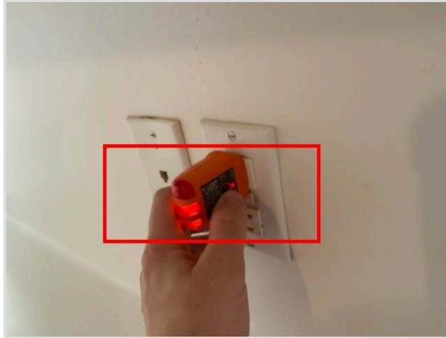
Kitchen electrical receptacle
