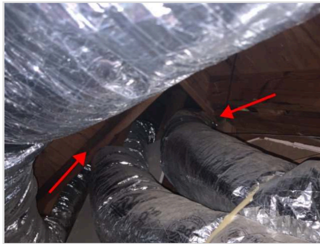
Upstairs heating unit
