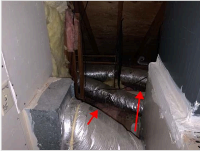
Attic space duct work
