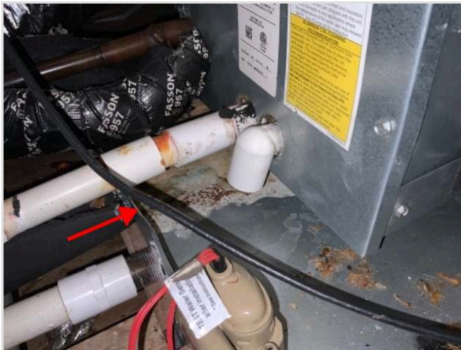
Downstairs heating unit
