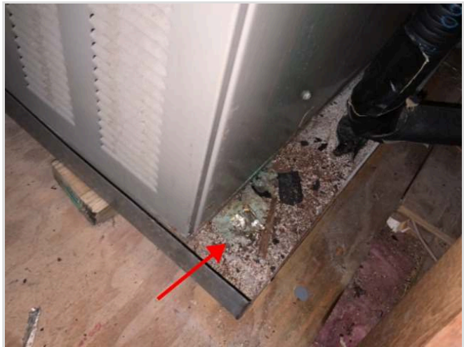
Upstairs heating unit
