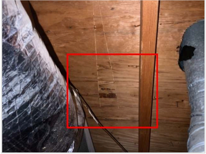
Above upstairs heating unit
