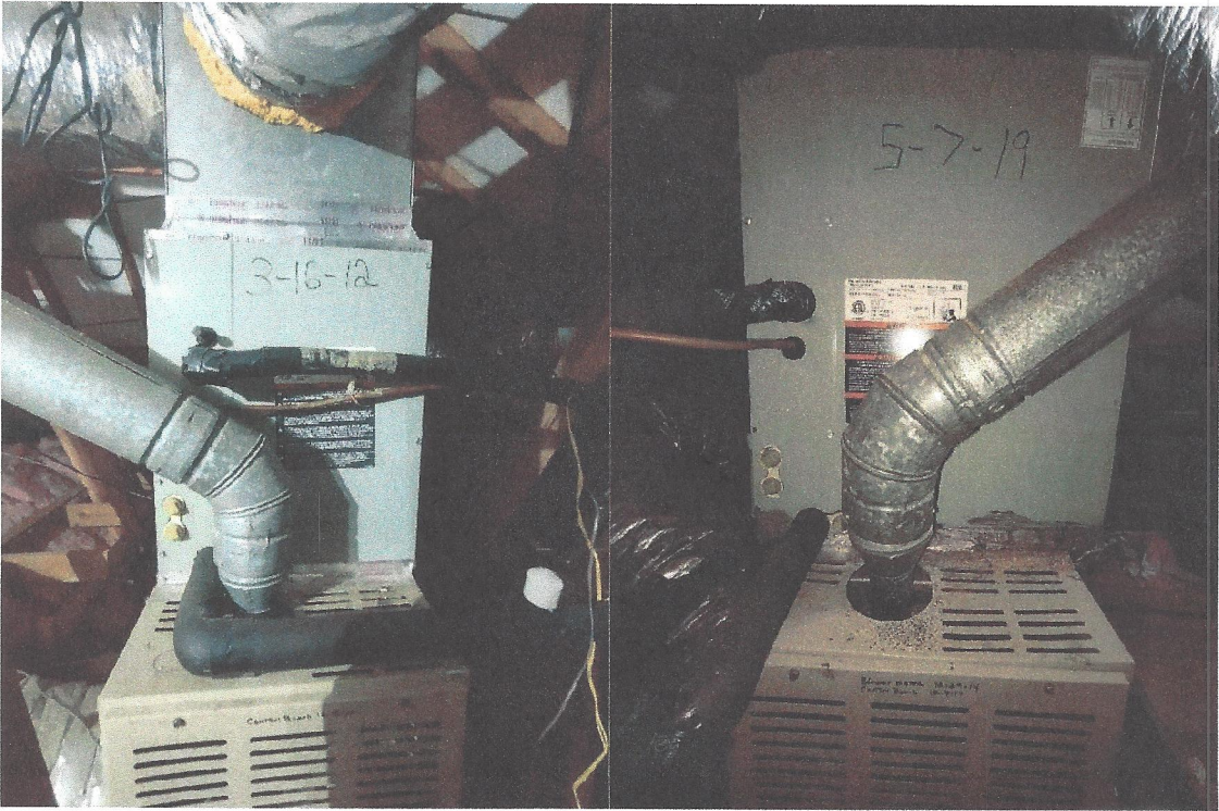
➤ Upgraded HVAC systems (both units)
