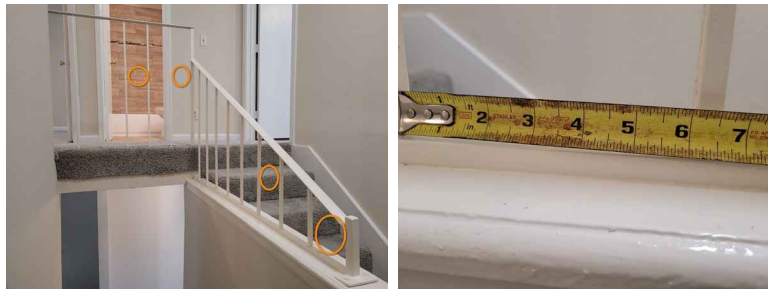
The baluster gap
