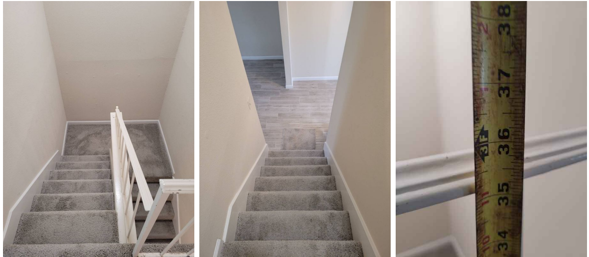
Proper guard rail height
