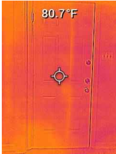
Some conditioned air loss from the back door
