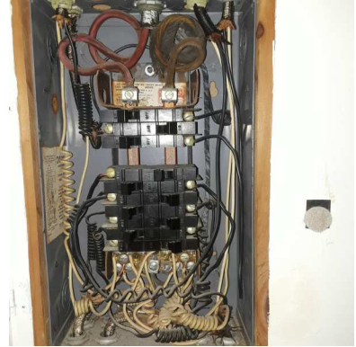
Sub panel in the hallway.
