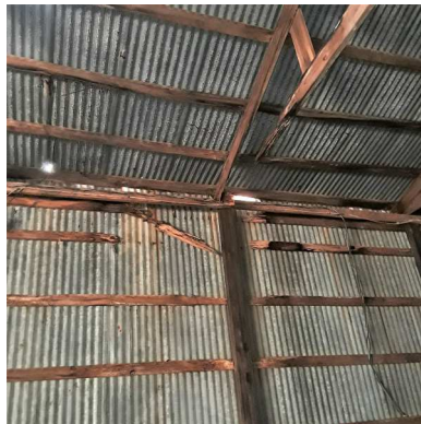
Water damage in large barn.
