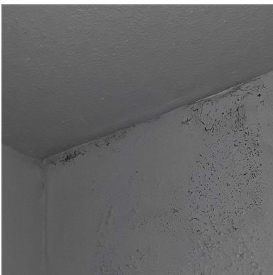
Mildew in bathroom wall.
