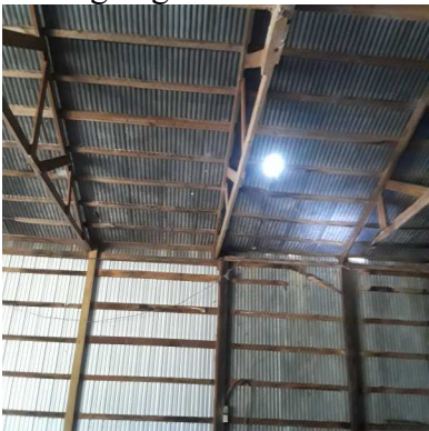
Holes in large barn roof.
