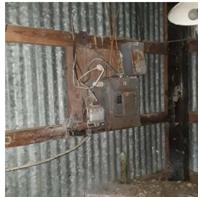
Large barn service panel.
