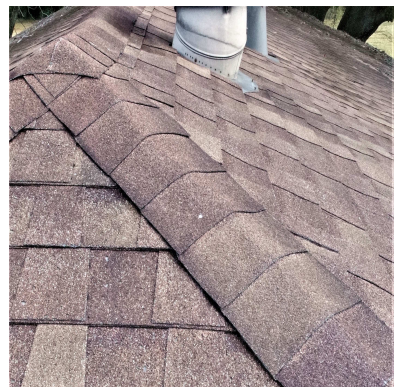
Little gravel loss, no spider cracking.
