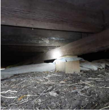
Grass debris under the home.
