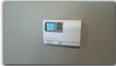
The Thermostat/s is located in the master bedroom.
