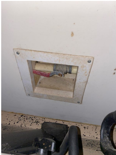
General Photos of Water Heating Equipment:
