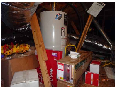
General Infrared Photos of Water Heating Equipment:
