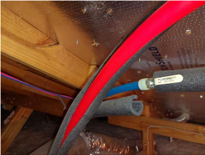
Picture of water supply lines - PEX
