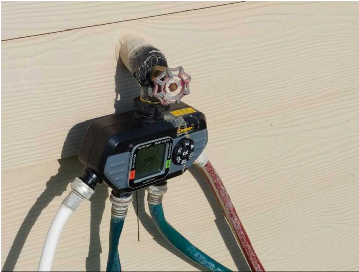
Unable to connect pressure gauge
