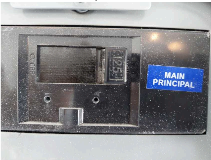
Main breaker (125 A)
