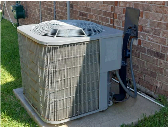
AC condensing unit
