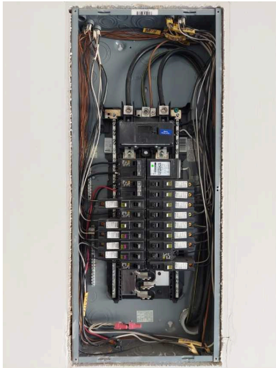
Picture with deadfront panel removed
