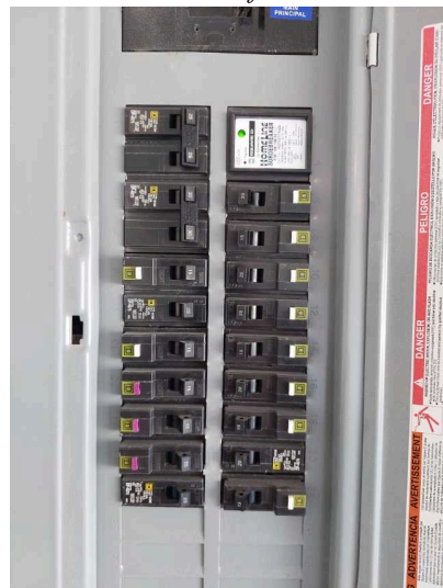
Picture of breakers
