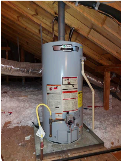
Picture of water heater
