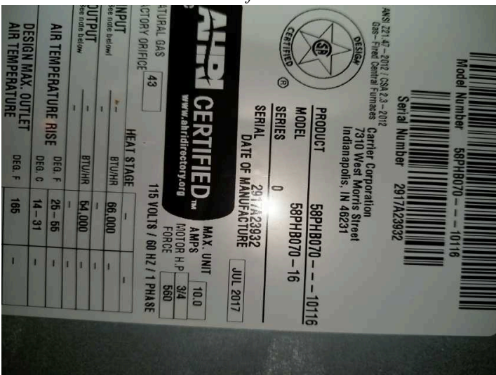
Furnace Data Tag (2017)
