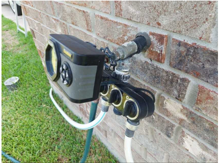
Unable to connect pressure gauge
