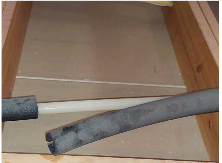
Picture of water supply lines - PEX
