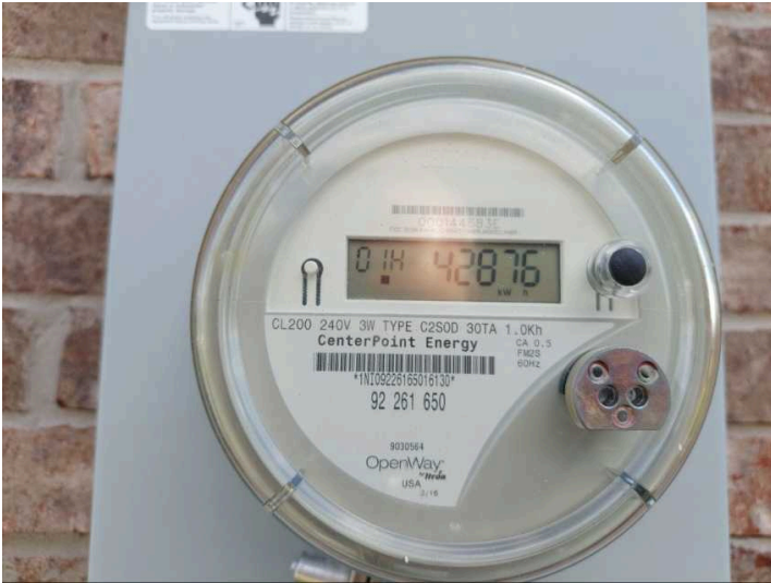
Picture of electric meter
