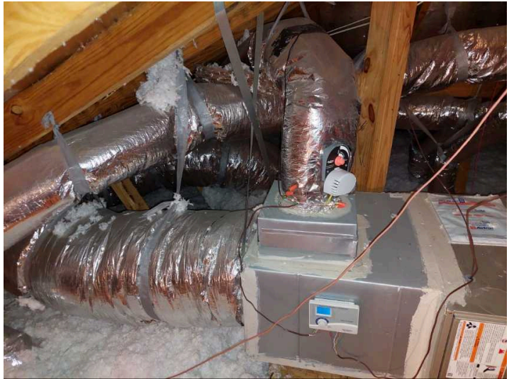
Picture of ducts in attic
