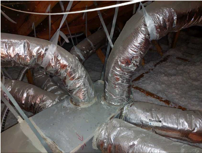
Picture of ducts in attic
