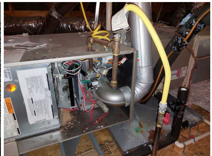
Gas furnace with cover removed
