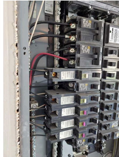
Branch conductor connections to breakers
