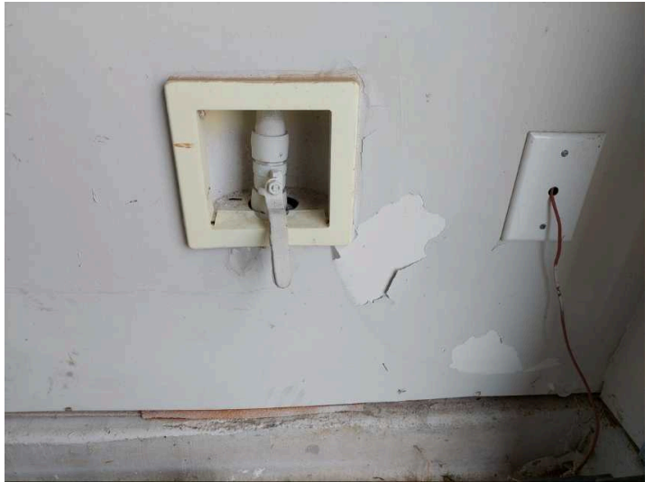
Main water shutoff valve
