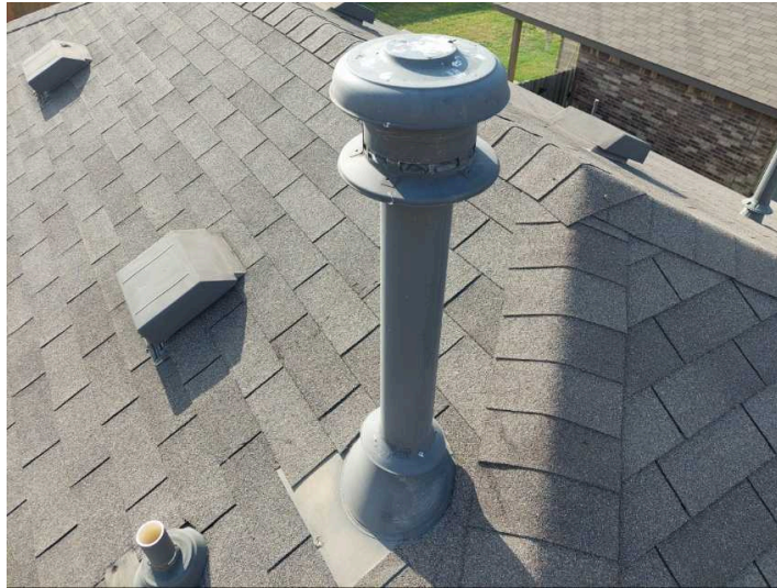
Gas furnace exhaust vent
