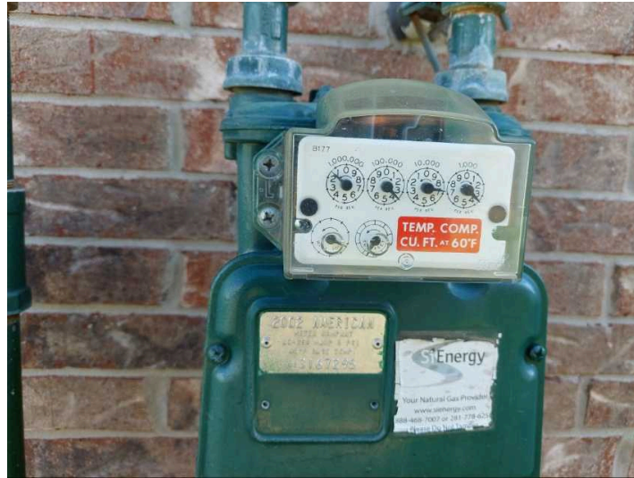
Picture of Gas Meter
