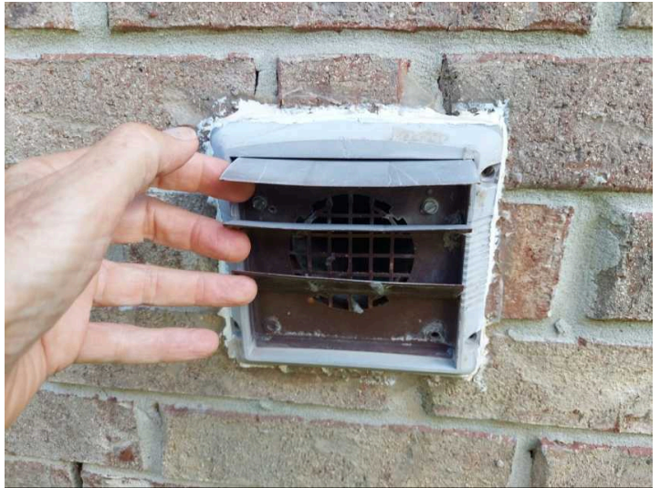
Dryer vent cover with screen
